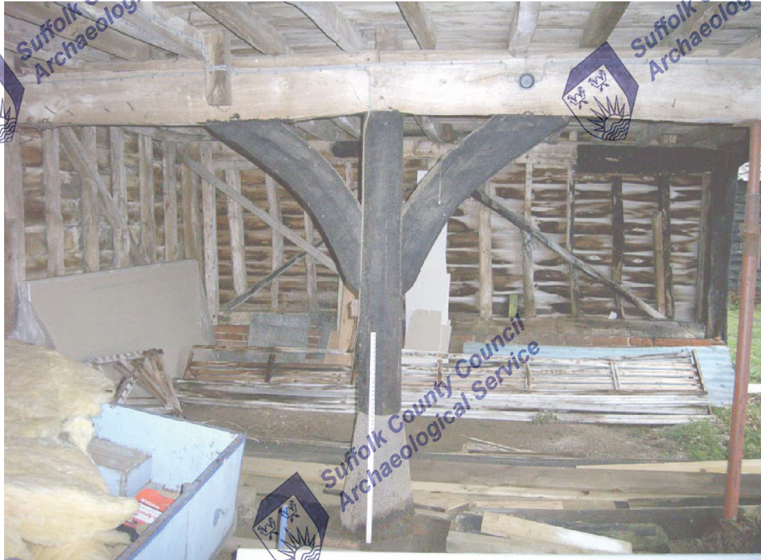
A2.9 Cartlodge (4). Interior from west showing the one of the two unusual octagonal Sampson posts with arch-braces to the binding joists and conical iron bases
