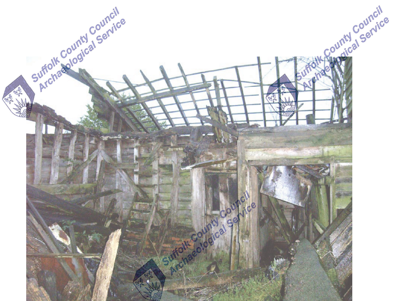
A2.7 Interior of stable (2) showing eastern elevation with door to collapsed shed (2a) to right
