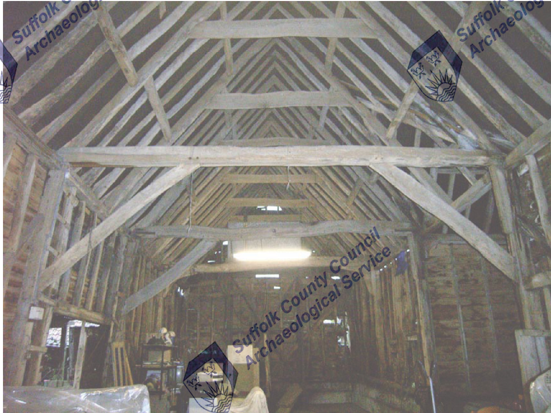
A2.3 Barn (1) Roof structure from south showing original arch-braces flanking central bay
