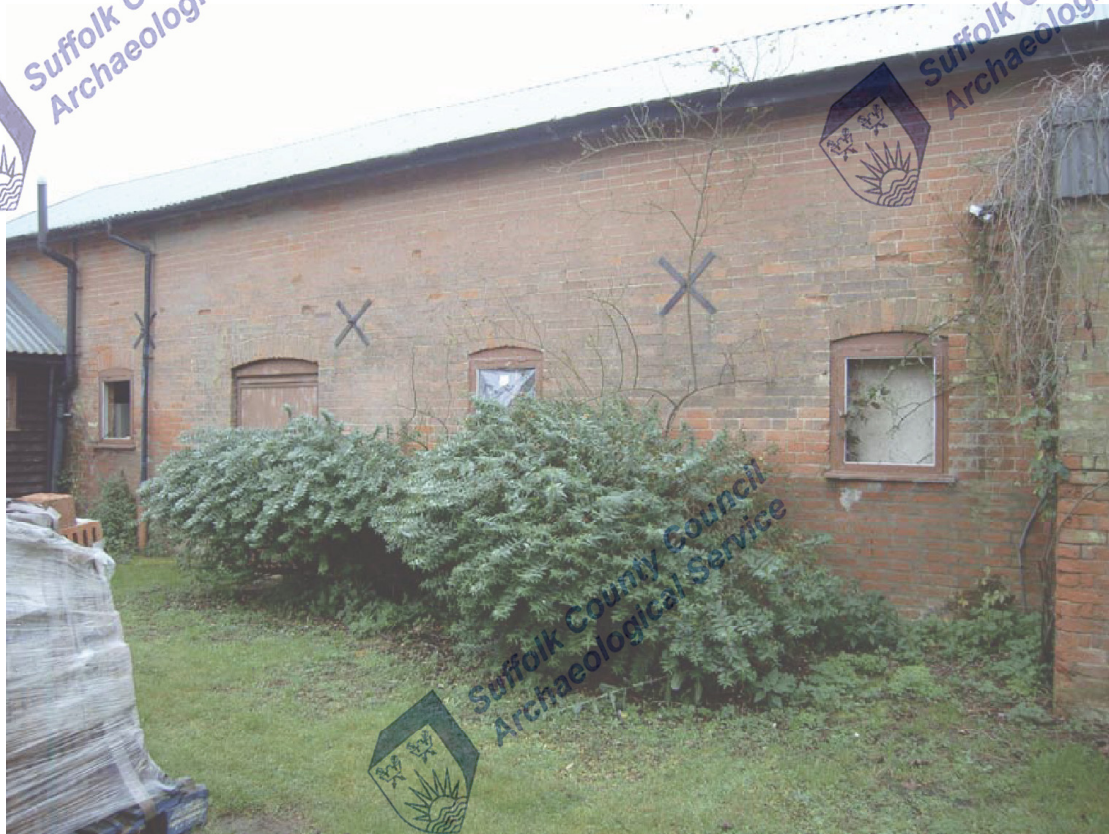
A2.7 Northern facade of stable (1) showing entrance door to left & tack room window right
