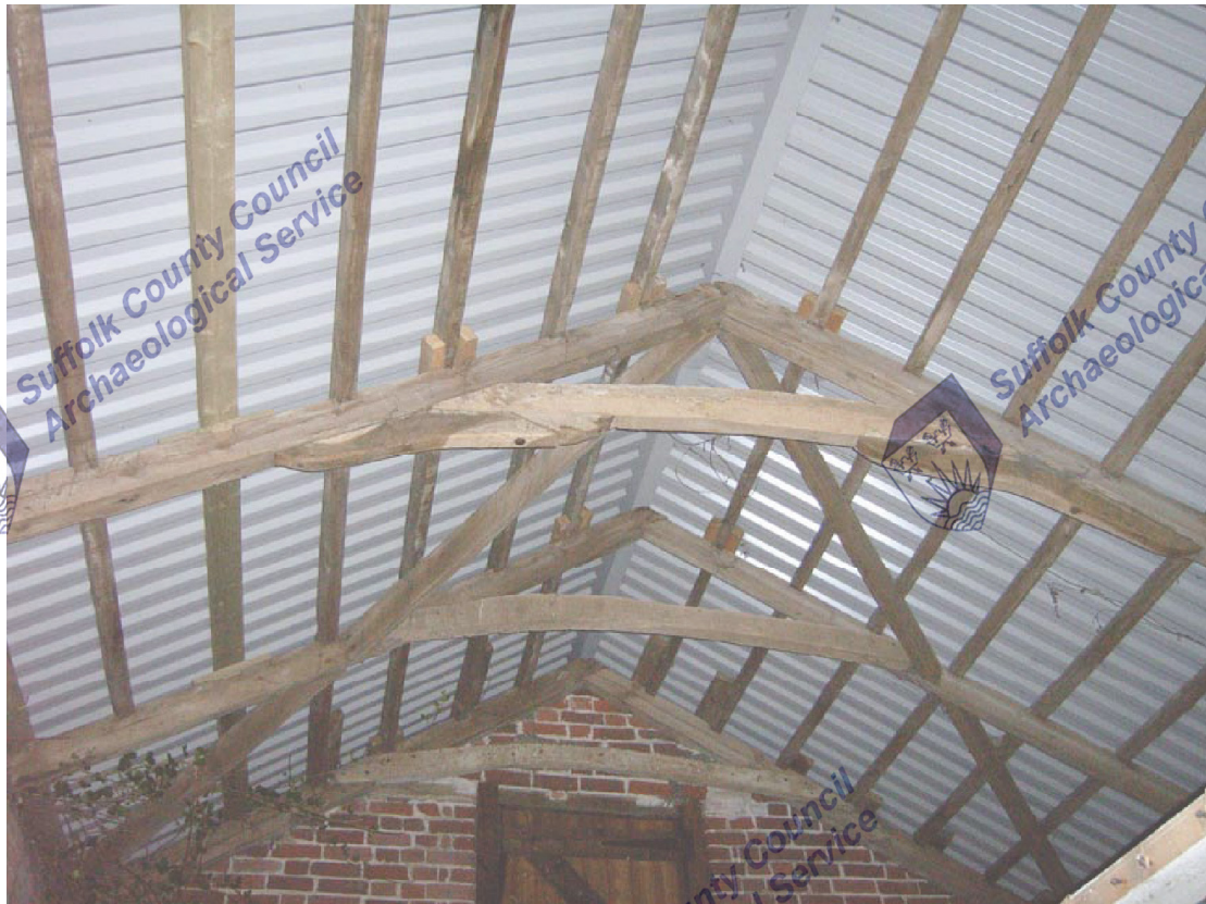
A2.10 Stable (1). Detail of roof structure showing loading door in western gable
