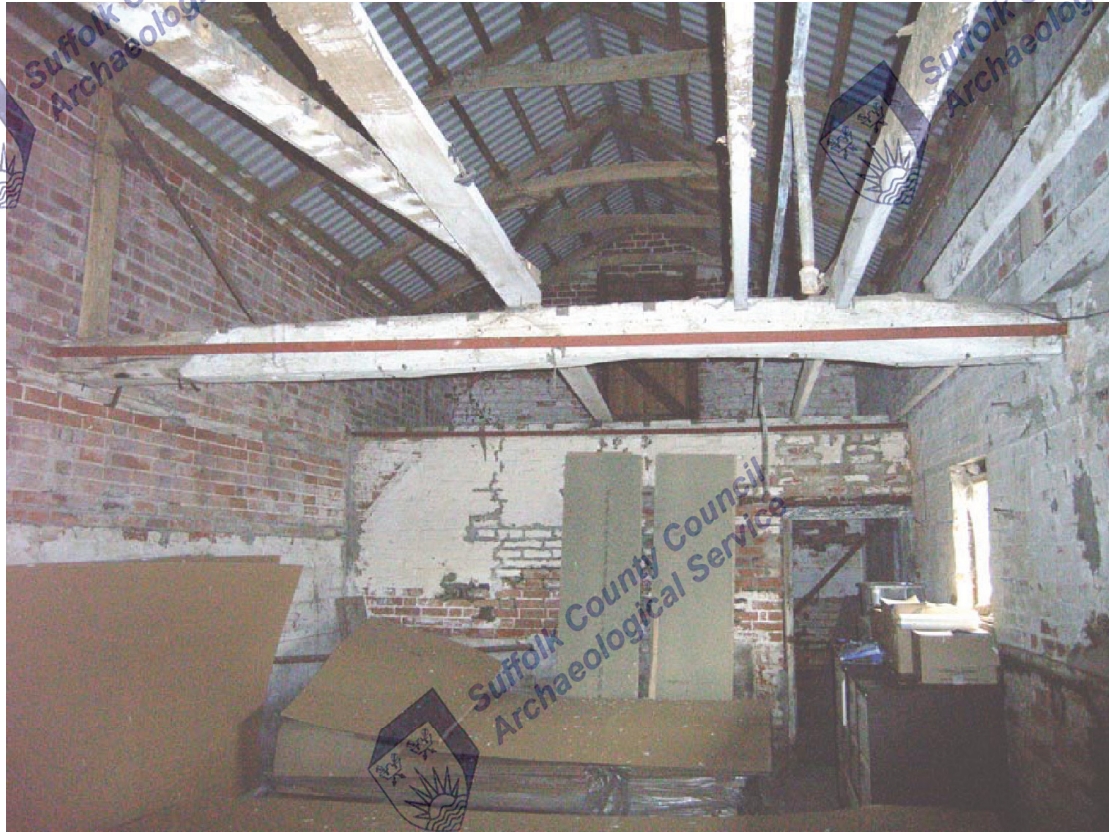
A2.9 Interior of stable (1). General view from east showing entrance to tack room against western gable to left and scar of former hay rack to left
