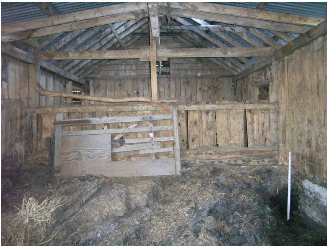
A2.8 Interior of southern loose boxes (4) from south, showing depth of cattle manure
