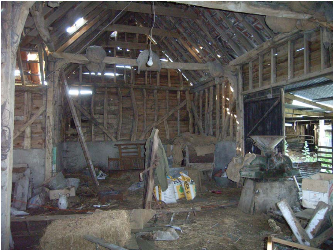
A2.4 Barn (1). General view of interior from southern gable showing entrance from eastern yard to right and porch to left
