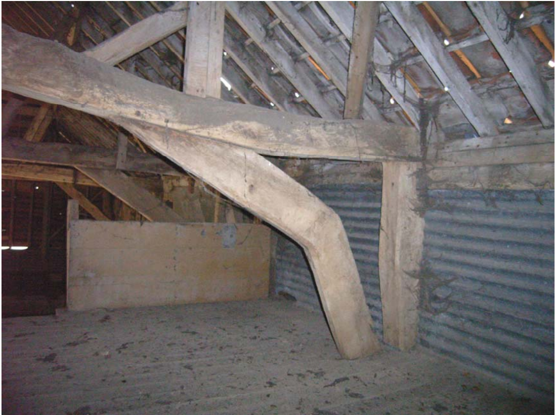
A2.5 Barn (1). Eastern elevation from south showing original cranked arch-brace and tie-beam above granary floor
