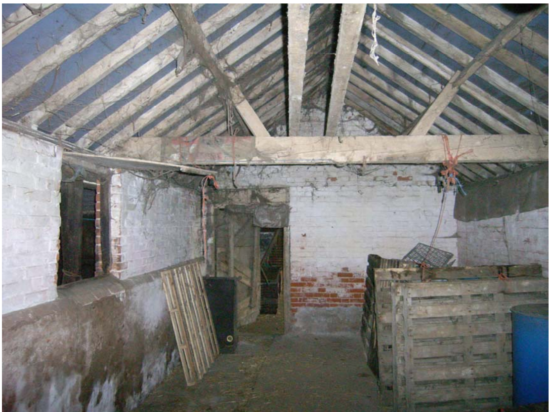
A2.8 Stable (3). Interior from west showing gable door and window to yard (8) left
