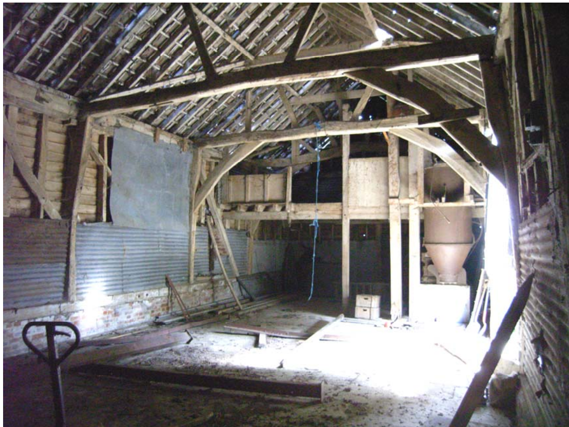
A2.4 Barn (1). General view of interior from north showing largely intact 5-bay late-16 th century timber frame beneath 19 th century roof, with blocked original eastern entrance to left and 20 th century granary and milling floor to south
