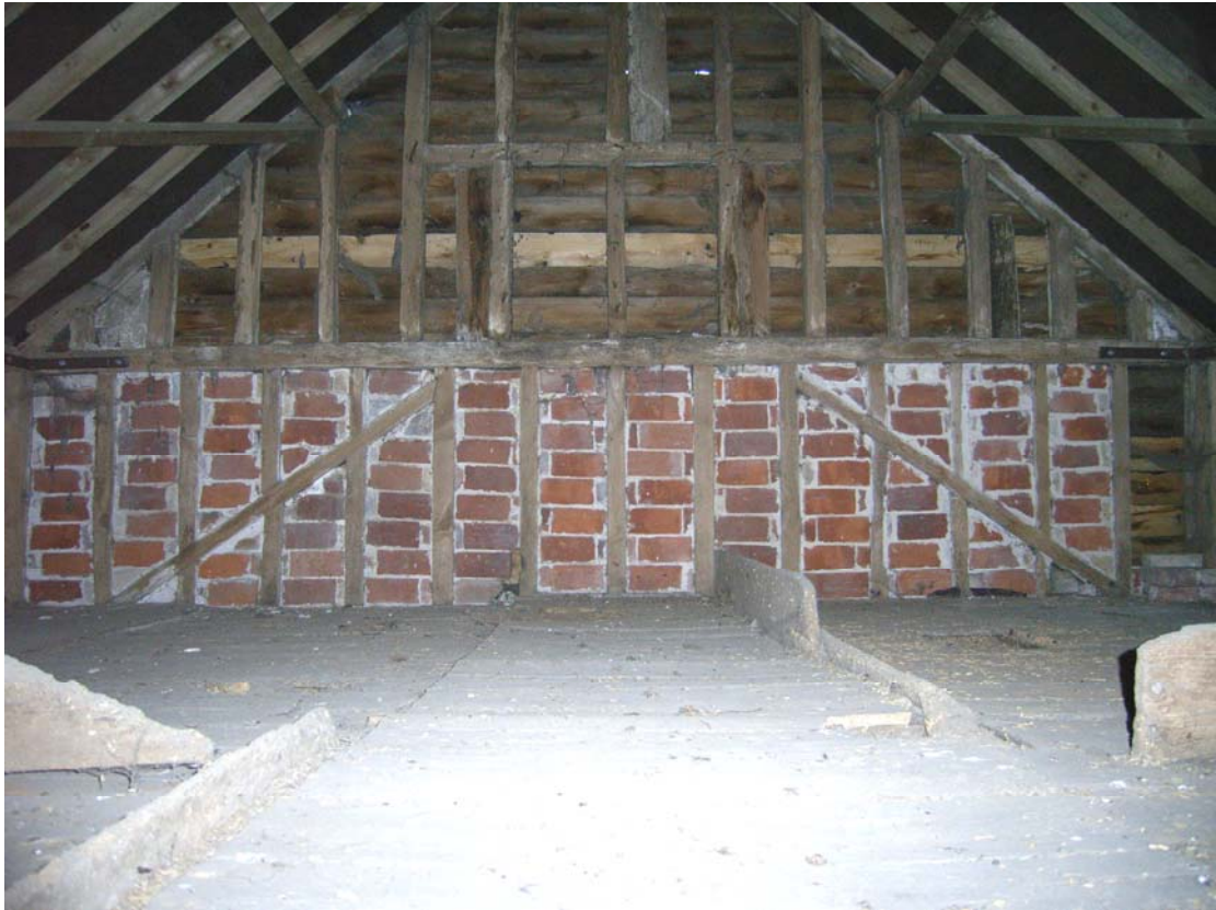
A2.7 Granary (4). Interior of granary floor showing blocked window in northern gable and remains of boarded grain bins with central passage from external entrance in southern gable
