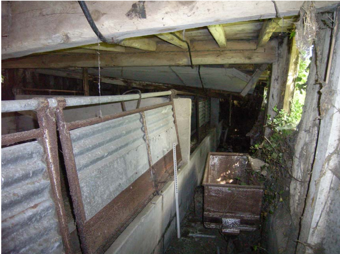
A2.5 Interior of southern range looking east on ground floor from western bay 1 with southern elevation to right and 20 th century pig sties to left. Note intact original ceiling
