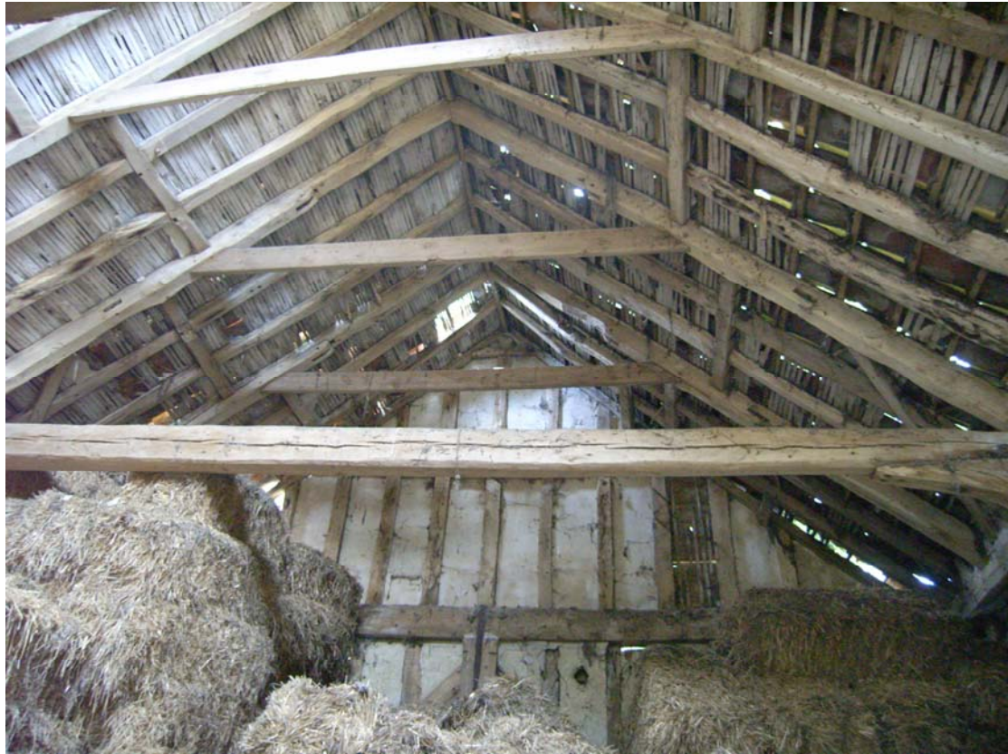
A2.9 Internal elevation of western gable showing re-used timbers in original staggered butt-purlin roof structure
