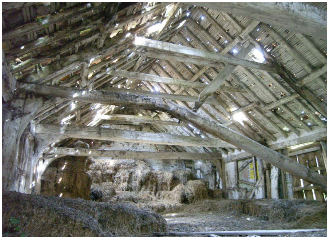
A2.10 Roof structure of clasped-purlins with nailed butt-purlins in eastern half of southern range (looking towards eastern gable). Note first-floor loading door in bay 10 to right
