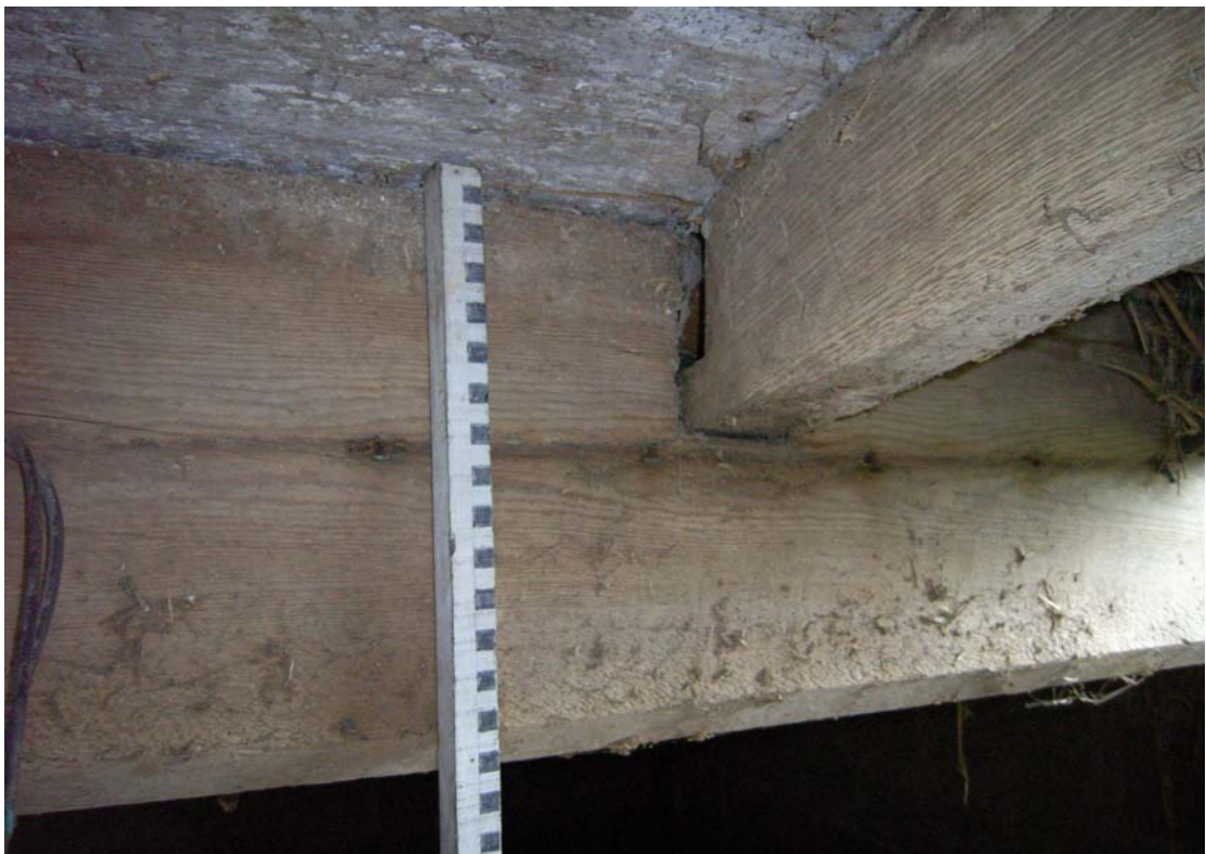
A2.6 Detail of original deal binding joist with oak common joists secured by soffit-tenon joints with diminished haunches. The common joists bear incised carpenters' numerals
