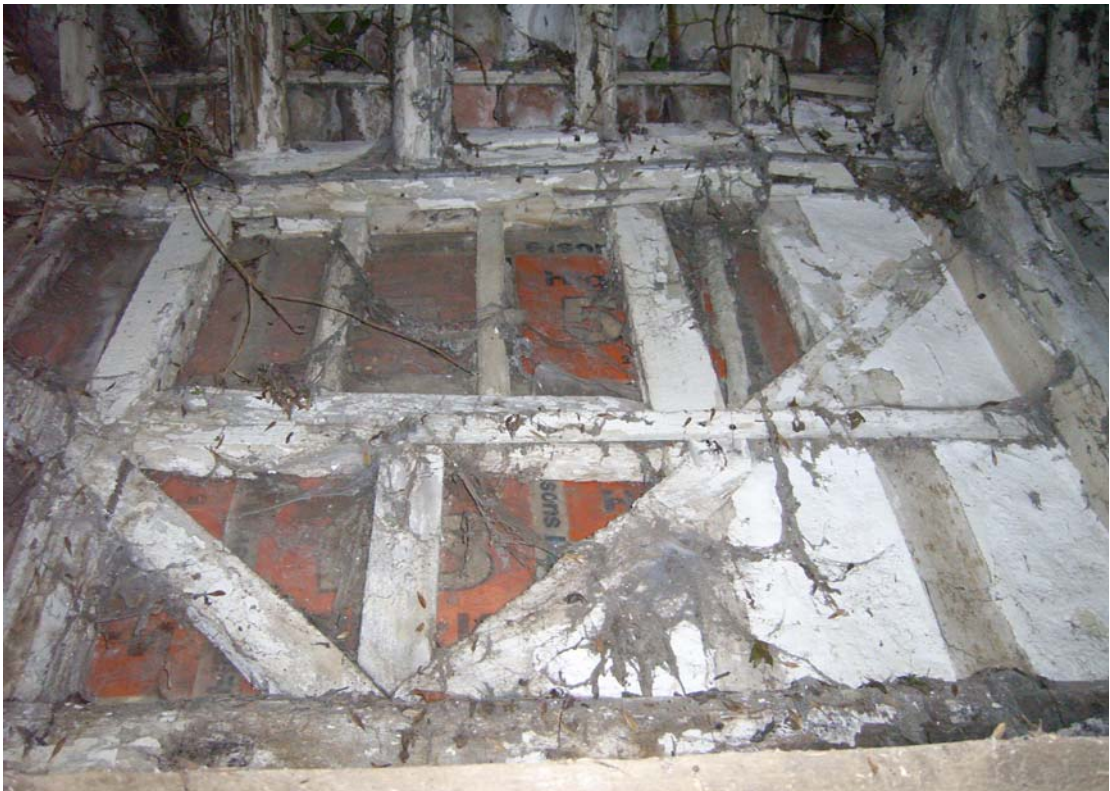
A2.12 Detail of original first-floor window mullions & shutter rails in northern elevation of bay 8.
