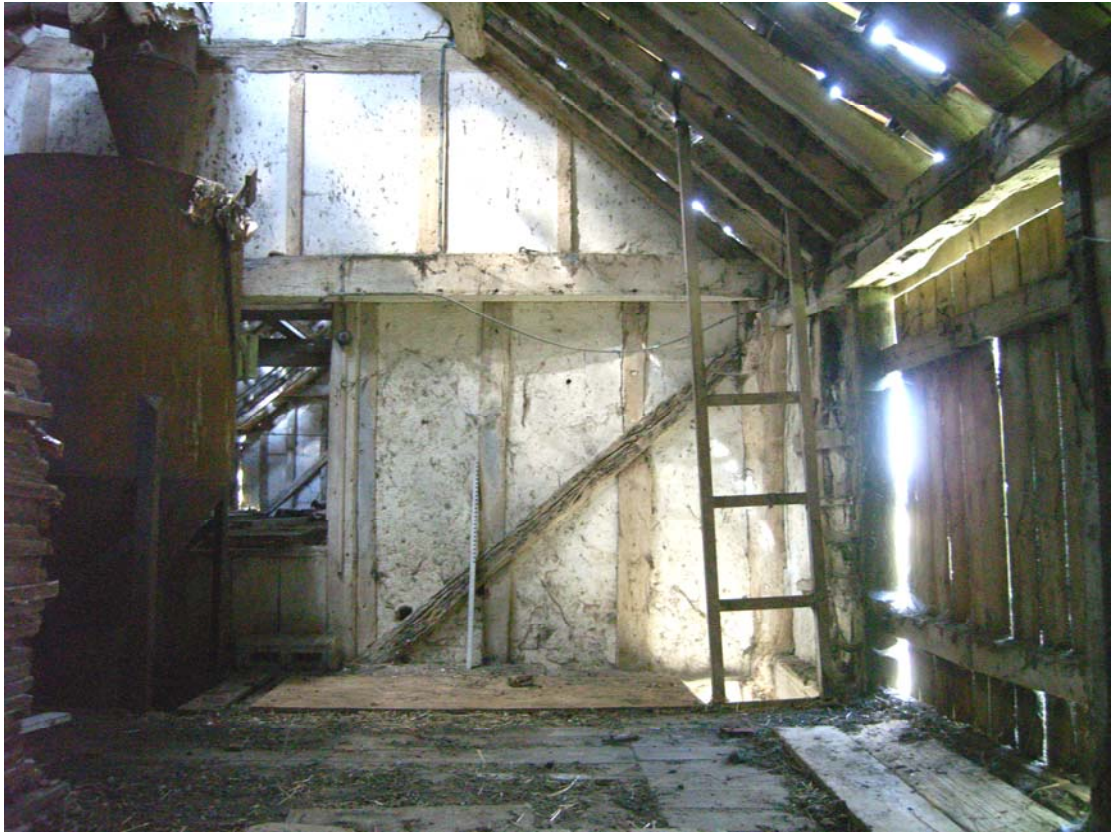
A2.15 First floor of rear wing looking north to original gable & ladder in north-east corner of bay 14 showing large hopper to left
