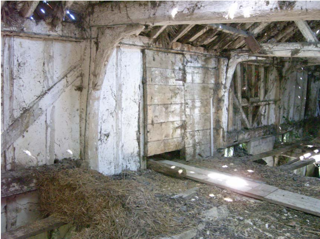
A2.11 Internal northern first floor elevation of bay 7 (centre) showing boarded door to rear wing and lower mid-rail than adjacent bays
