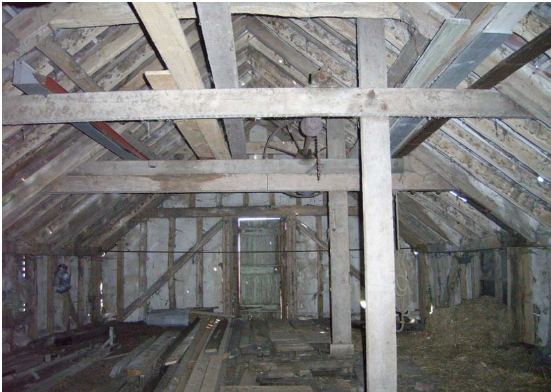
A2.16 First floor of bays 15-17 looking towards northern gable and showing sack hoist chain and wheel in roof
