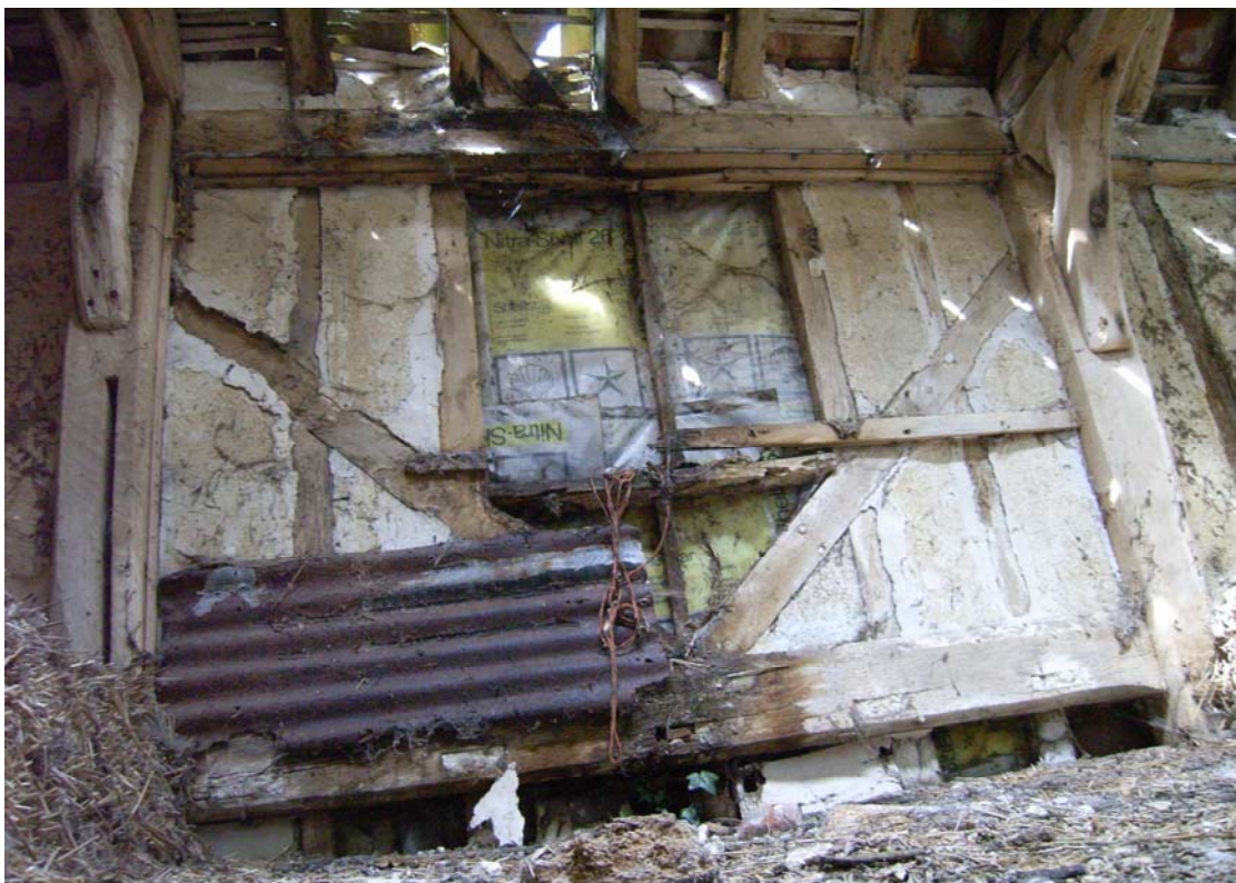
A2.8 First floor internal northern elevation of bay 3 showing high mid-rail 15 cm above floor and a blocked window aperture with original sliding shutter rails. Some timbers re-used.
