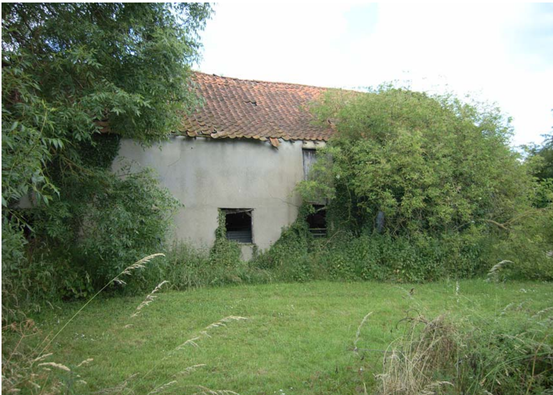
A2.2 Exterior of southern elevation showing easternmost bays with first-floor loading door in bay 10
