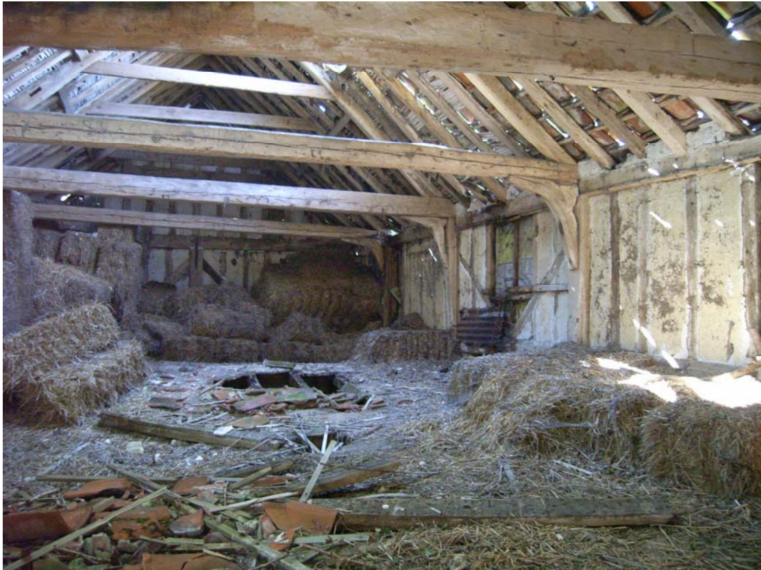
A2.7 First floor of southern range looking towards western gable with rear walls of bays 1-4 to right
