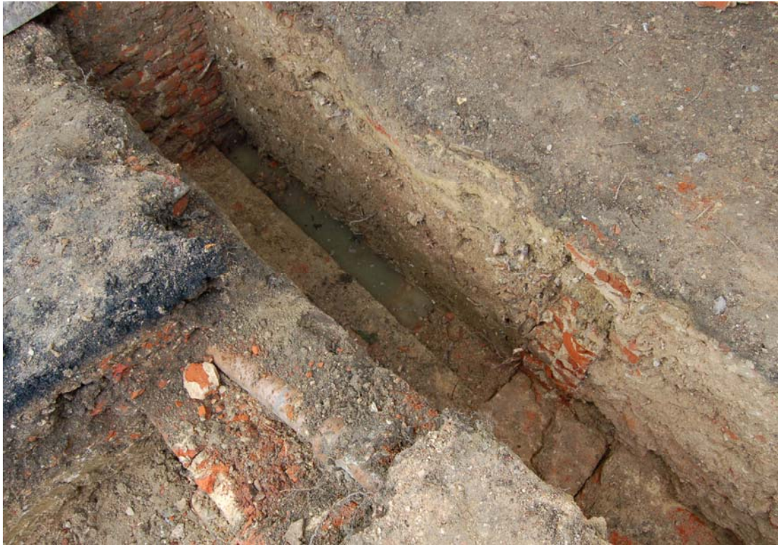
Figure 9. View of the construction trench for the rebuilding of the northeast wall of the 'study' wing, showing L-shaped foundation 0011 (in plan), overlying cellar wall 0010/0013 (in section) and cellar wall 0022 (in elevation, top left)
