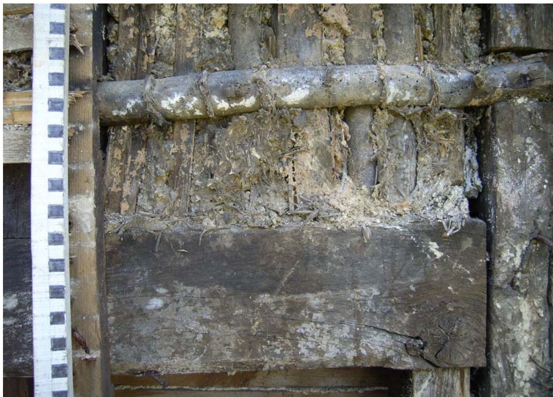
A2.6 Detail of external elevation H-I from east showing entrance door lintel (right-hand jamb lacking) and infill construction: Withy ties secure horizontal half-poles that are trenced and nailed against the exterior to vertical poles and half-poles between the studs.
