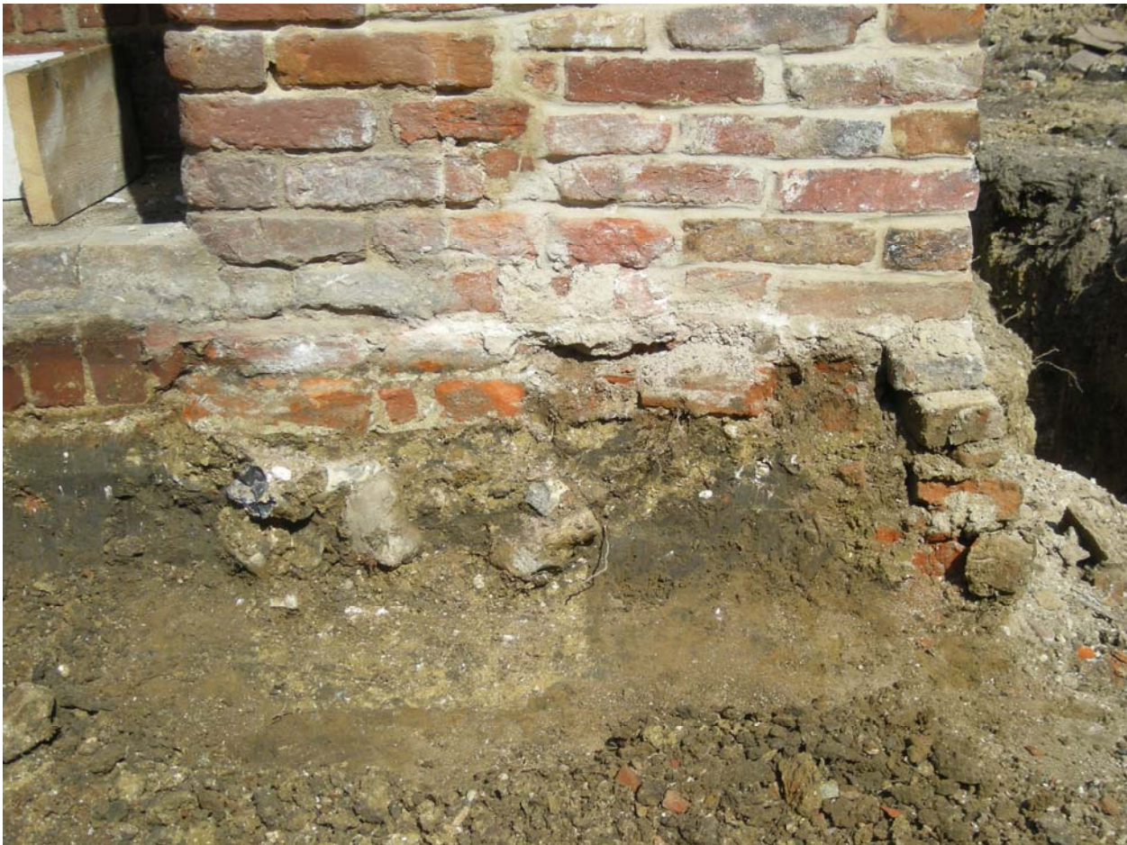
Plate 3. Part of the footing beneath the brick piers of the 17th century fireplace. The footing comprised a trench packed with yellow clay and large flints and would have been the only substantial piece below ground evidence that an early post-medieval building ever stood here at all.
