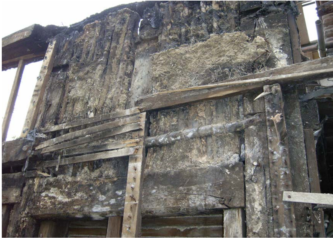
A2.5 Detail of external elevation H-I from east showing neatly chamfered original entrance lintel (bottom) with mason's mitres and original infill above (post I to right).
