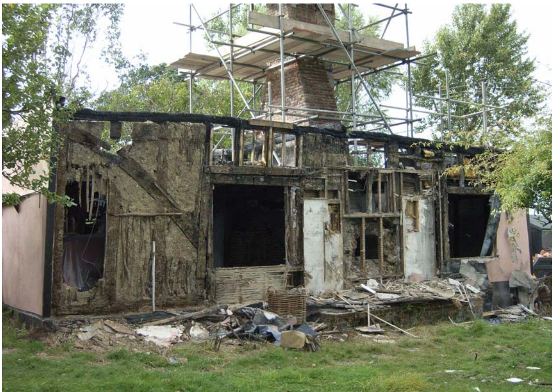
A2.2 External elevation H-N from south-east after commencement of demolition, showing original brace to left and infill of wattle-and-daub attached to externally trenched laths. A secondary bread oven against the eastern side of the chimney formerly projected beyond the plane of the wall.
