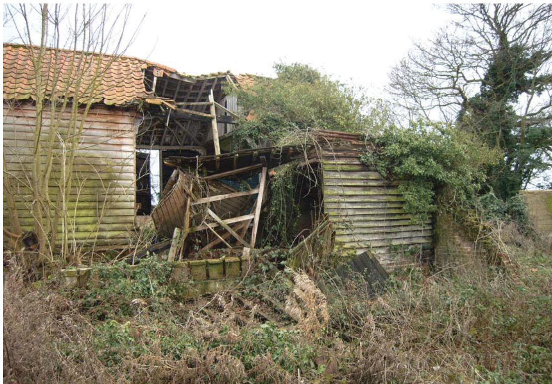
A2.8 Barn. Exterior from north-west showing collapsed porch with possible brick corner of demolished maltings to right
