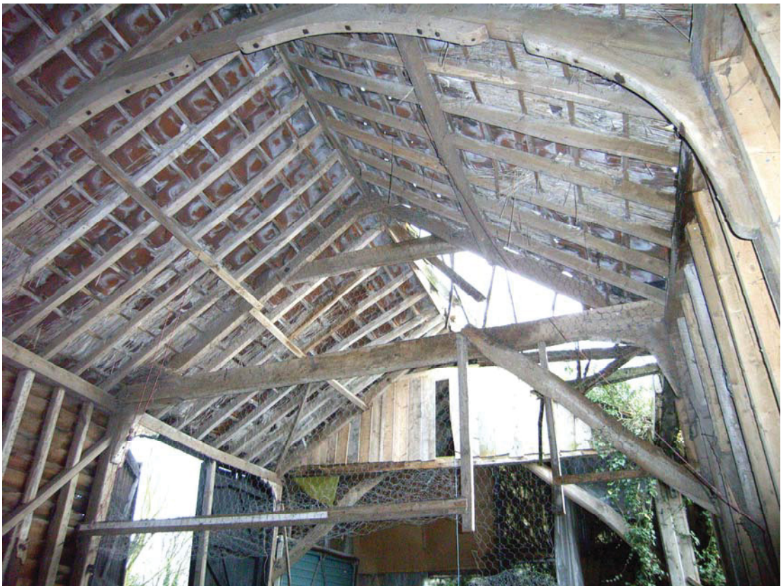
A2.10 Barn. Original butt-purlin roof structure viewed from north, showing secondary tie-beam braces
