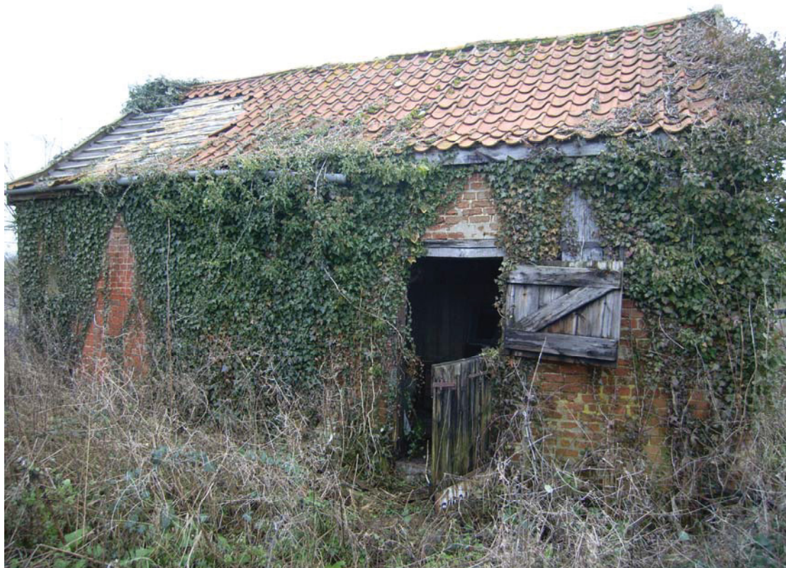
A2.4 Stable. Southern external elevation showing double-hung entrance door with hay loft hatch to right
