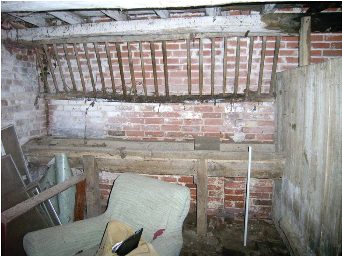
A2.6 Stable. Hay rack and manger against western elevation of southern stall (A1)
