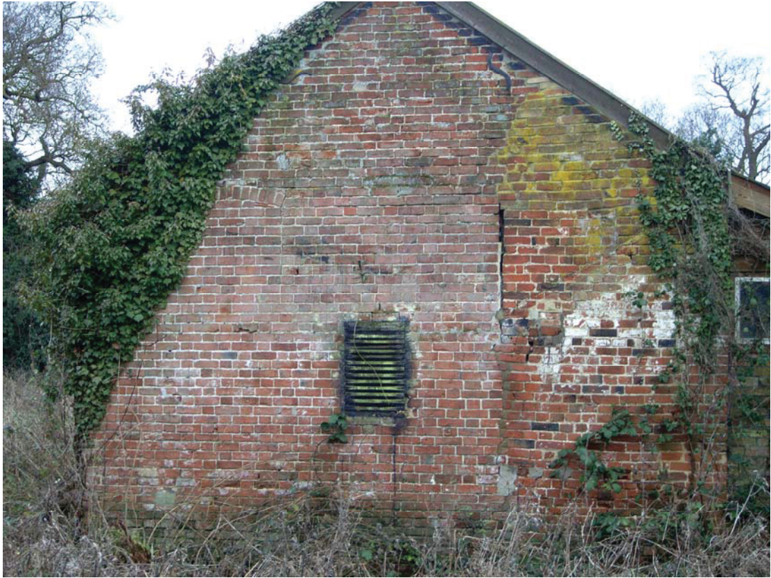
A2.5 Stable. Eastern external gable showing blocked window of original building to left with blocked door and scar of demolished eastern range to right
