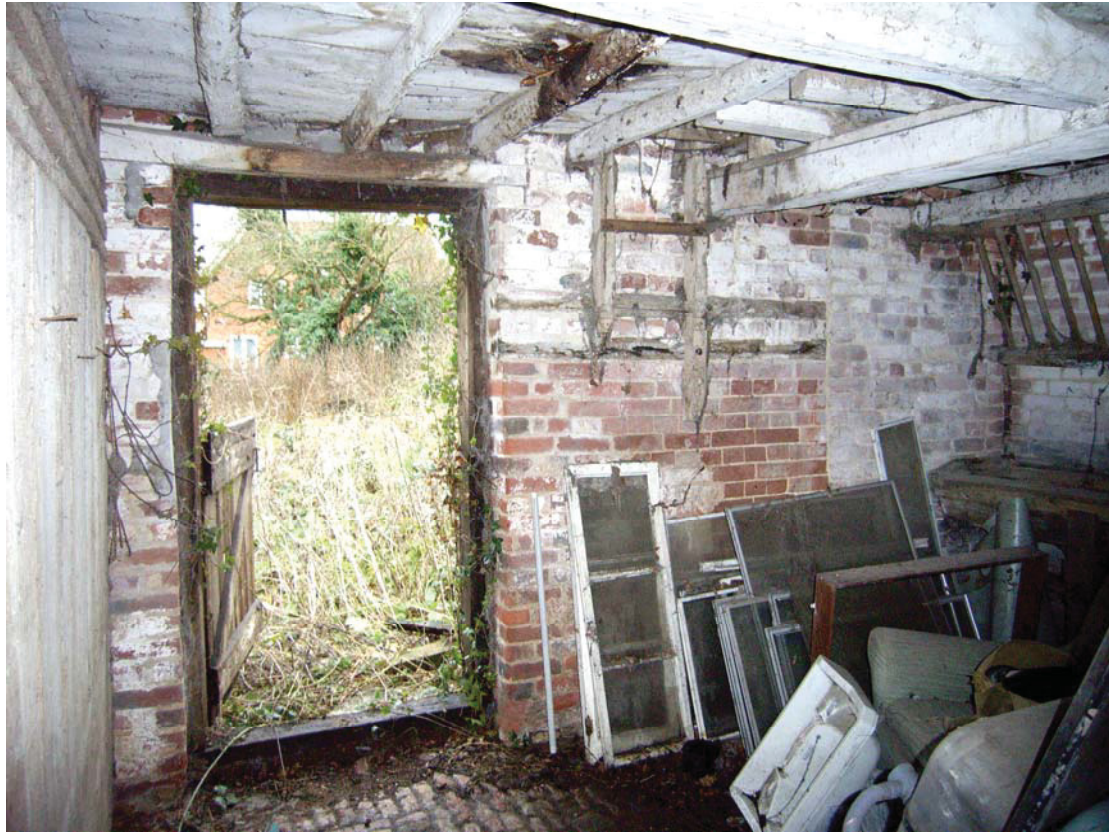
A2.7 Stable. Internal southern elevation of southern stall (A1) showing loft ladder to right of entrance, with vertical junction in brickwork & hay rack to right and boarded partition to tack room (A3) to left.
