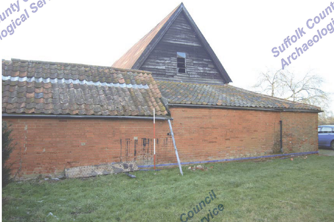
A2.3 External eastern elevation of barn showing 19 th century brick shed (7) in foreground
