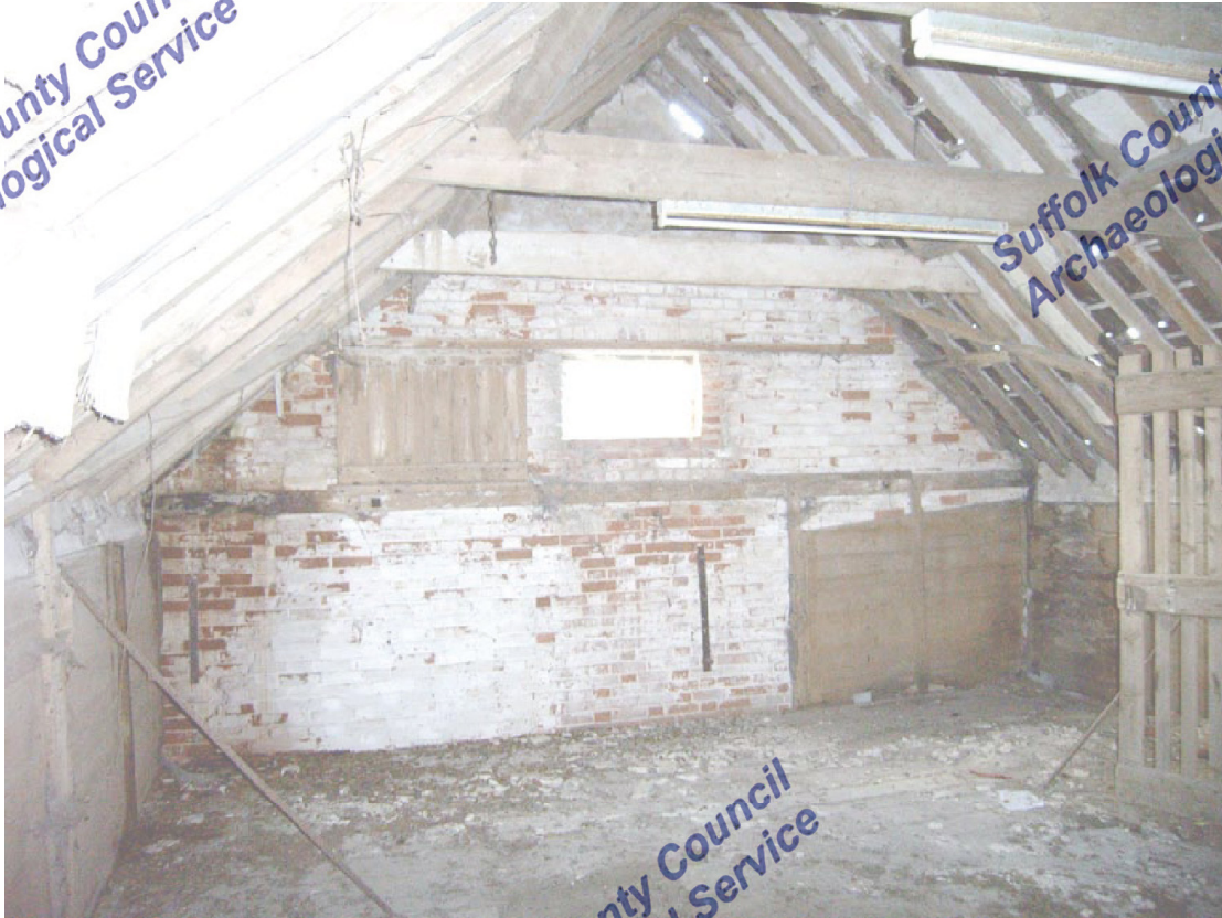
A2.5 Upper storey from east showing interior of western gable with evidence of grain bins to right & left
