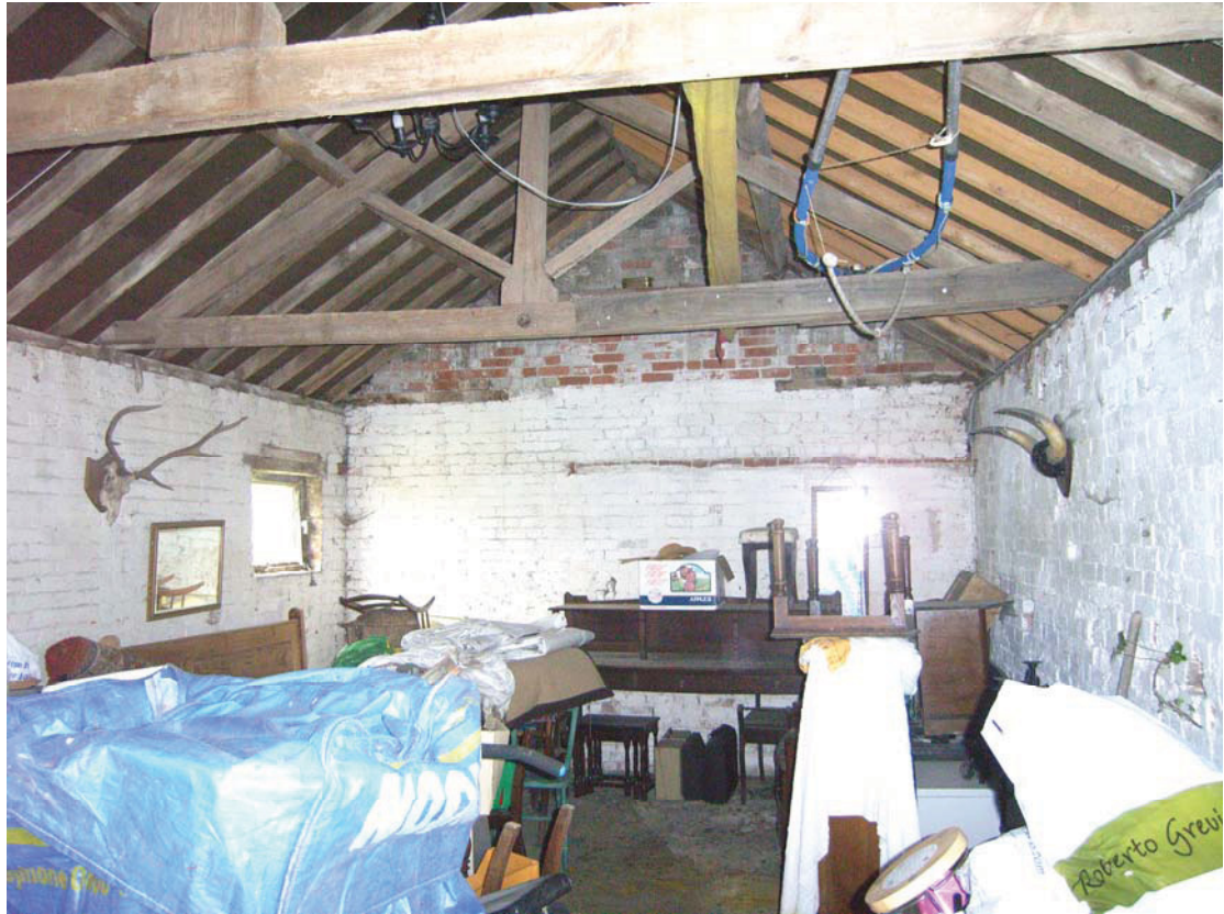
A2.7 Interior of shed C from north showing notches of manger to western elevation to right and original king-post roof
