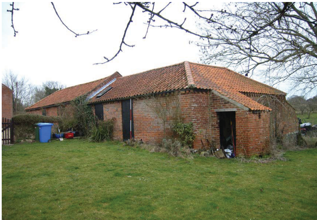
A2.2 Exterior from south-west showing privy against southern gable to right. Note the step in the roof which was designed to accommodate the slope of the ground
