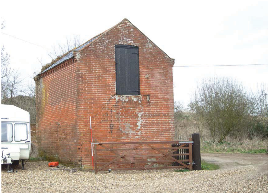
A2.8 Exterior of stable (3) from south-west showing scar of external stair to hay loft. Included for site context
