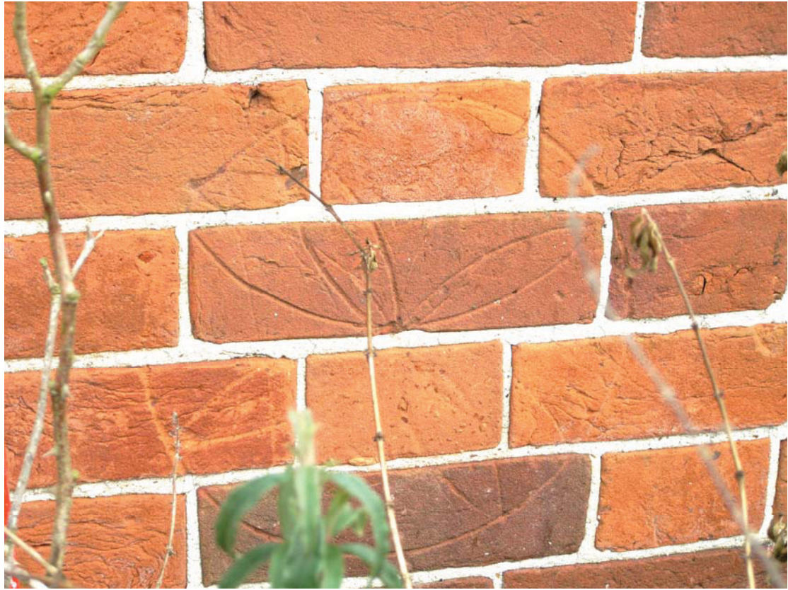
A2.5 Detail of 'daisy-wheel' apotropaic mark incised to brickwork of western external elevation
