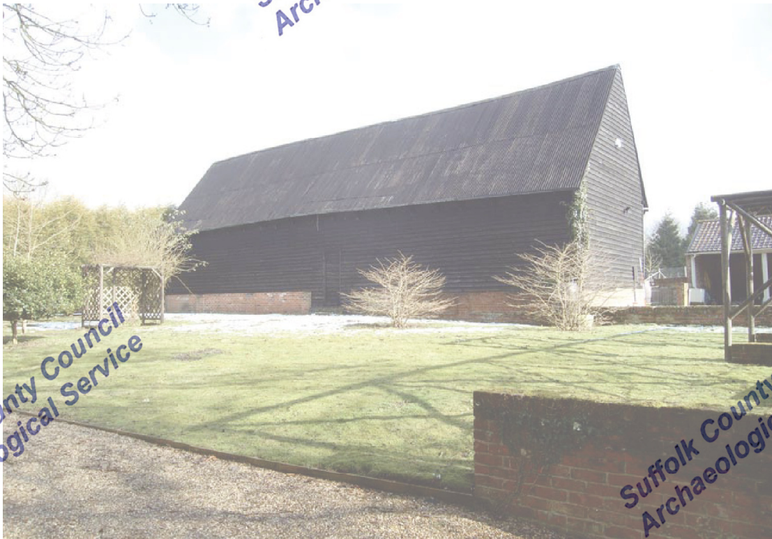
A2.2 Western external elevation from south-west showing blocked entrance in central bay (C) and brick shed to right
