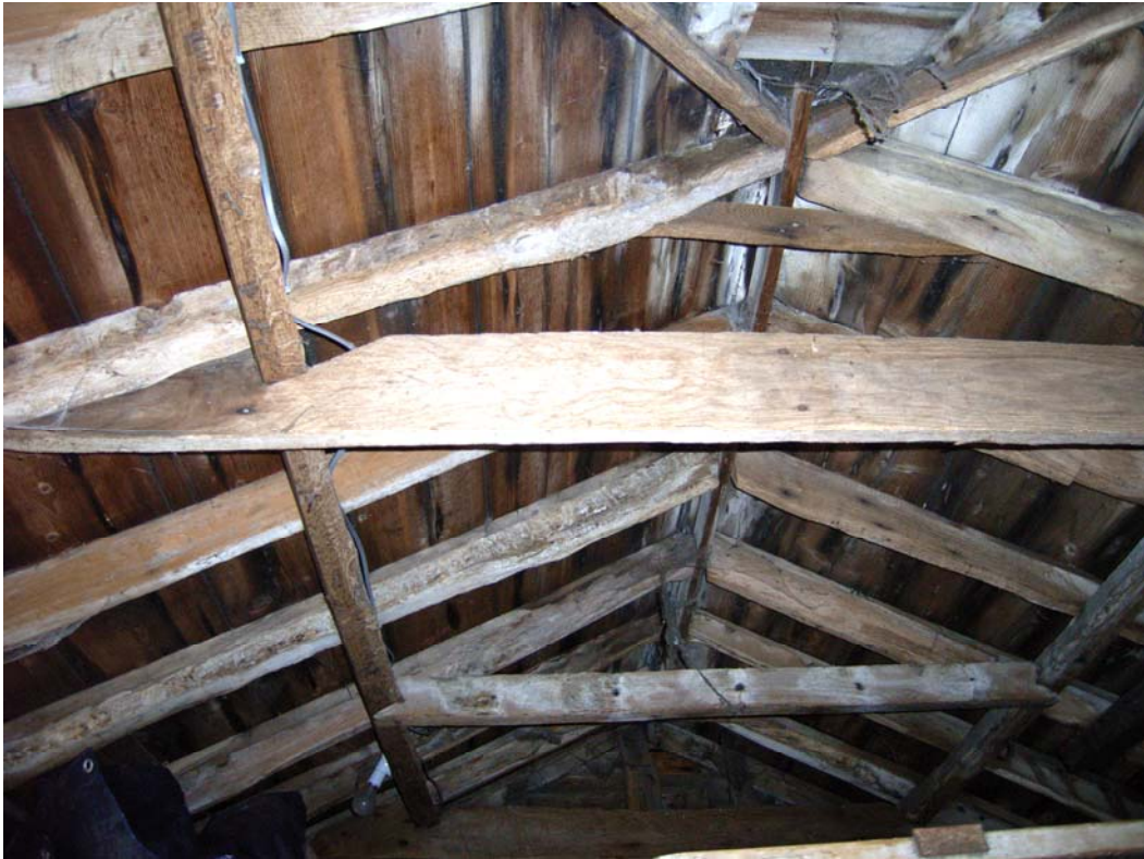
A2.9 Detail of original clasped-purlin roof structure with nailed collars seen from east in open shed
