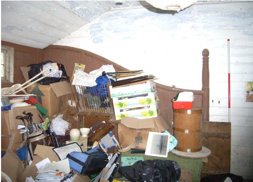
A2.7 Internal eastern elevation of stable (A) showing curved wainscot with turned finial and northern elevation to left
