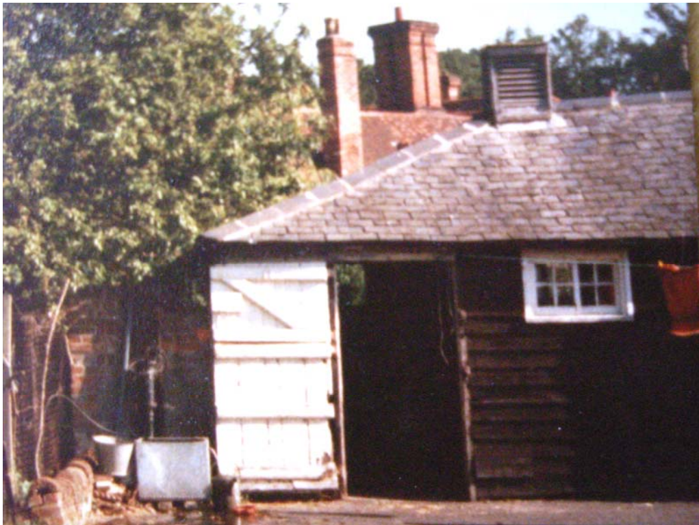
A2.4 Western end of southern external elevation as shown in a late-20th century photograph in the present owner's possession showing the original stable louver
