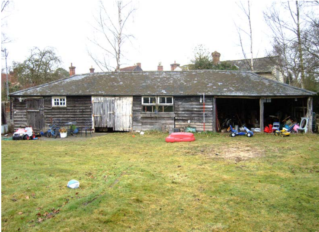
A2.3 External southern elevation showing stable to left and open shed to right
