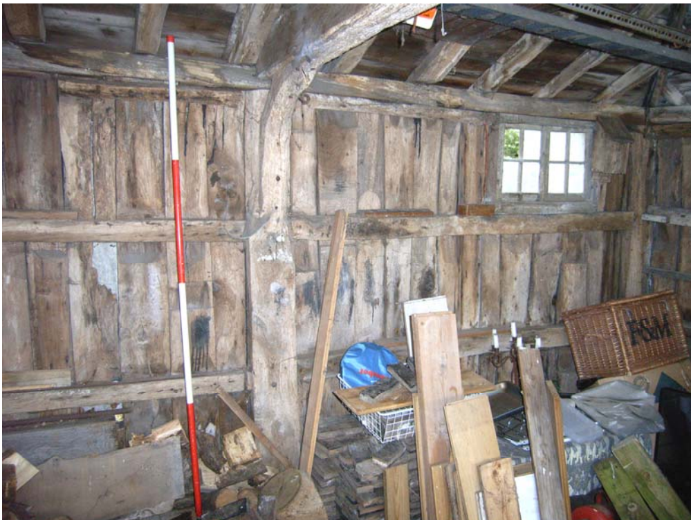
A2.8 Detail of board-and-rail construction of northern internal elevation of open shed (C) with bolted knee-brace to tie-beam. Eastern gable to right
