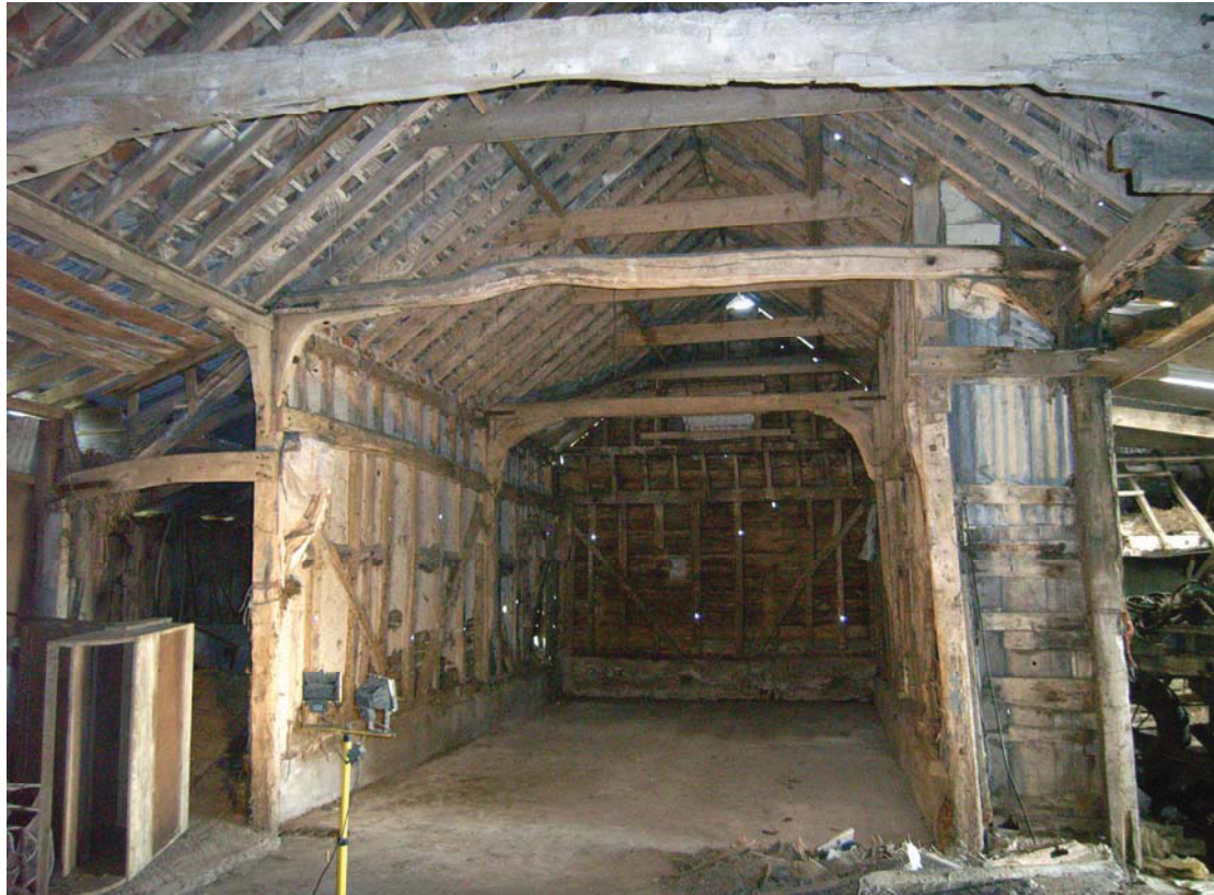
A2.5 General view of barn interior from west showing narrow 17 th century structure (A) with raised walls in rear and wider 18 th century structure (B) in foreground
