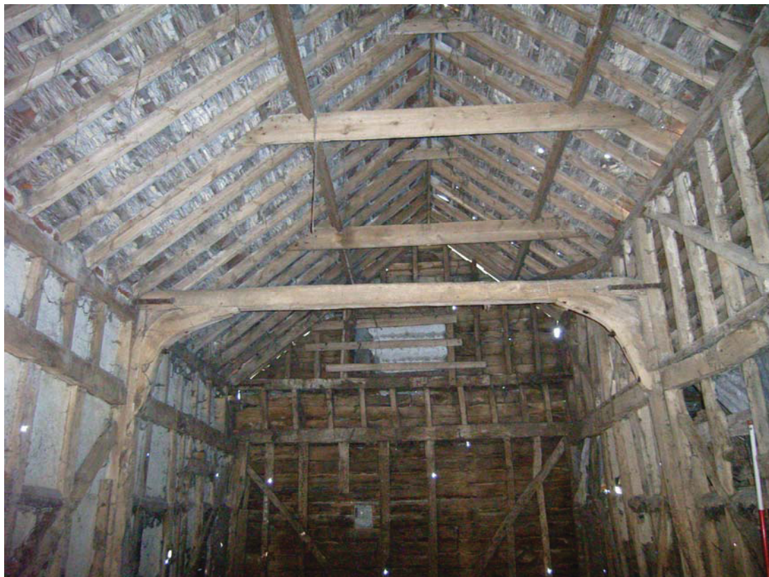
A2.8 19 th century roof structure from west showing greater height of roof raise in structure A to south (right). The raised tie-beam contains pegged mortises for a missing partition.
