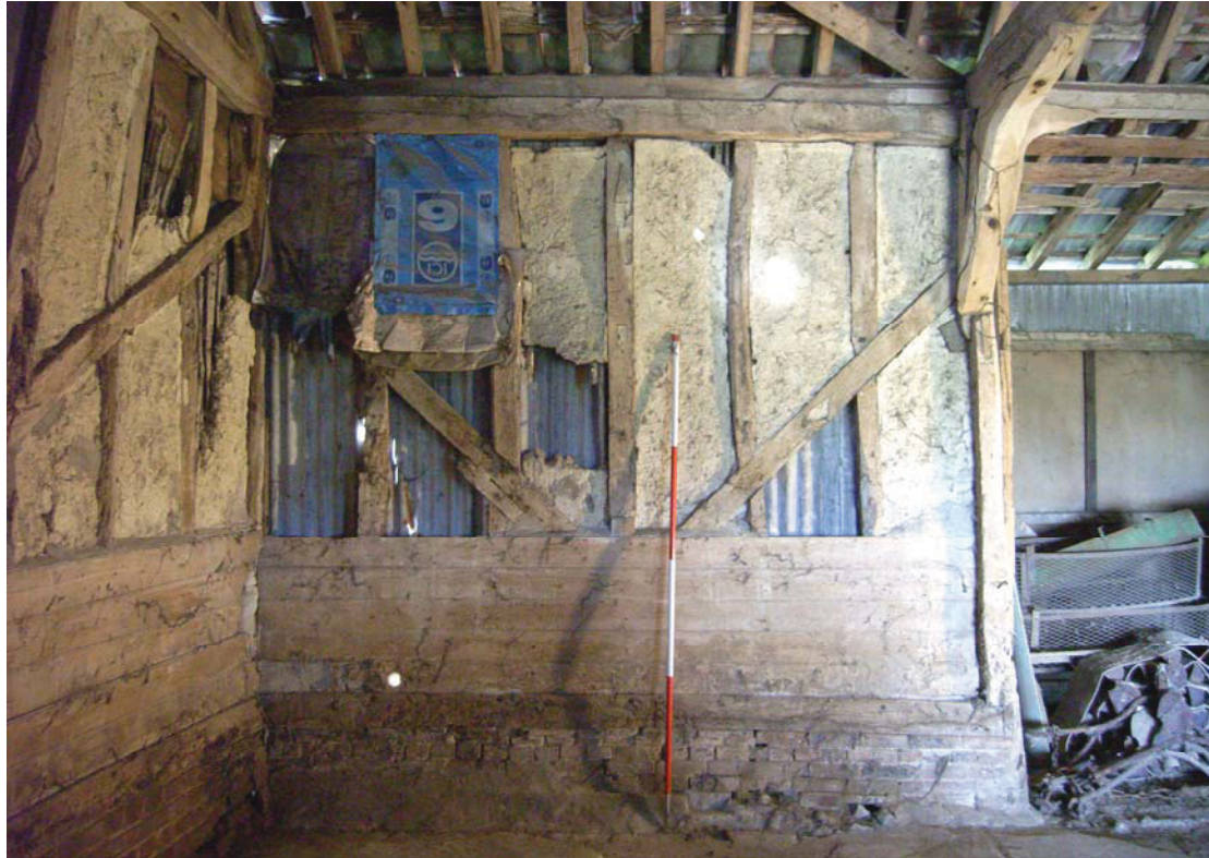
A2.6 Internal northern elevation of western bay (B1) showing original wattle-and-daub infill with entrance bay to right (B2) and re-used ovolo-moulded window mullion in western gable to left
