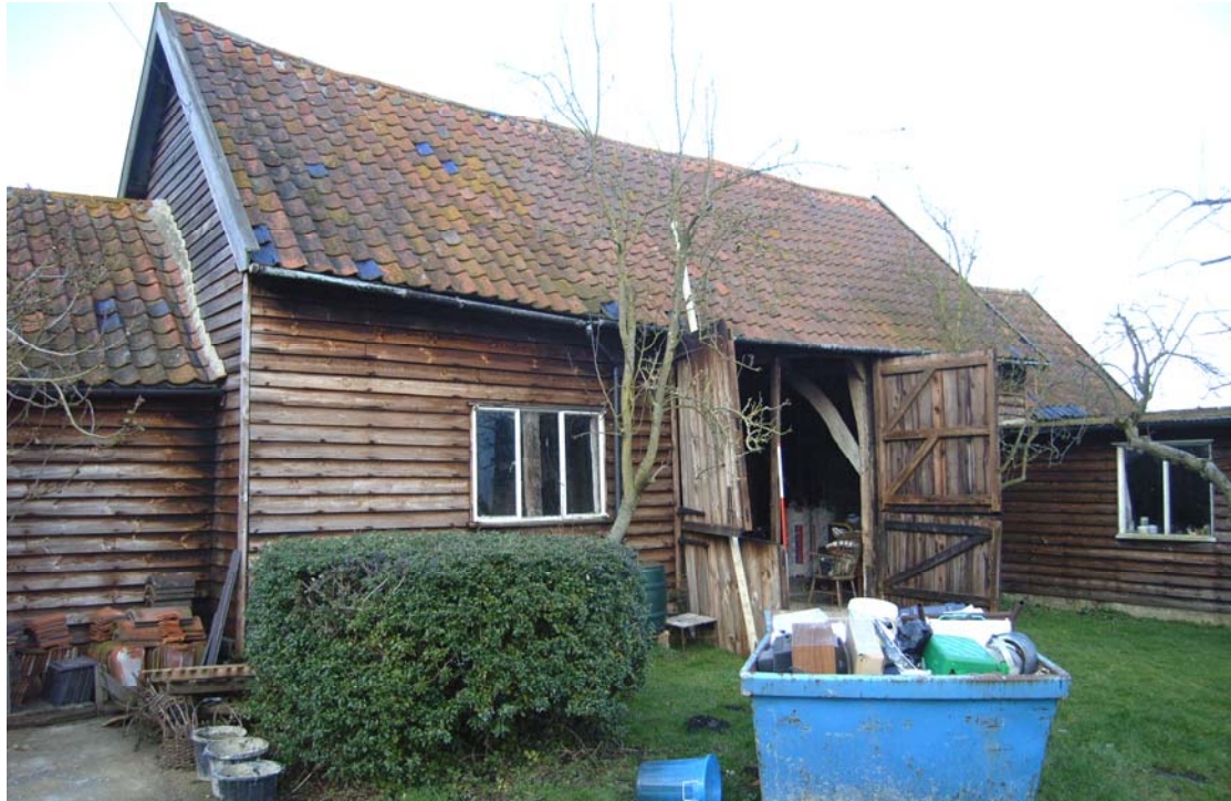
A2.3 Southern external elevation of barn from south-west showing double-hung doors original 17 th century entrance bay (A2) to right & 18 th century extension bay (b) to right. The sheds to right and left are modern.
