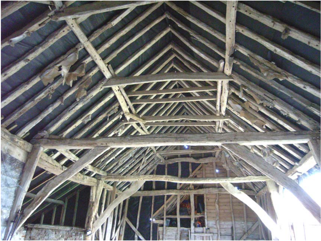
A2.5 Barn roof structure from west showing clapsed purlins with wind brace mortises in principal rafters, and profile of stable roof in rear
