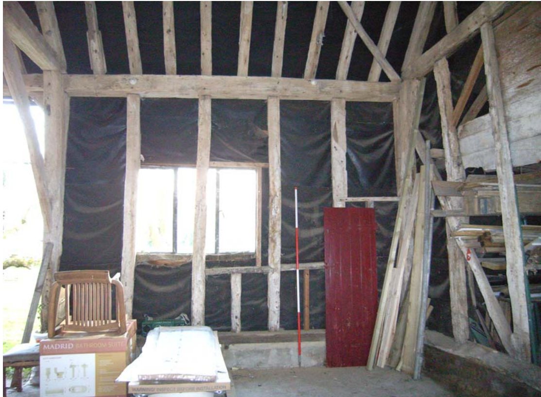
A2.7 Southern internal elevation of western bay (A1) showing original wall studs with mortises and trench for missing internal brace to right.
