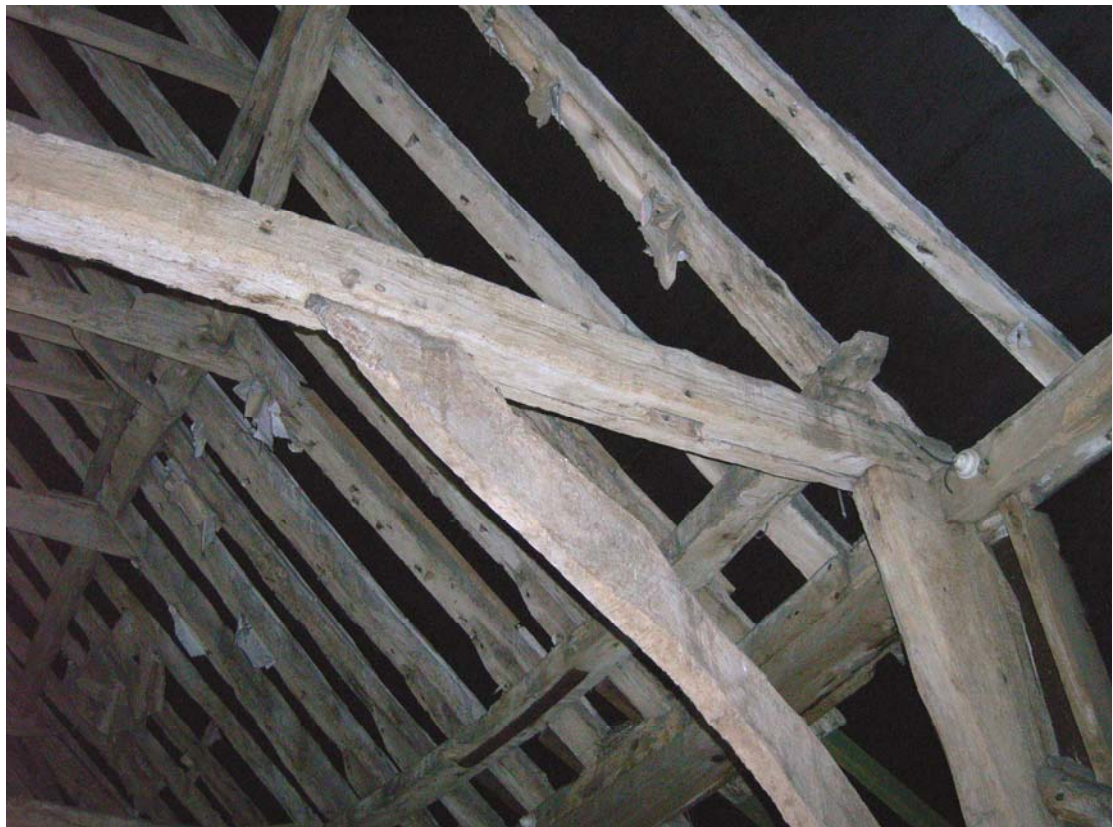
A2.8 Detail of weathering to eastern elevations of tie-beam & north-eastern corner post of original barn (A).
