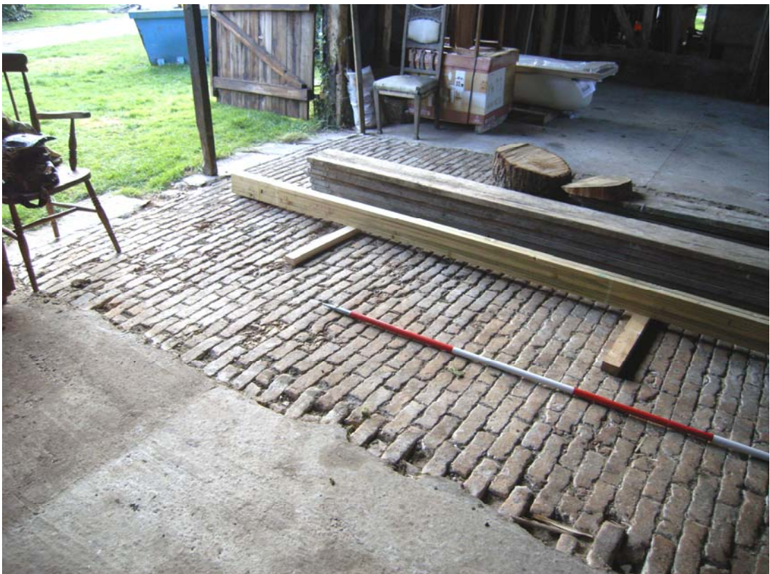
A2.6 Brick threshing floor in bay A2 seen from north-east, showing southern entrance to left
