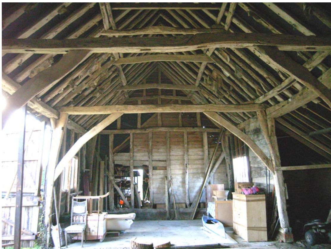
A2.4 General view of barn interior from structure B to east, showing 18 th century arch-braces and stud mortises of original eastern gable in tie-beam, & 17 th century arch-braces of structure A in rear
