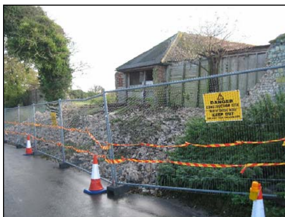
Plate 1 Collapsed wall section
