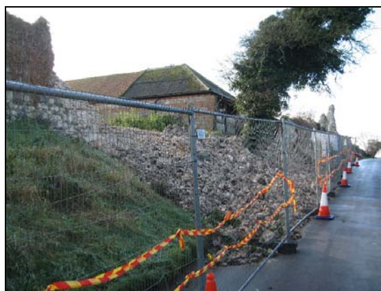
Plate 2 Collapsed wall section
