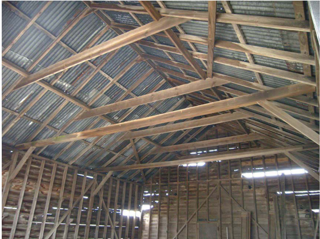
A2.7 Enclosed sheds (2). Detail of original softwood roof structure of western shed viewed from west, showing gable adjoining eastern shed to right
