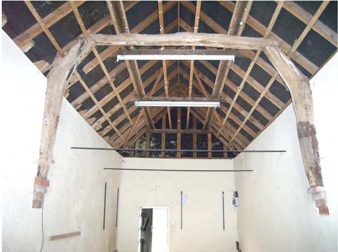
A2.5 Brick shed (1). Apparently original open truss of recently rebuilt roof from north
