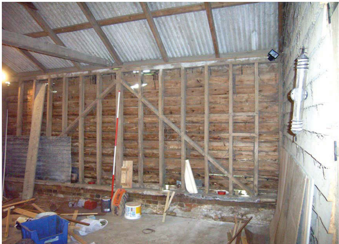
A2.8 Enclosed sheds (2). Internal southern elevation of lower eastern shed showing original 20 th century wall fabric.
