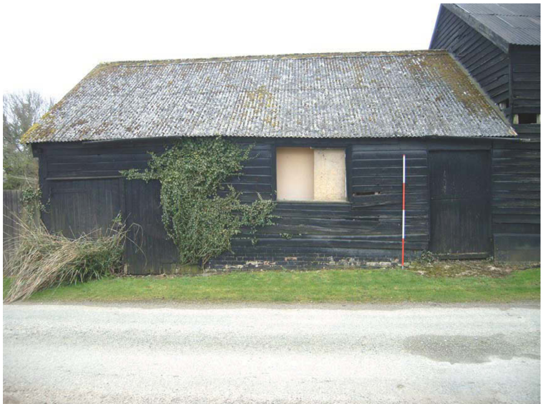
A2.6 Enclosed sheds (2). External northern elevation of eastern enclosed shed, showing double doors to vehicle compartment to left and double-hung doors to right
