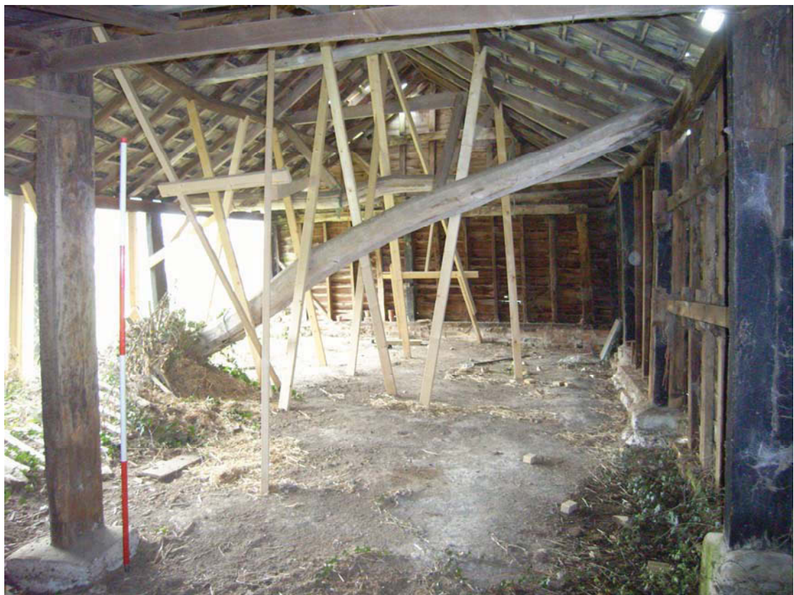
A2. 10 Open shed (3). Interior from east showing modern props and collapsed tie-beam
