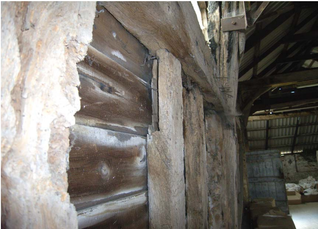
A2.12 Detail from south of door head mortise and external chamfers beneath mid-rail in western elevation of barn
