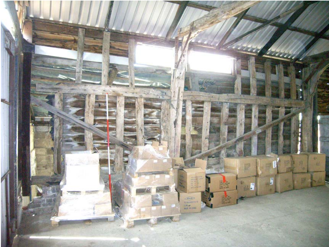
A2.11 Internal western elevation of barn showing 16th century framing with intact mid-rails but lacking roof-plate and evidence of arched doorway to left (diagonal braces are secondary)
