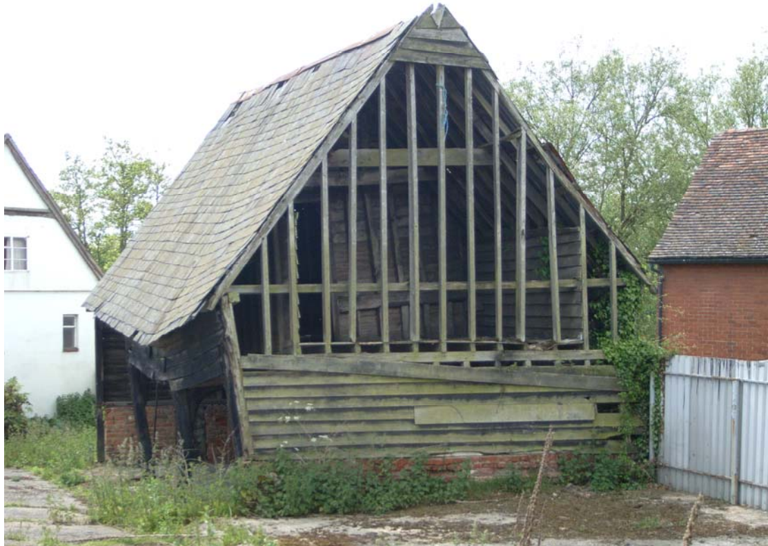
A2.5 Northern external elevation of granary showing internal partition through exposed studwork and open eastern elevation, with farmhouse in rear to left
