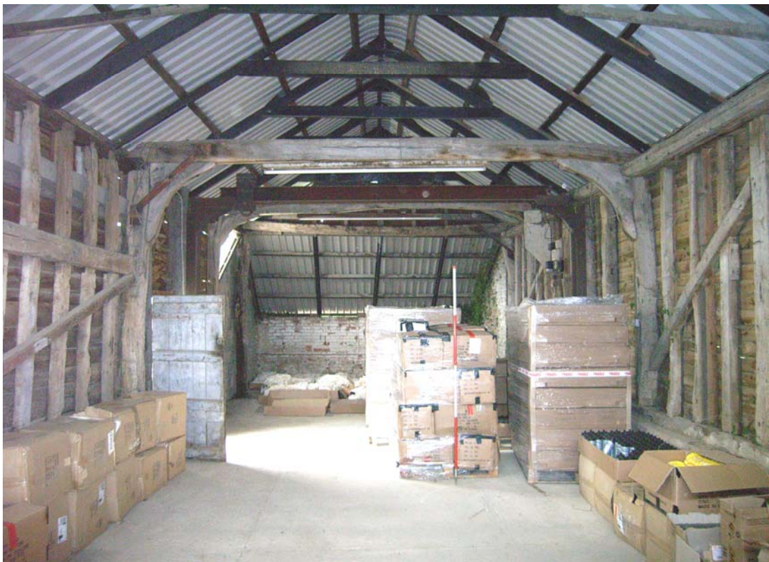
A2.10 General internal view of barn from south showing modern roof structure with 16 th century timber-framing of western elevation to left
