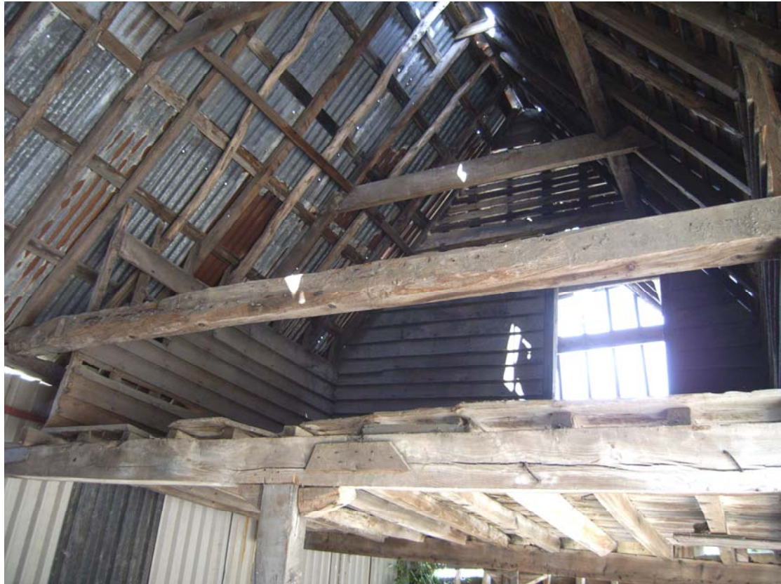
A2.7 Interior of granary from south showing original clasped-purlin roof structure and boarded granary floor with doorway to northern compartment (floor removed from southern bay in foreground)
