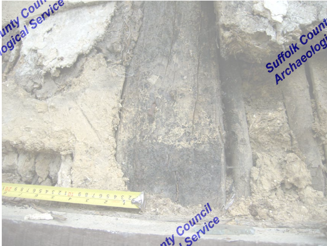
A2.7 Detail of sooted original stud and daub beneath later plaster of internal gable C-D
