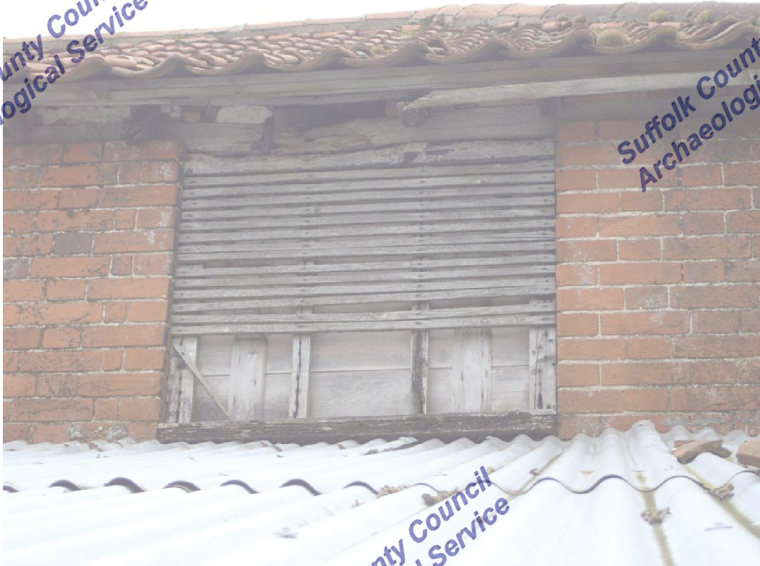
A2.5 Detail of original louvered window in western external elevation of granary
