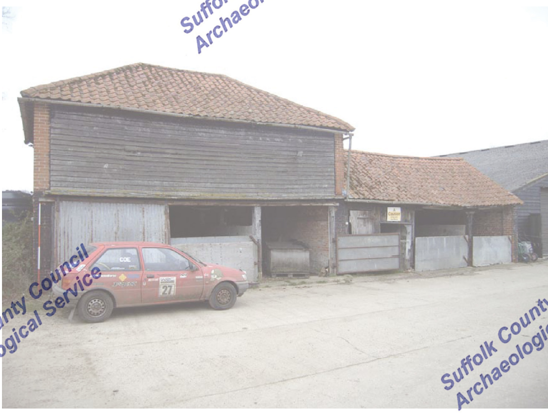
A2.2 Eastern external elevation of granary showing open arcade to ground floor and later single-storied shed to right
