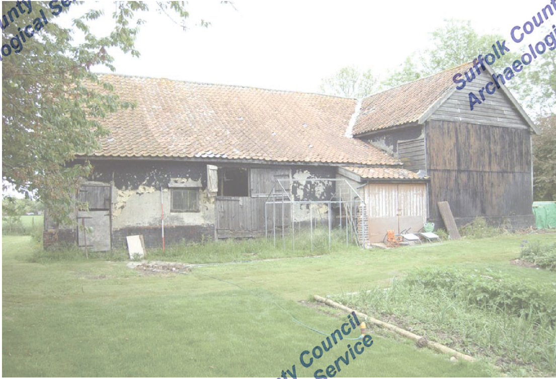
A2.1 Southern external elevation from south-west showing doors to lean-to shed (B) and porch (C) to left with gable of floored eastern range to right
