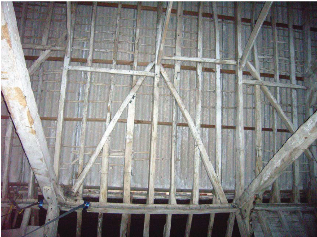
A2.8 Detail of staggered butt-purlin roof of early-19 th century structure (A3) from west
