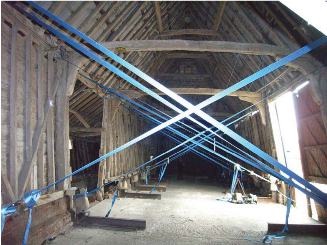
A2.5 General internal view of barn from north showing modern bracing straps.
