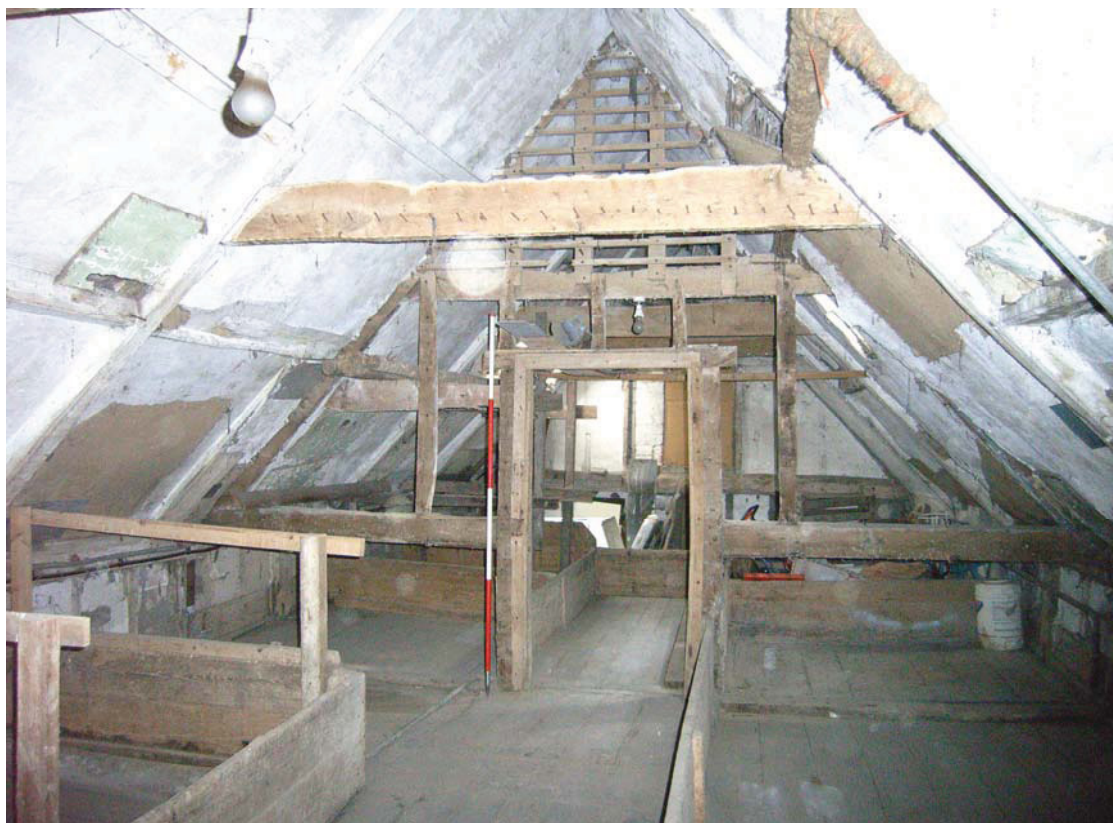
A2.12 Interior of first-floor granary (B1) from south, showing 19 th century grain bins with central passage and butt-purlin roof structure
