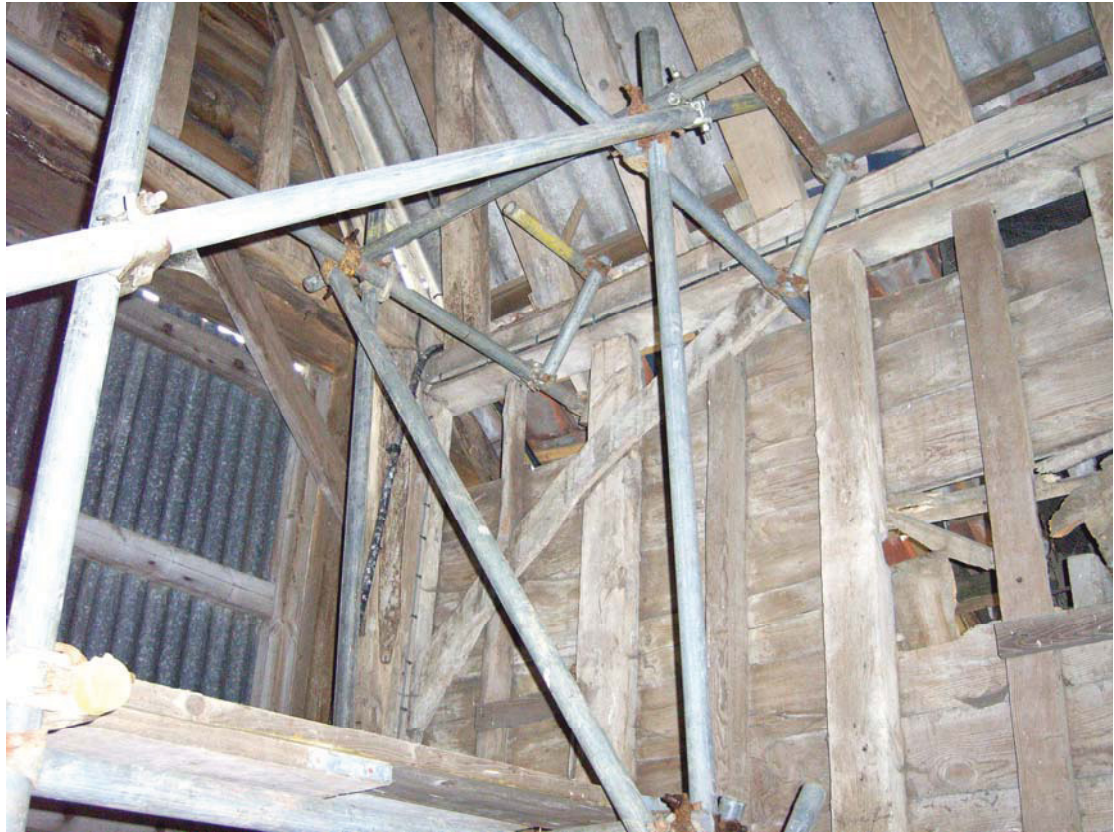
A2.9 Detail of original internal corner brace and studs in eastern elevation of mid-17 th century northern extension bay (A2). The northern gable to the left has been rebuilt
