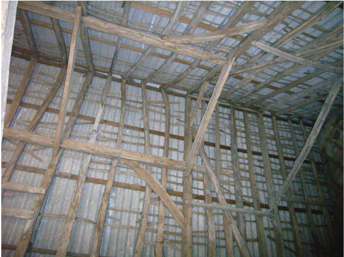
A2.7 Southern end of original 17th century roof (A1) seen from west, showing wind braces and original hip collar in centre
