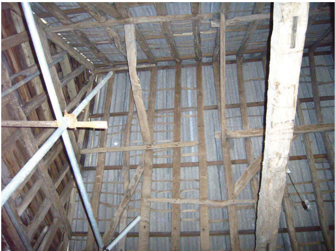
A2.6 Northern end of roof from west showing wind braces of original 17 th century open-framed gable right (A1) & former hipped gable of mid-17 th century extension bay (A2) left
