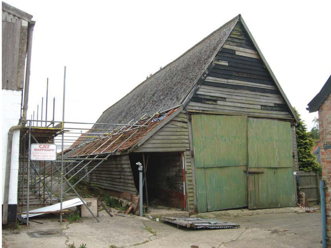
A2.3 Exterior of barn from north-west showing northern gable with steeply pitched roof (formerly thatched) and rear lean-to (A4) to left
