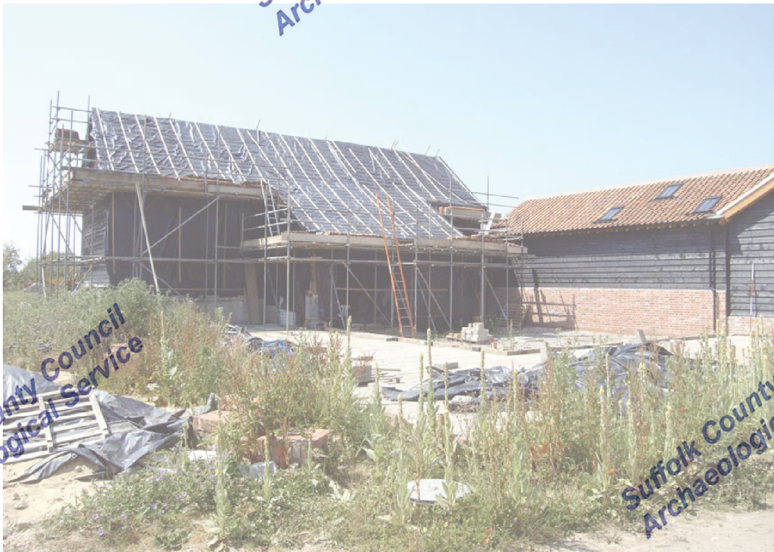
A2.2 Eastern yard from south-east, showing site of demolished southern shed to left
