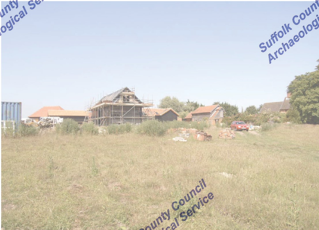
A2.1 General view from south-west, showing house to right with barn in centre & new development in rear
