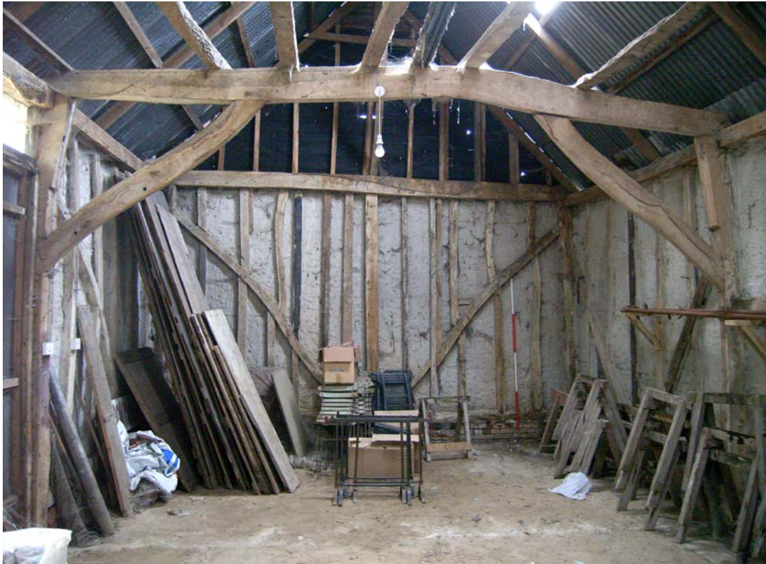
A2.5 General internal view of barn from north showing original arch braces to southern tie-beam, with original chalk floor and primary wall bracing.
