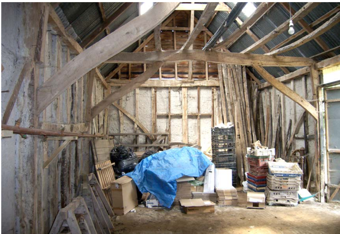
A2.6 General internal view of barn from south showing original arch-braces & central entrance to right. The roof structure is modern but a number of original rafters are lodged on the tie-beams and leaning against the northern gable.
