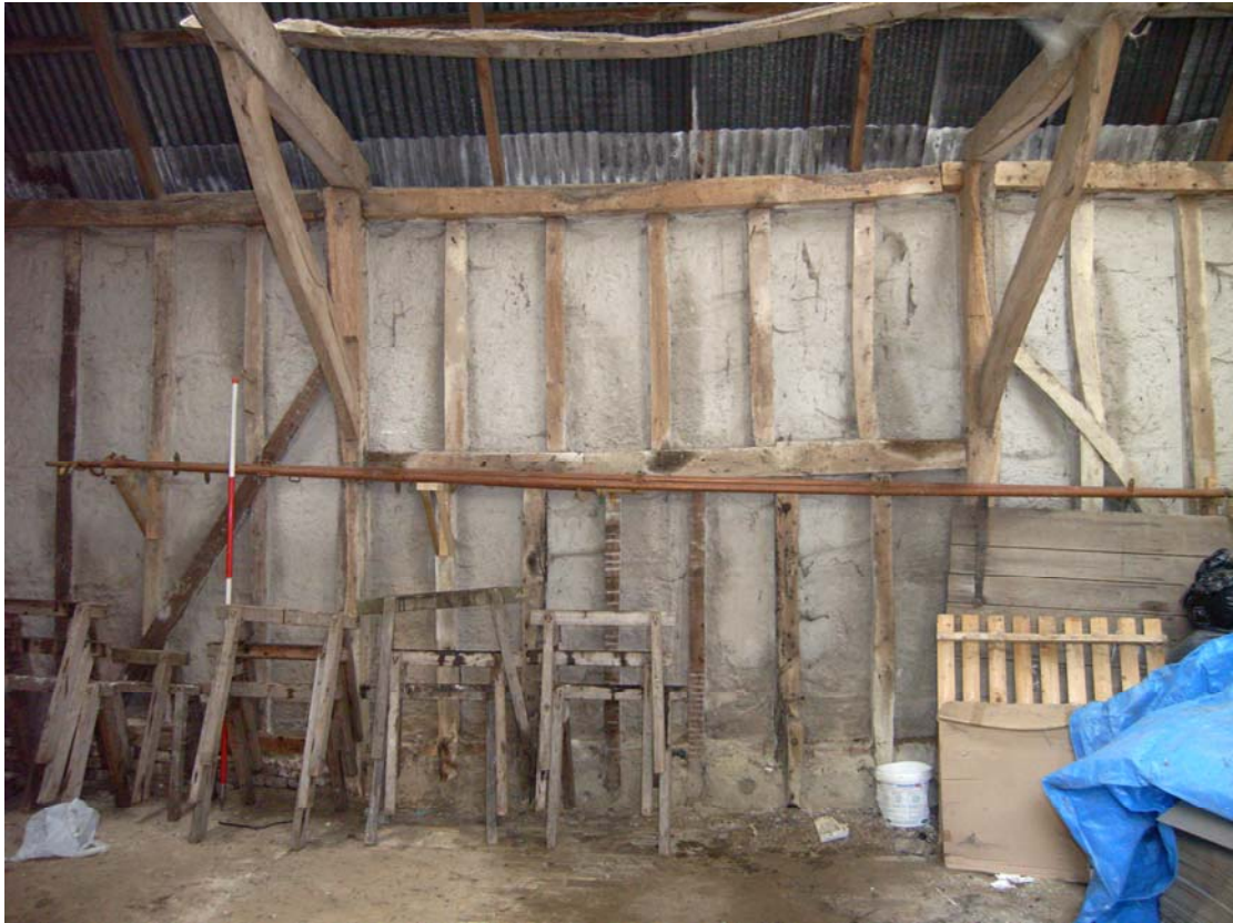
A2.7 Internal bay of western internal elevation showing the original lintel of the rear door (the door now blocked by the central pair of narrow studs, but the jambs intact)
