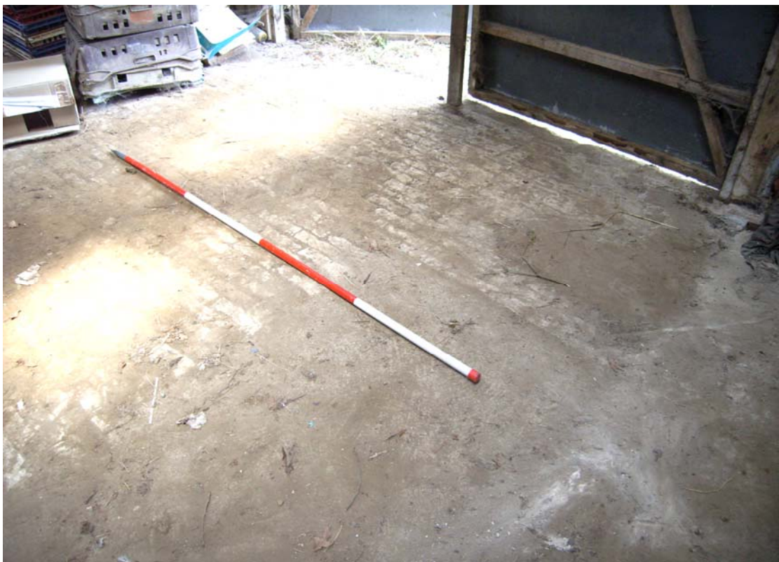
A2.8 Gault brick threshing floor of the central bay seen from south-west, with the original rammed chalk floor of the southern bay to the right
