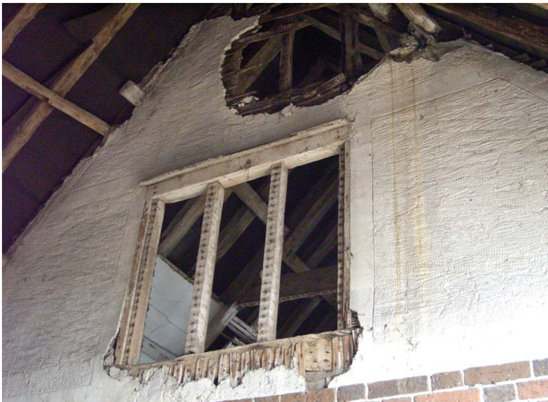
A2.8 Detail of window and pargeting to north-western gable of granary (1) from roof of later stable (2). The original window mullions contain nails for missing louver slats
