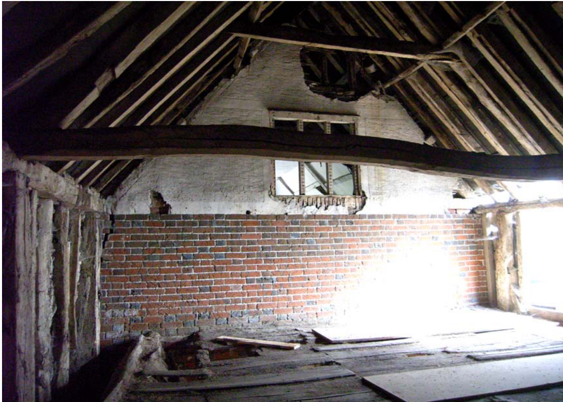
A2.7 North-western external gable of brick stable & granary (1) seen from roof of later stable (2), showing original pargeted but unpainted lime plaster above brickwork. The remains of the hay rack and loading vent in the loft floor are visible to bottom left
