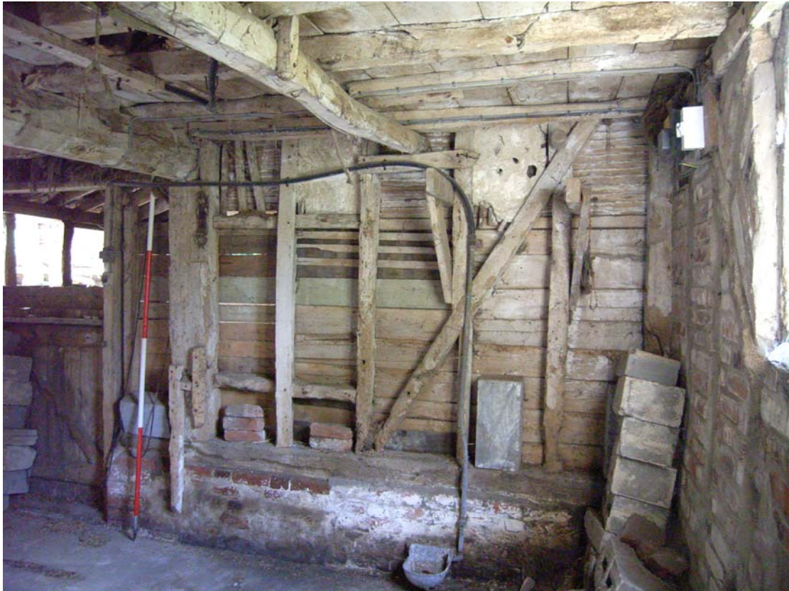
A2.9 Internal south-western elevation of stable (2) showing primary bracing of studwork and harness hooks to right.
