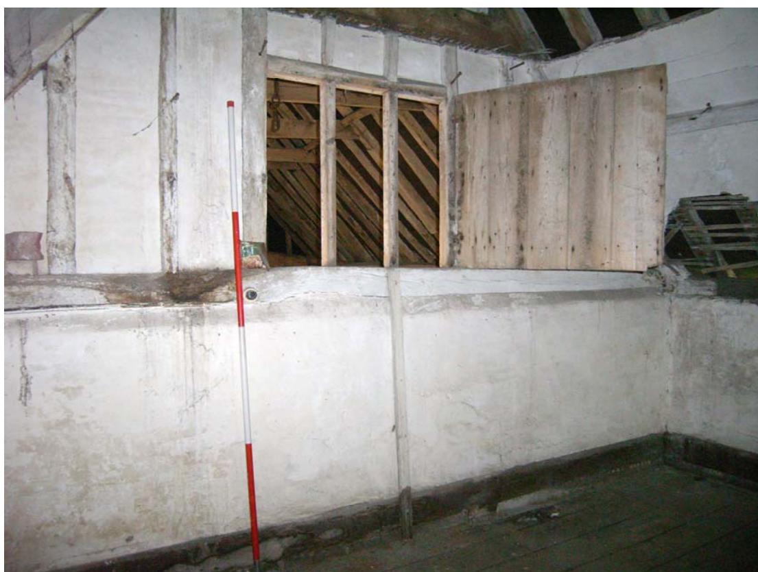
A2.6 Internal north-western gable of first-floor granary (1) showing original window & hinged internal shutter
