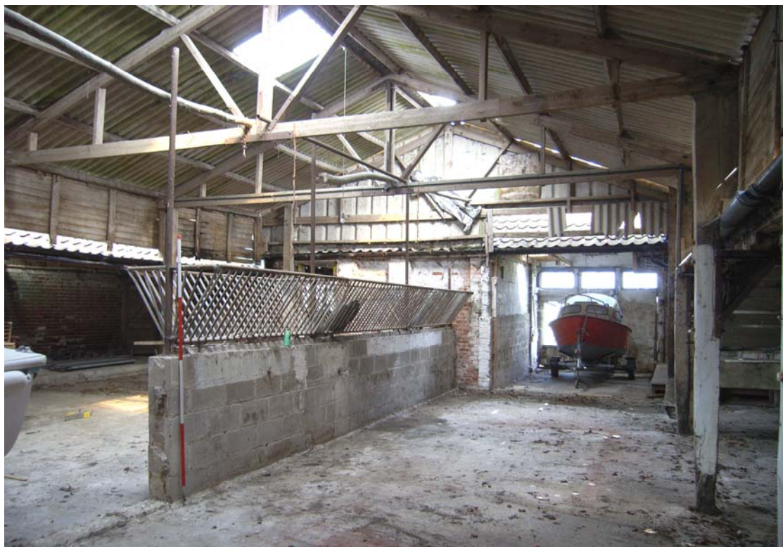
A2.10 Northern end of yard B beneath 20 th century roof showing shelter shed 10 to left and shelter shed 12 to right (all posts renewed) with 20 th century cattle hay rack in centre
