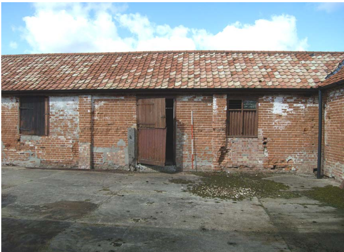
A2.6 North-western corner of yard A (right) showing the original doorway and window to shed 3
