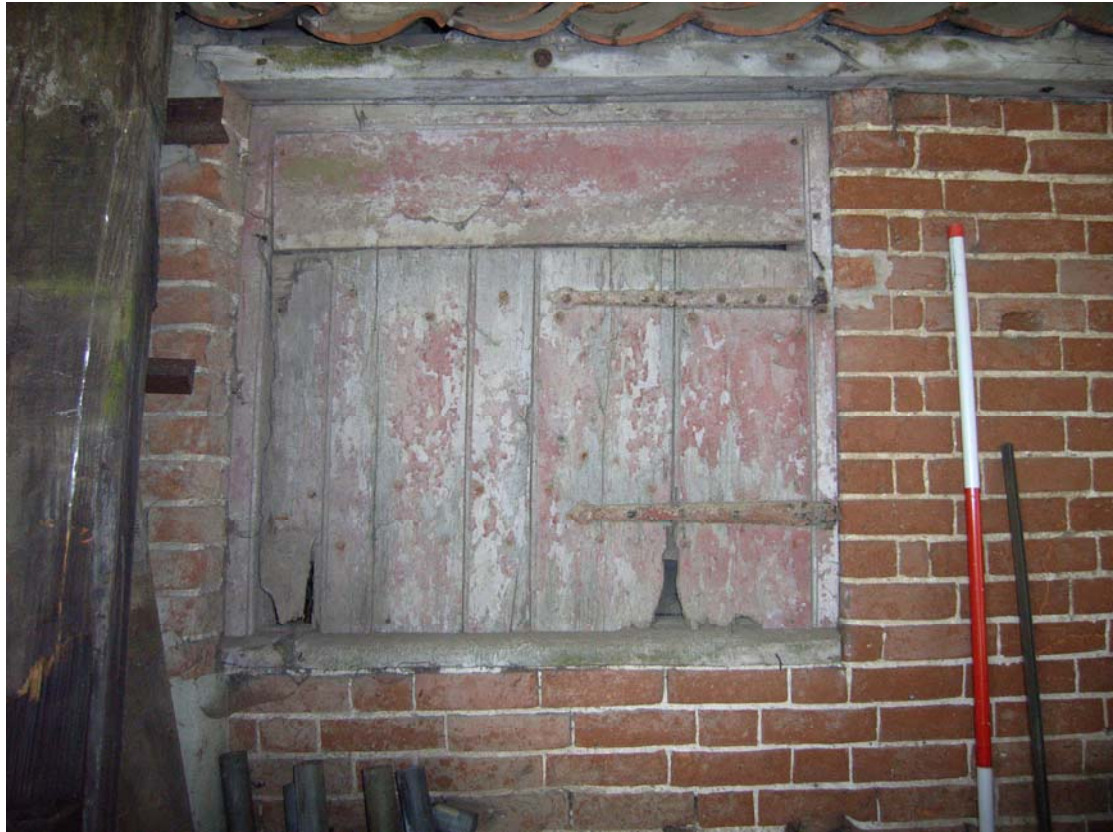
A2.9 Detail of reddled hatch in external northern elevation of shed 4 (within area of apparent horse mill shown on Ordnance Surveys).
