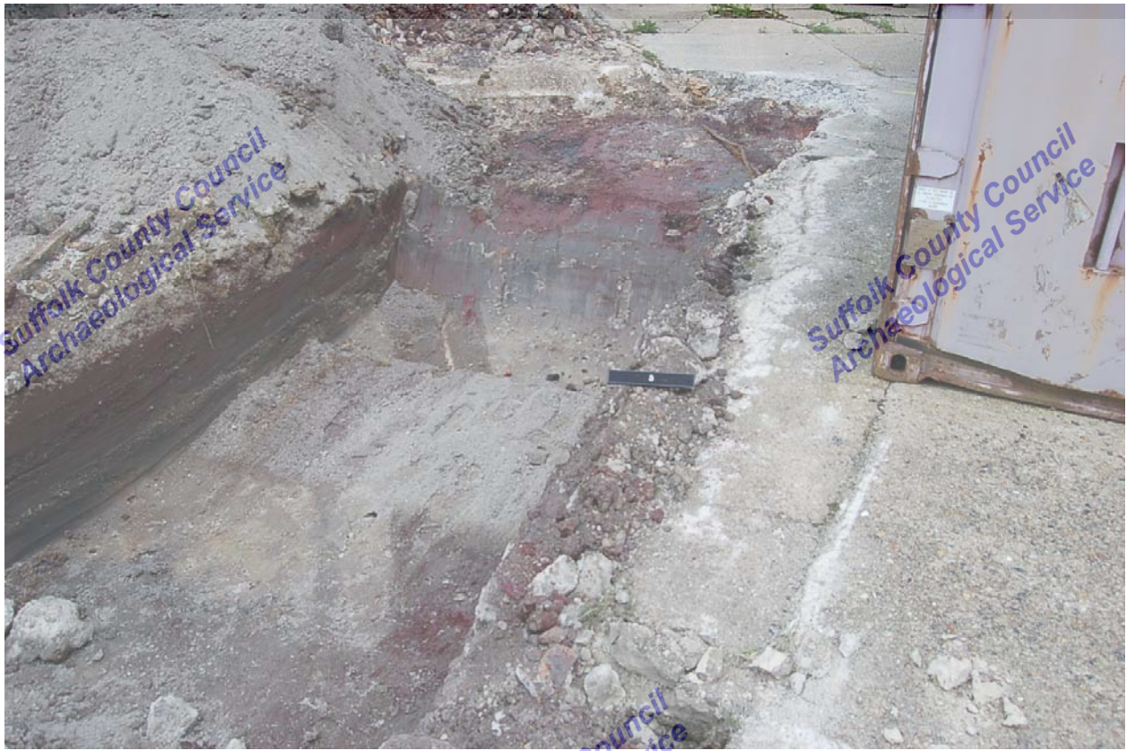
Plate 3. Trench 3, facing north, showing unidentified pipes in centre and northern end of trench.
