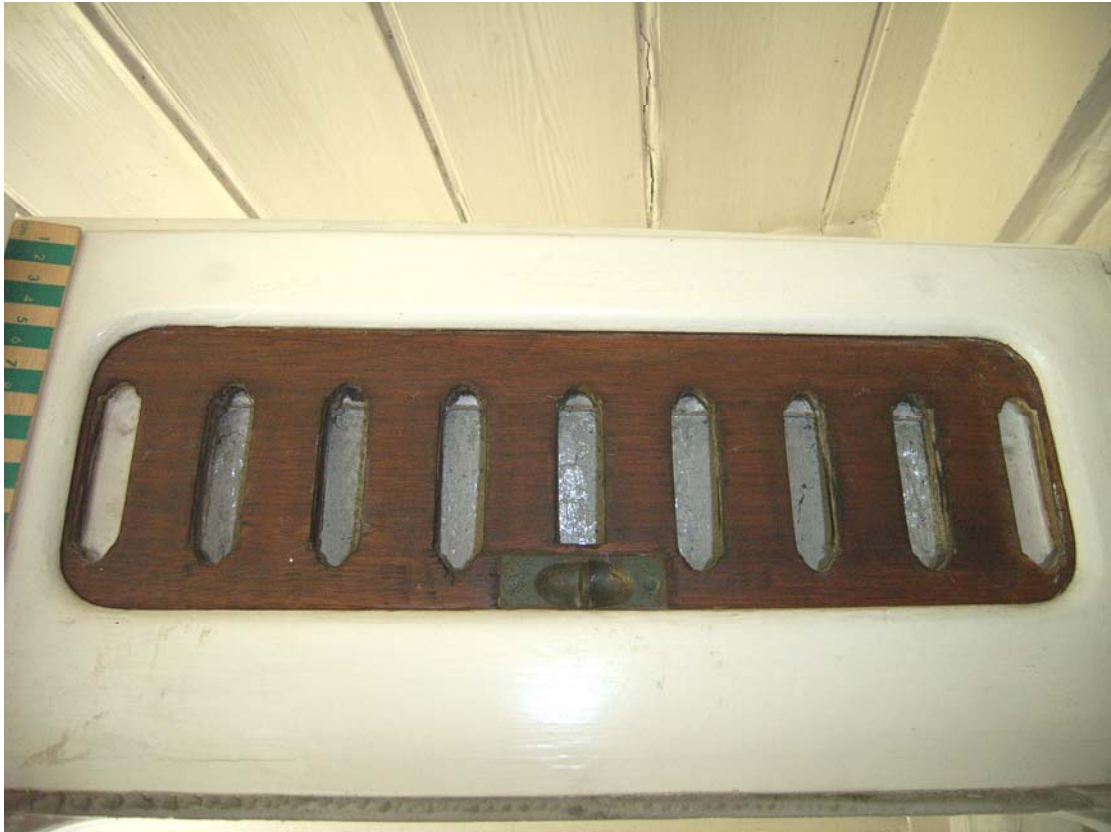
A2.7 Detail of wooden internal ventilator slat to door between bedroom (1) and veranda (4)
