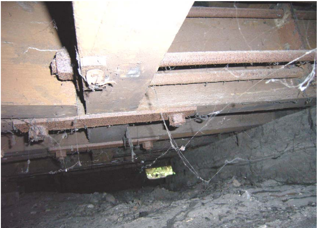
A2.12 Underside of carriage from west showing original floor structure resting on lateral sleepers
