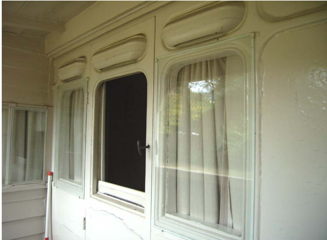
A2.5 Detail of carriage door and windows within southern veranda (4) – the door now opening into the bedroom (1).
