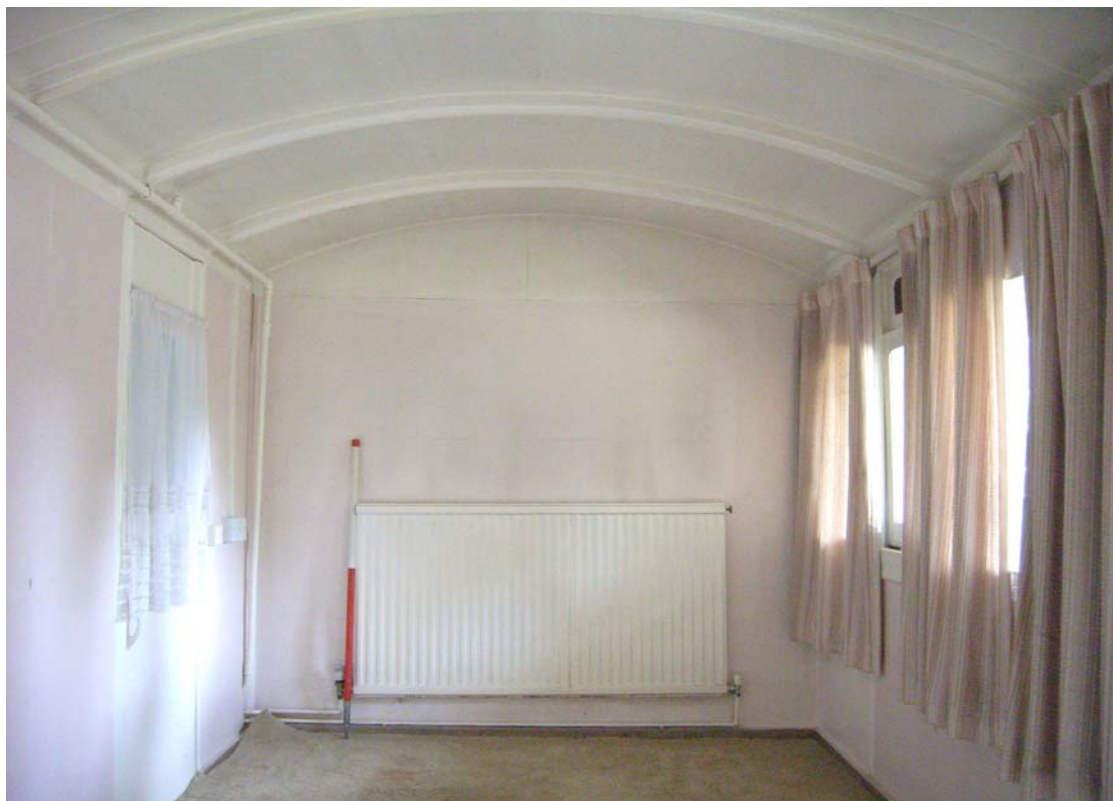
A2.10 Interior of bedroom (1) from north showing profile of carriage at southern gable and SMOKING window to right
