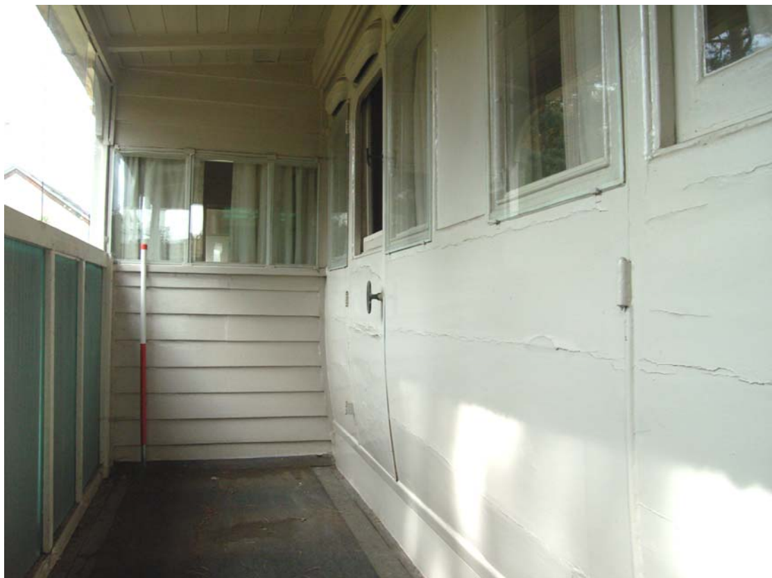
A2.4 Veranda (4) from south showing the external profile of the carriage to right. The original fabric appears to be concealed behind painted boarding
