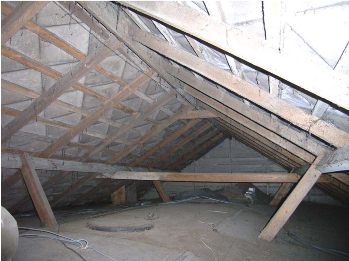
A2.11 Roof void from north showing curved oilcloth-covered carriage roof beneath later pitched roof
