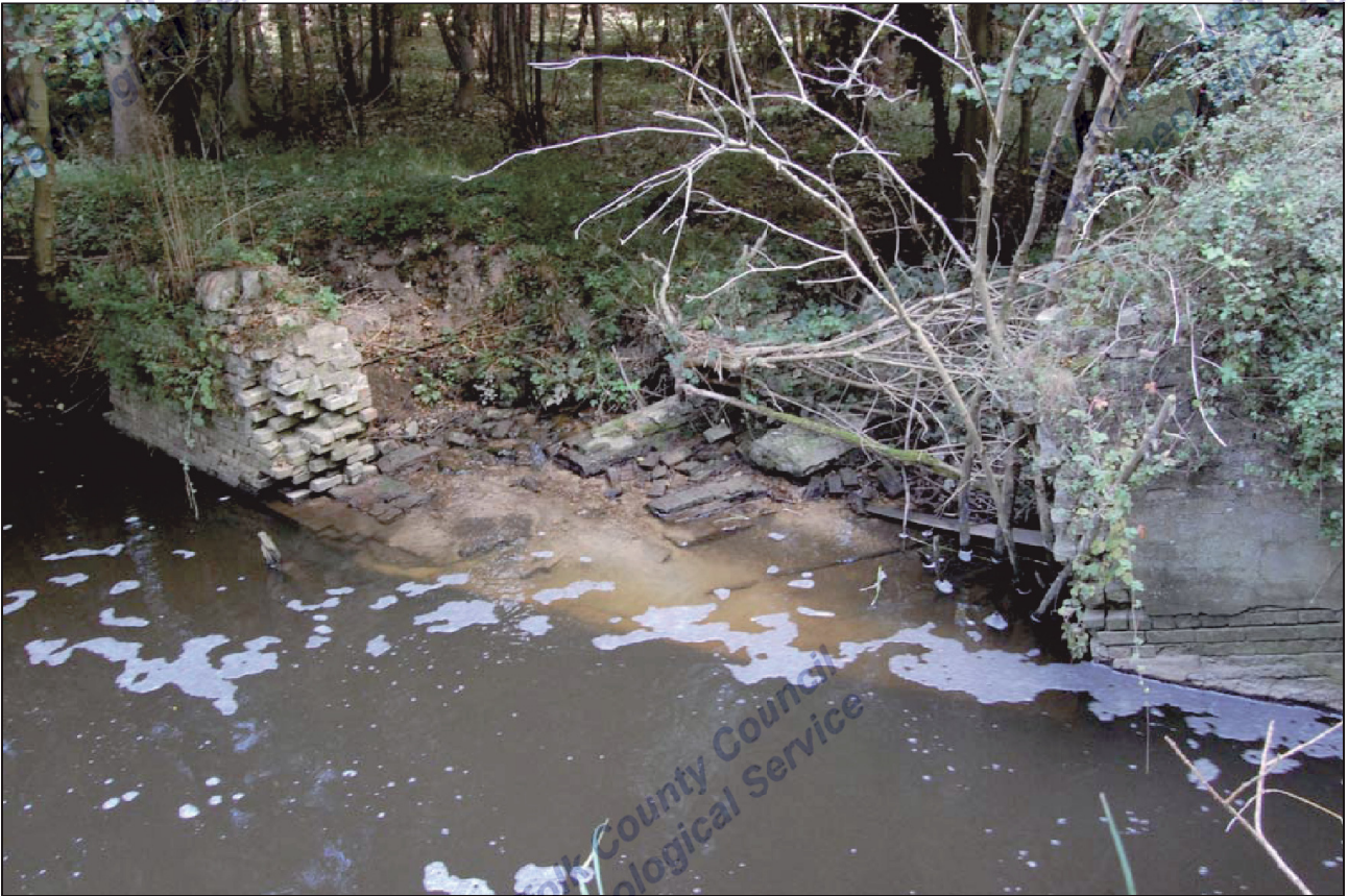
13. CUL 046, northern end, eastern wall damaged by secondary channel, looking NE
