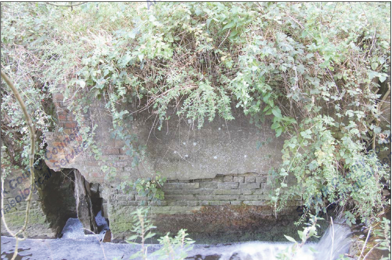
16. CUL 046, northern end, eastern wall, exposed reinforcing timber
