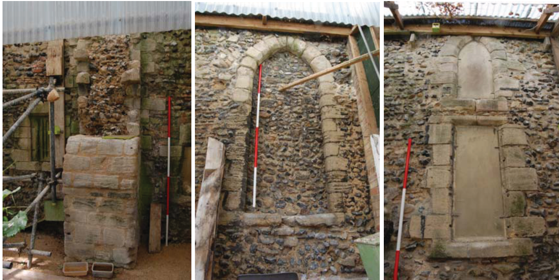
a b c South elevation buttress (a), window 0021(b) and window 0026(c)
