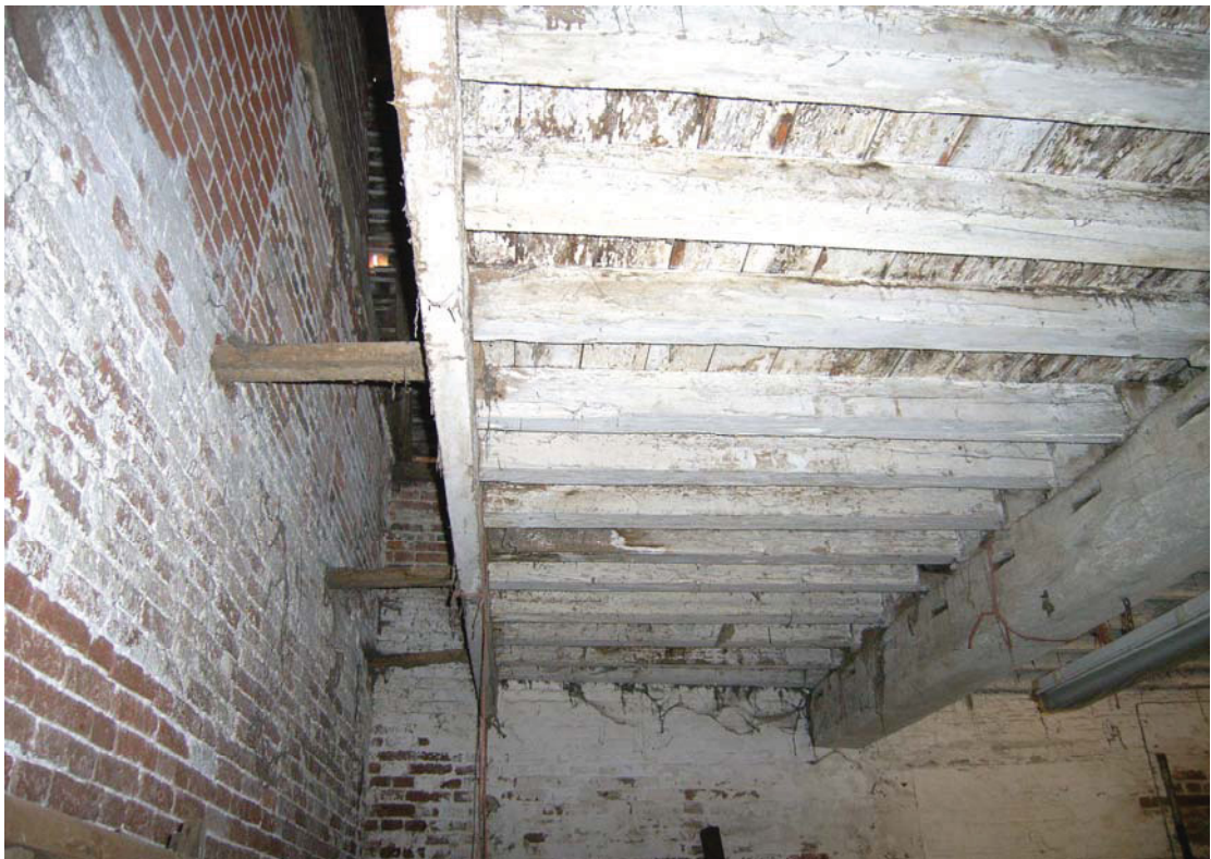
A2.6 The southern end of the original ceiling in the stable (B) seen from the east, showing the loading vent above the removed hay rack. Note the re-used binding joist to right.
