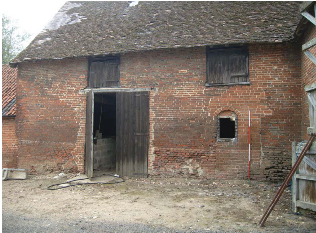
A2.3 Eastern façade of stable wing (B) showing blocked original door to right. The existing entrance is a recent insertion and the upper courses of brickwork which incorporate the hay loft hatches are also secondary
