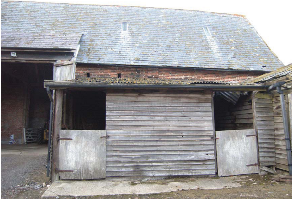
A2.11 Eastern half of barn's southern elevation above the 20 th century loose box (E) with two ventilation slits in the original brickwork to the left and secondary brickwork to the right where the barn abutted a demolished eastern wing
