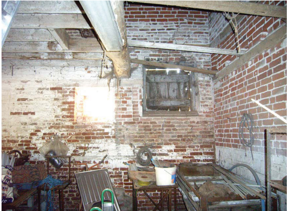
A2.7 The northern end of the stable's western internal elevation, showing the position of the removed chaff house with external loading hatch.
