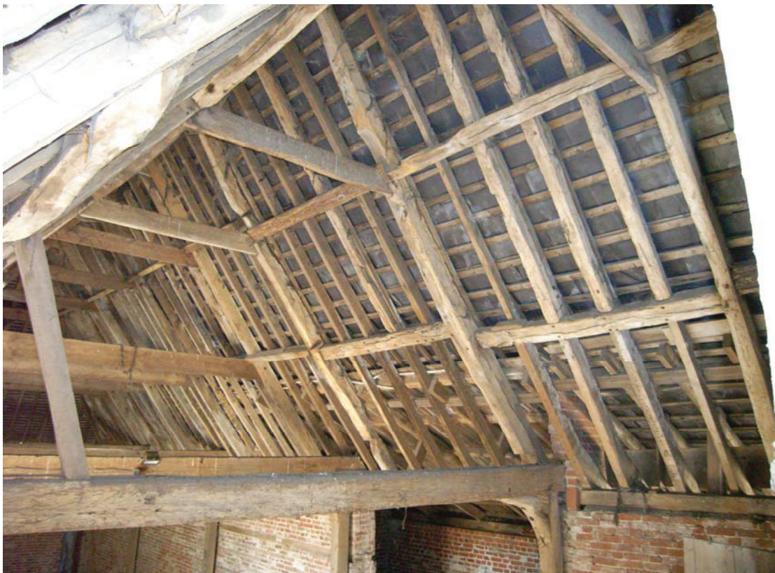
A2.10 Northern elevation of barn roof from south-east, showing the original structure of clapped and staggered butt-purlins to the right and the rebuilt 19 th century section to left.
