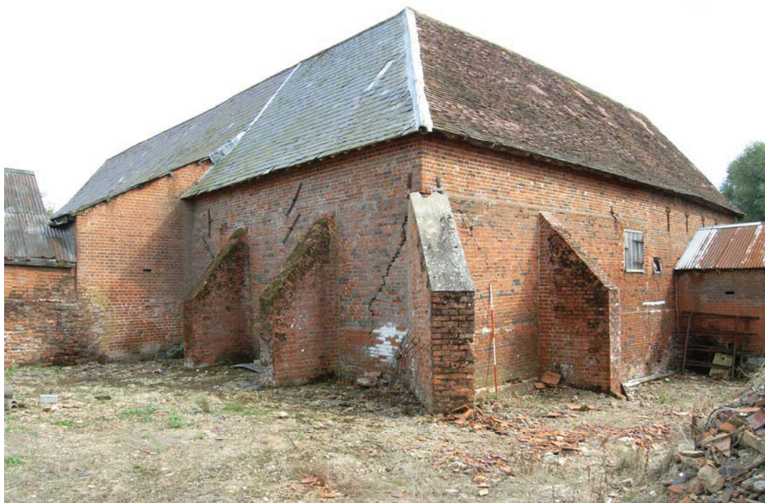
A2.4 The barn and the stable wing from the north-west, showing the slate roof of the barn to left and the peg-tiled stable to right. The buttresses are secondary, and the upper brick courses of the barn have been rebuilt along with both roof structures
