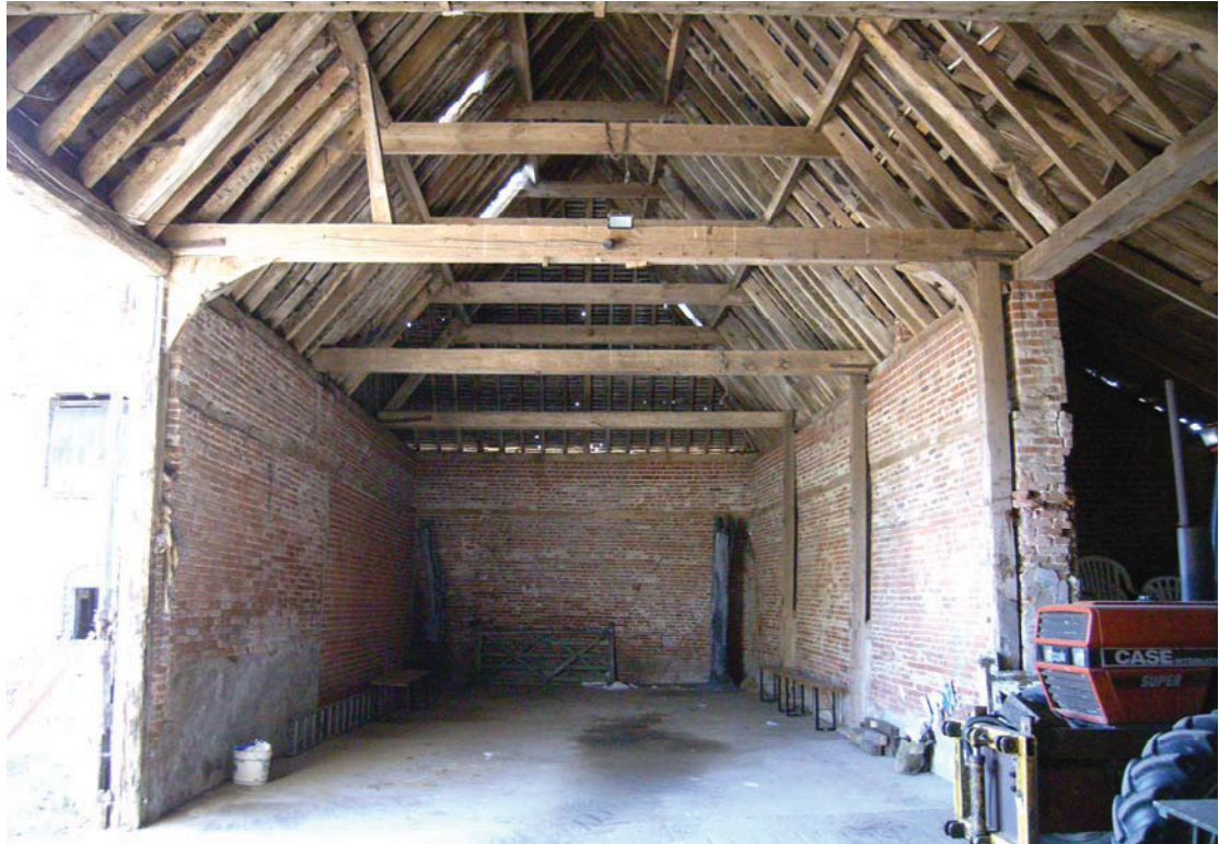
A2.8 Interior of barn from east, showing secondary lean-to porch to right and southern central entrance doors to left. The brickwork and roof structure at this end of the barn has been rebuilt above the timber rails set into the internal walls.
