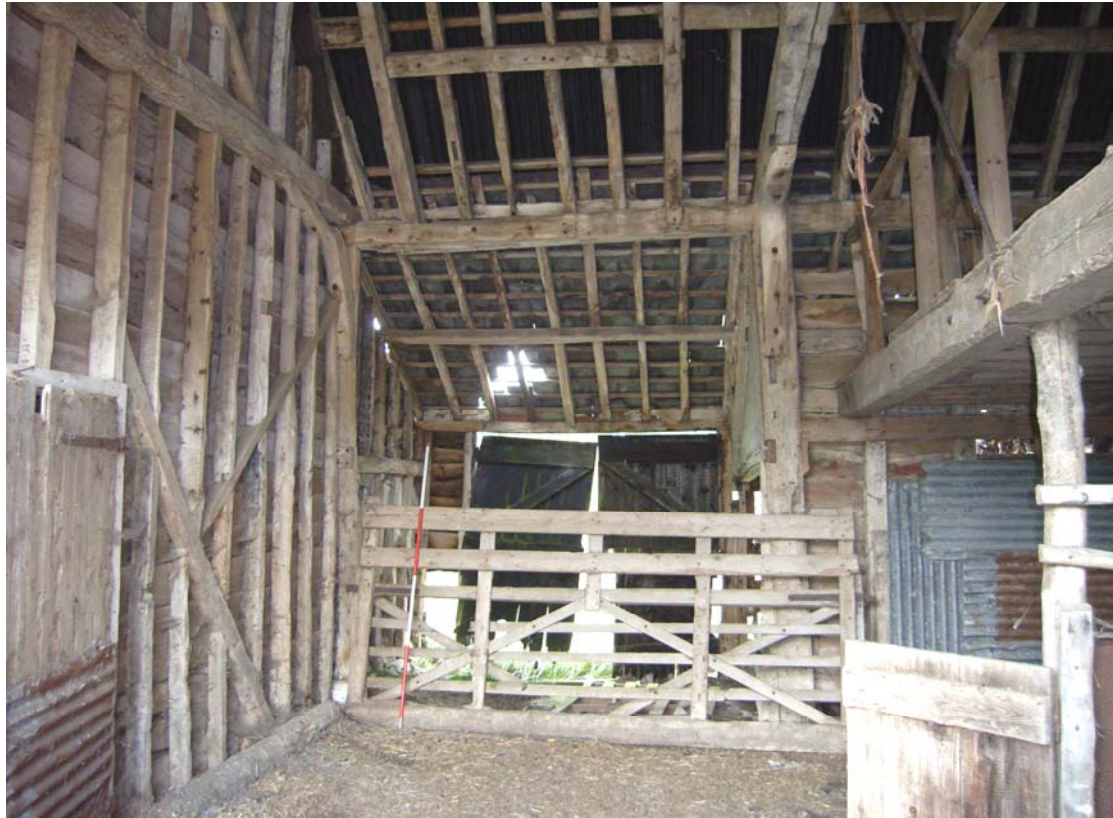
A2.7 Interior of 16 th century stable from east showing 20 th century loft and cattle stalls to right, entrance to lean-to porch (2b) in centre and 19 th century internal partition to left.
