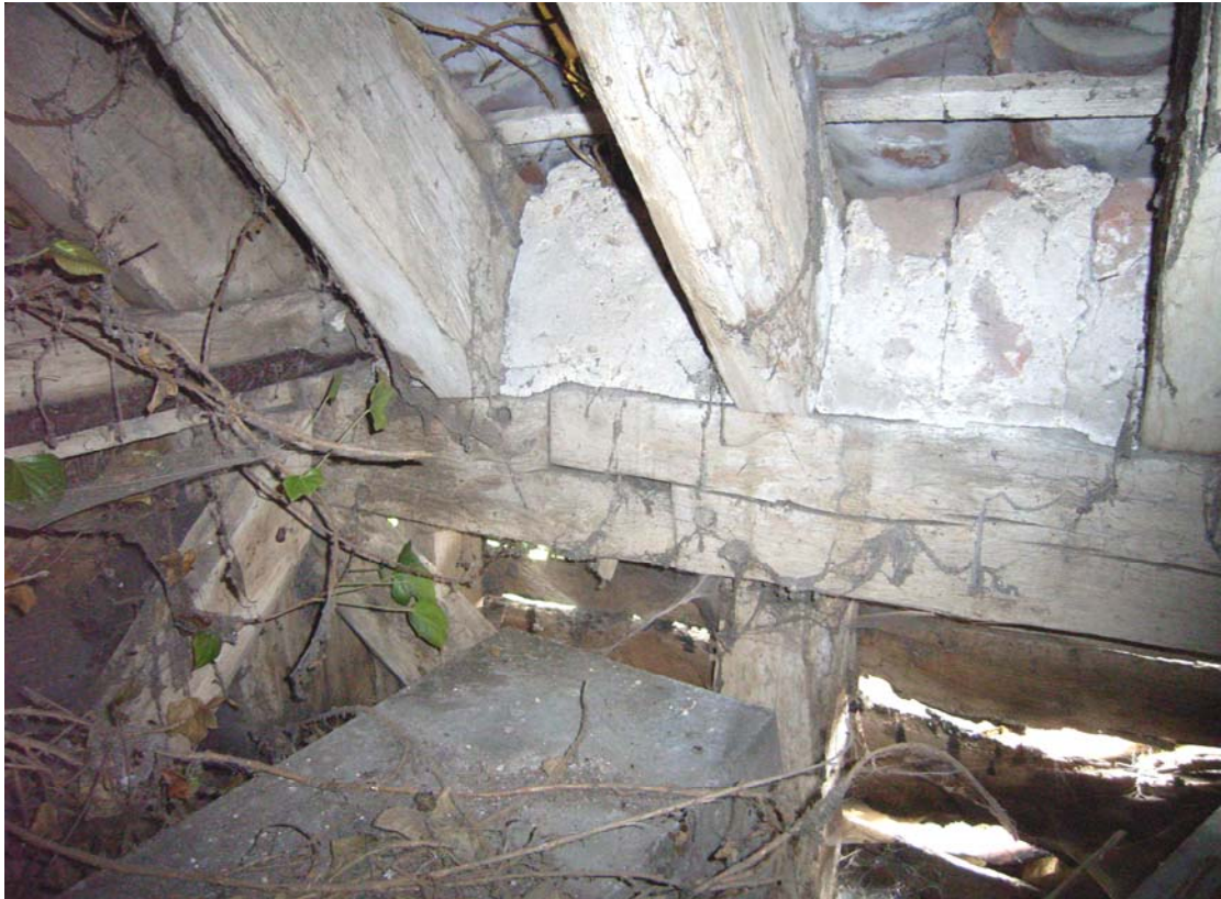
A2.11 Detail of short edge-halved and bridled scarf joint at northern end of eastern roof plate (1b), showing original door jamb and tie-beam of northern gable to left.
