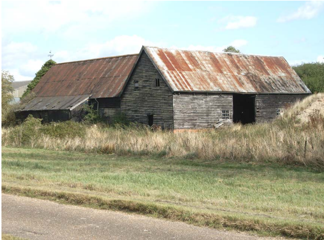
A2.3 Exterior of complex from south-west showing approach to hall in foreground, 19th century barn (3) to right & 16 th century stable range (1) & slate shed (2) to left
