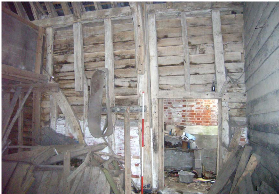
A2.10 Western internal elevation of 16 th century stable (1a) showing storey post C with framing of original door to right (now opening into 19 th century lean-to shed (2a)). The curved primary wall brace to the left is secondary.
