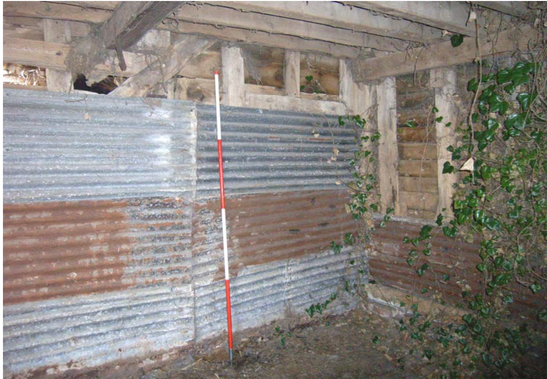
A2.9 Internal north-western corner of barn (1b) showing the intact jambs and lintel of an original door to the left of the corner post (E) and the intact jambs with mortises for a missing similar lintel in the northern gable to its right. Much of the original framing is hidden by boarding or corrugated iron as here.
