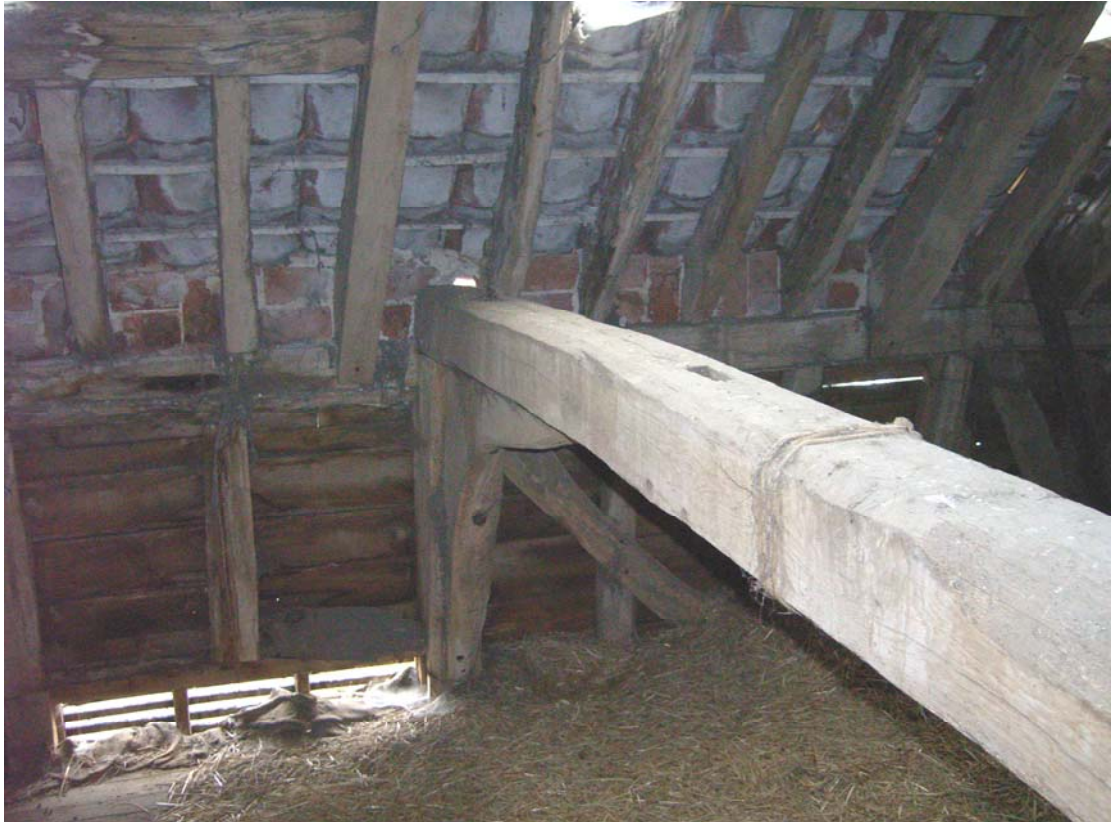
A2.12 Detail of tie-beam of open truss B-G from east, showing mortise of original queen-post or queen-strut in upper surface and bolted knee-brace replacing arch-brace.
