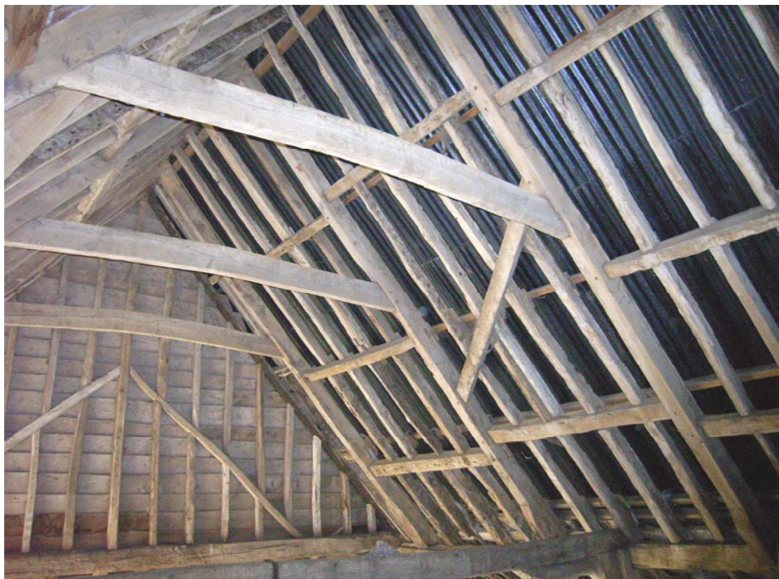
A2.8 Early-19 th century roof structure of staggered butt-purlins to former 16 th stable seen from northern bay and showing internal partition to southern compartment (1a) left.
