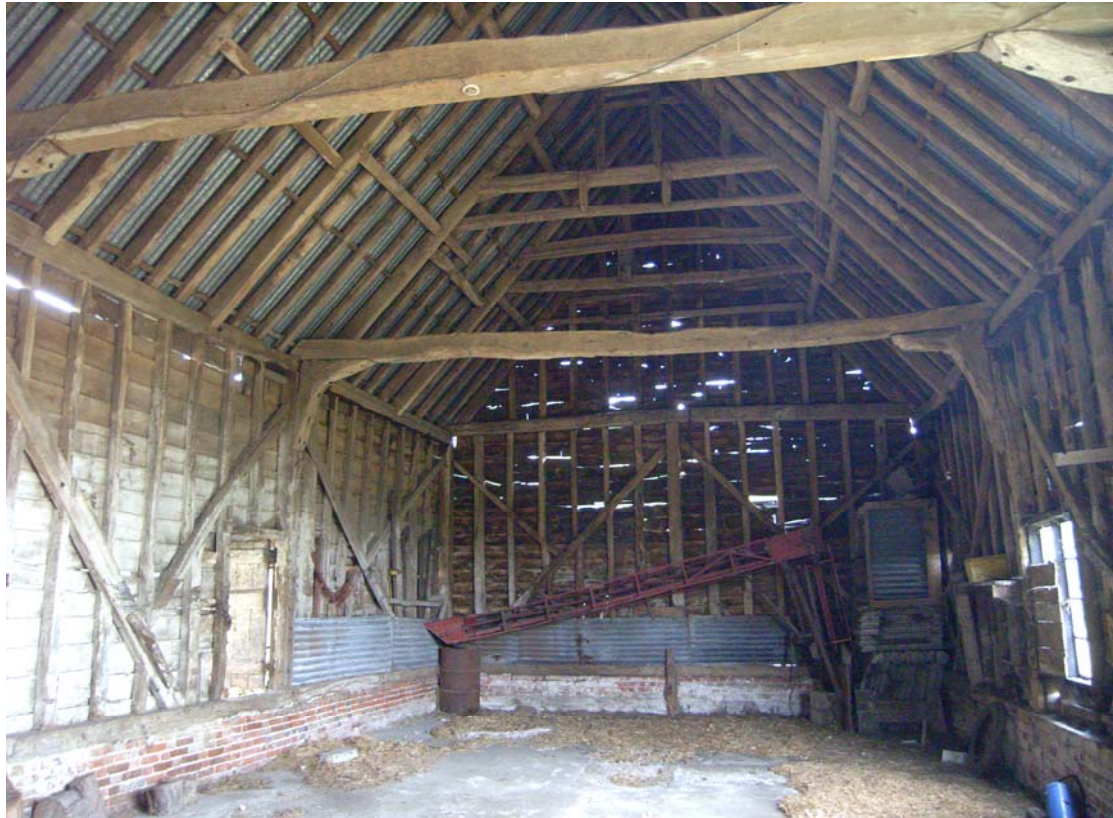
A2.5 Interior of 19 th century barn (3) from west showing original primary wall-bracing, bolted knee-braces to tie-beams and staggered butt-purlin roof structure
