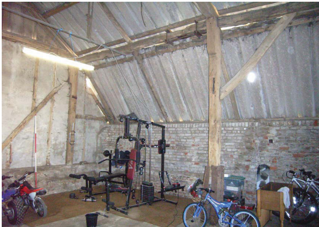
A2.6 North-west internal corner of barn showing the rebuilt rear (northern) aisle with the only original arcade brace to right
