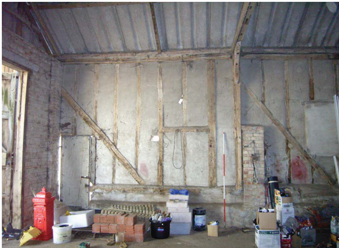
A2.8 Southern interior of eastern bay showing blocked stable door to right and later door to yard shelter to left.
