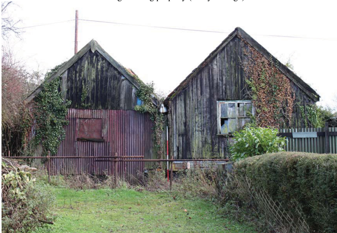
A2.3 External rear (western) gables showing the original cladding of vertical boards to shed 1 (right) and the roof gable of shed 2 (left). The secondary weatherboarding of shed 2 (which was originally open-sided) is hidden by corrugated iron.
