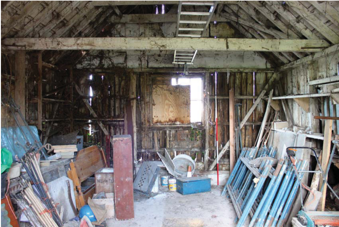
A2.4 Shed 1. General view of interior from east showing original wall fabric of horizontal rails with diagonal bracing to corners and external cladding of vertical boards. The framing of the two windows in both the northern and southern elevations is original, as is that of the central window shown here in the western gable, but the original glazing survives only to the north (right). Note the secondary shelving.
