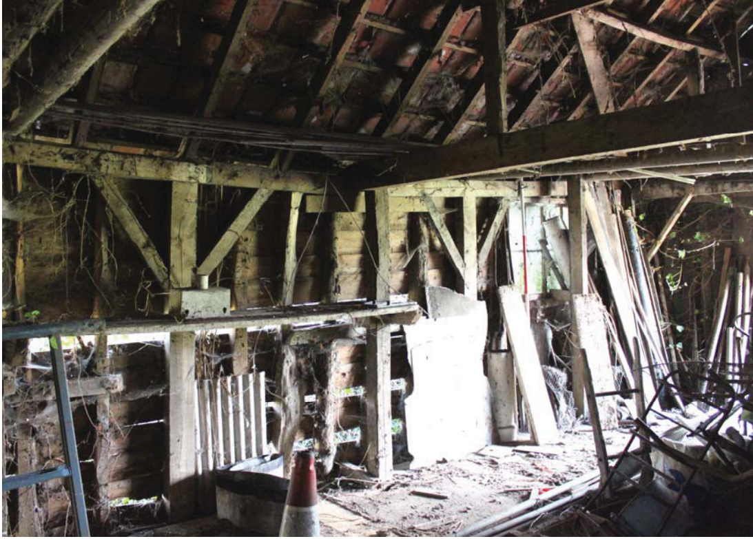
A2.12 Shed 2. Internal northern elevation from south-west, showing posts and braces or original open arcade with secondary outer weatherboarding.
