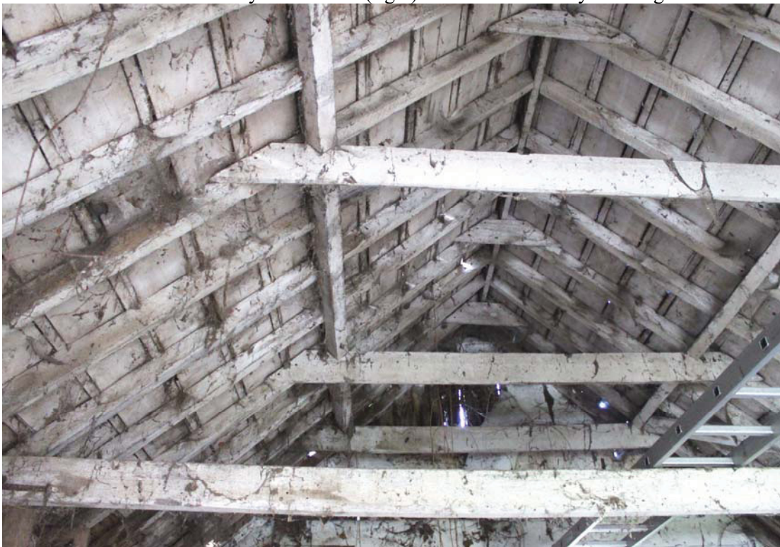
A2.5 Shed 1. The well-built clasped-purlin roof structure from the east, showing original rafters with boards between the tile battens.
