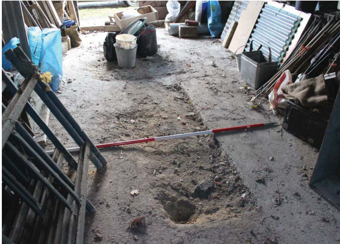
A2.8 Shed 1. Concrete floor from west showing area of collapse possibly caused by infilled saw pit.
