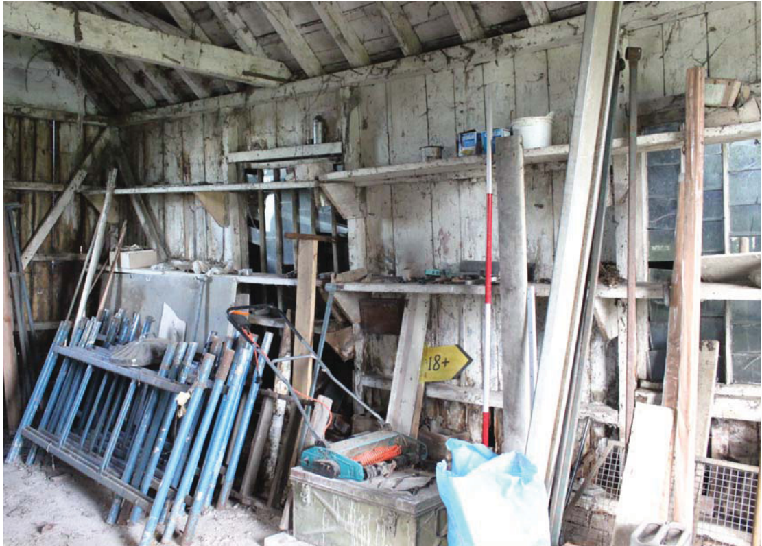
A2.6 Shed 1. Internal northern elevation seen from the south-east, showing two windows with original glazing now blocked by secondary shelving.
