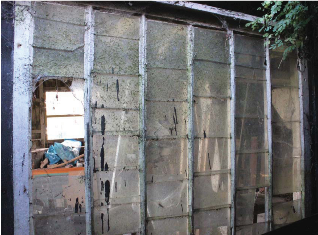
A2.10 Shed 1. Detail of original lapped glazing to eastern window of northern wall (seen from shed 2).
