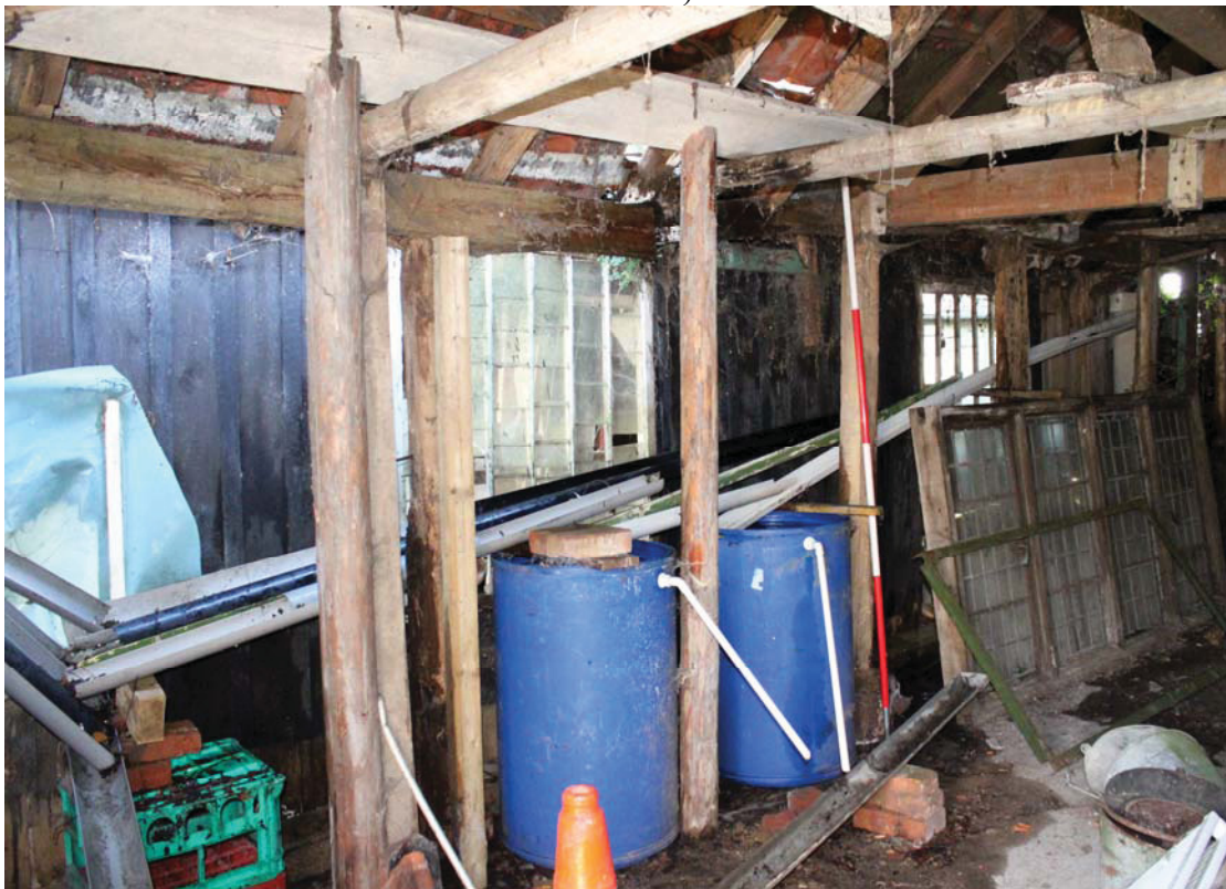
A2.11 Shed 2. Interior of open southern elevation from north-east showing original northern exterior of shed 1.
