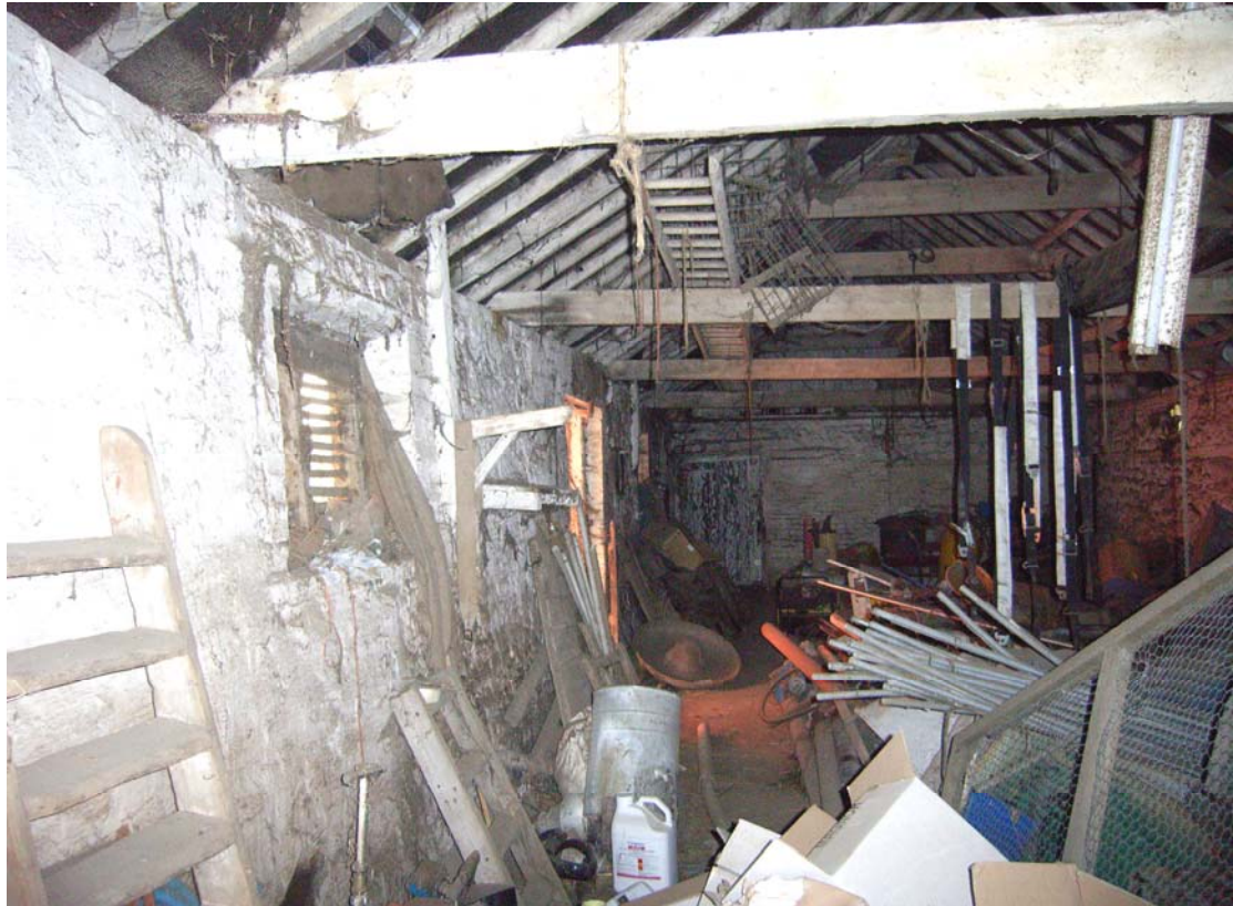
A2.11 Stable (8). Interior from south showing harness hooks, yard door and louvered windows to left. The door in the rear (northern) gable opens into a tack room in the corner of the western barn (1).
