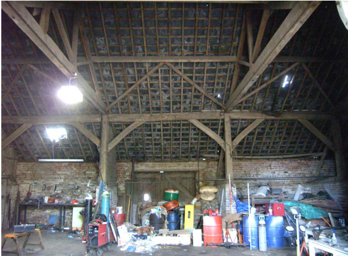
A2.5 Western Barn (1). Interior of the aisled southern elevation showing central door to yard. The tie-beams and roof structure are late-19 th century replacements and the storey posts contain mortises for arch-braces as in the eastern barn (3).
