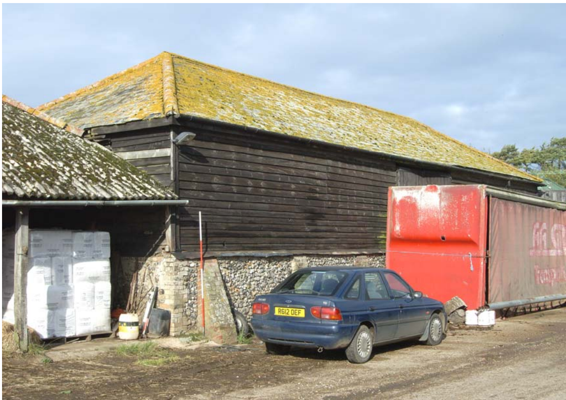
A2.6 Eastern Barn (3). Exterior from south-east showing slate roof, hipped gables & tall flint plinth.
