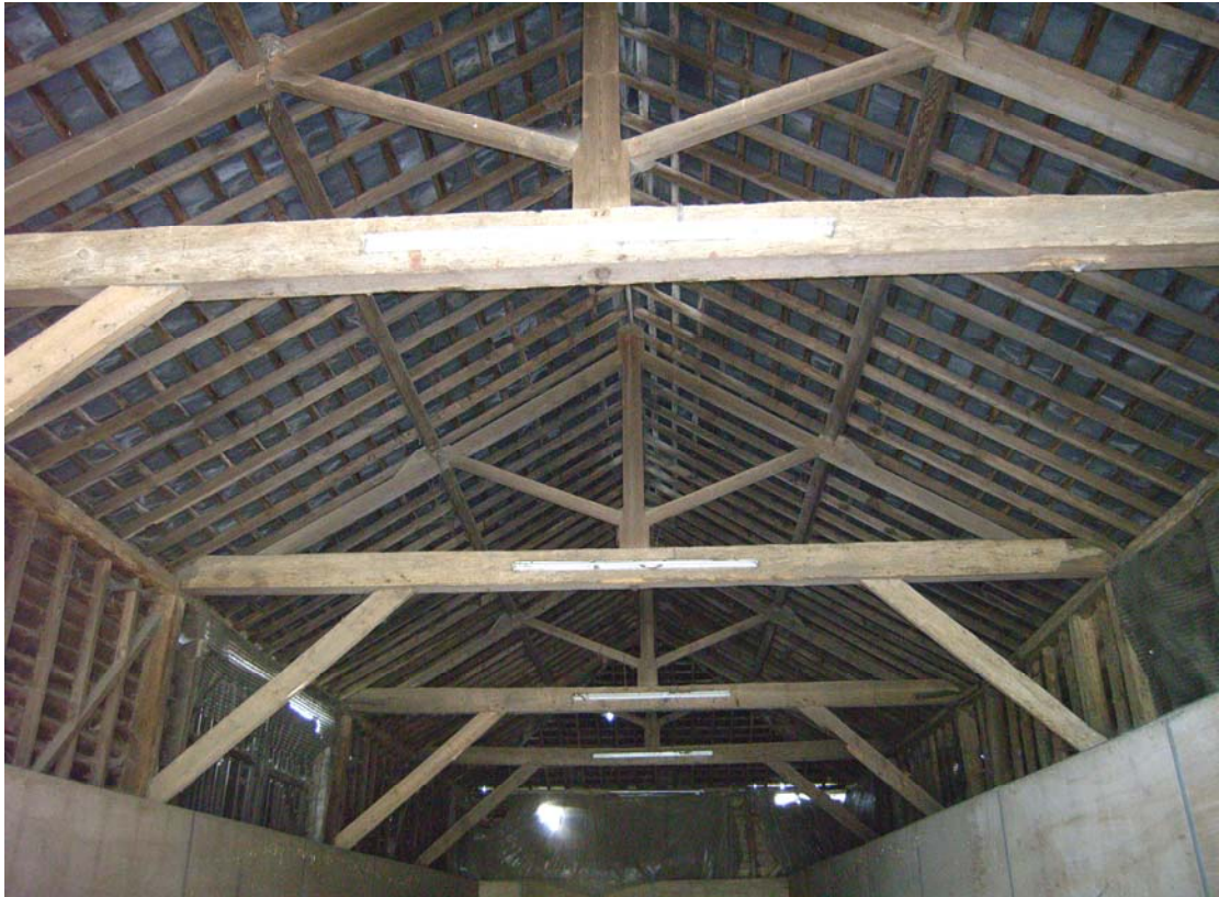
A2.7 Eastern Barn (3). Original roof structure seen from northern gable showing king-post trusses with intact braces to tie-beams.
