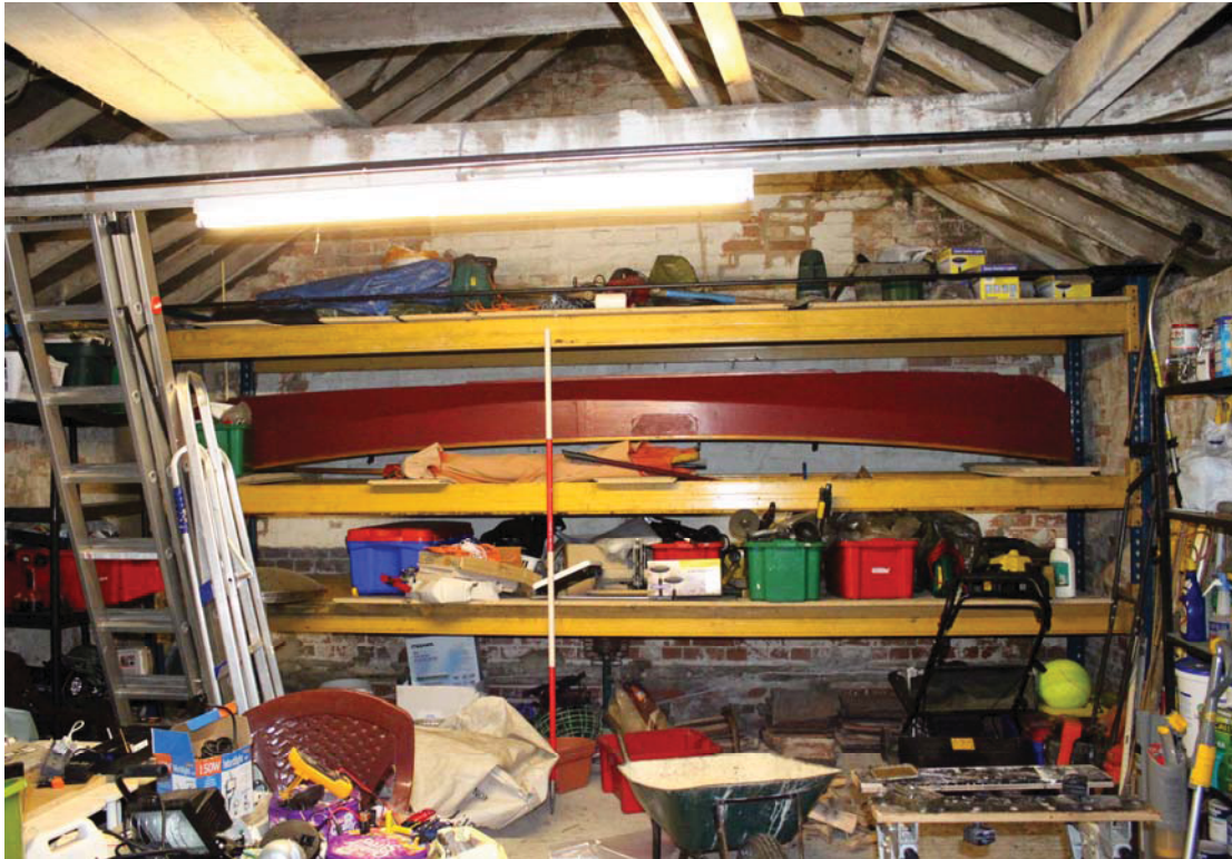
A2.7 Interior from south showing the northern gable and the shed's current purpose as a general storage 'garage' with metal shelving against its walls. Note the original whitewashed tie-beam spanning the shed's width, with horizontal axial and diagonal braces to the south.
