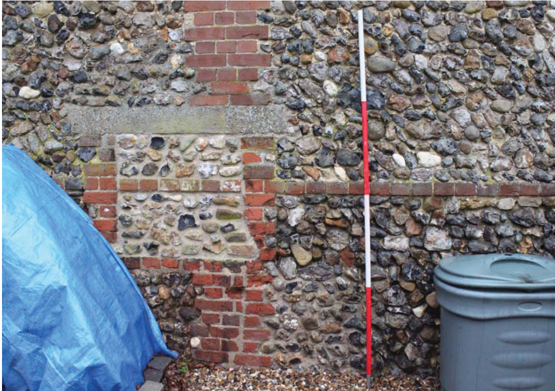
A2.6 Detail of blocked secondary door with stone or concrete lintel in centre of eastern external elevation. This probably formed a feed hatch onto the cattle yard, but was subsequently converted into a window. It interrupts the original red-brick dressing above
