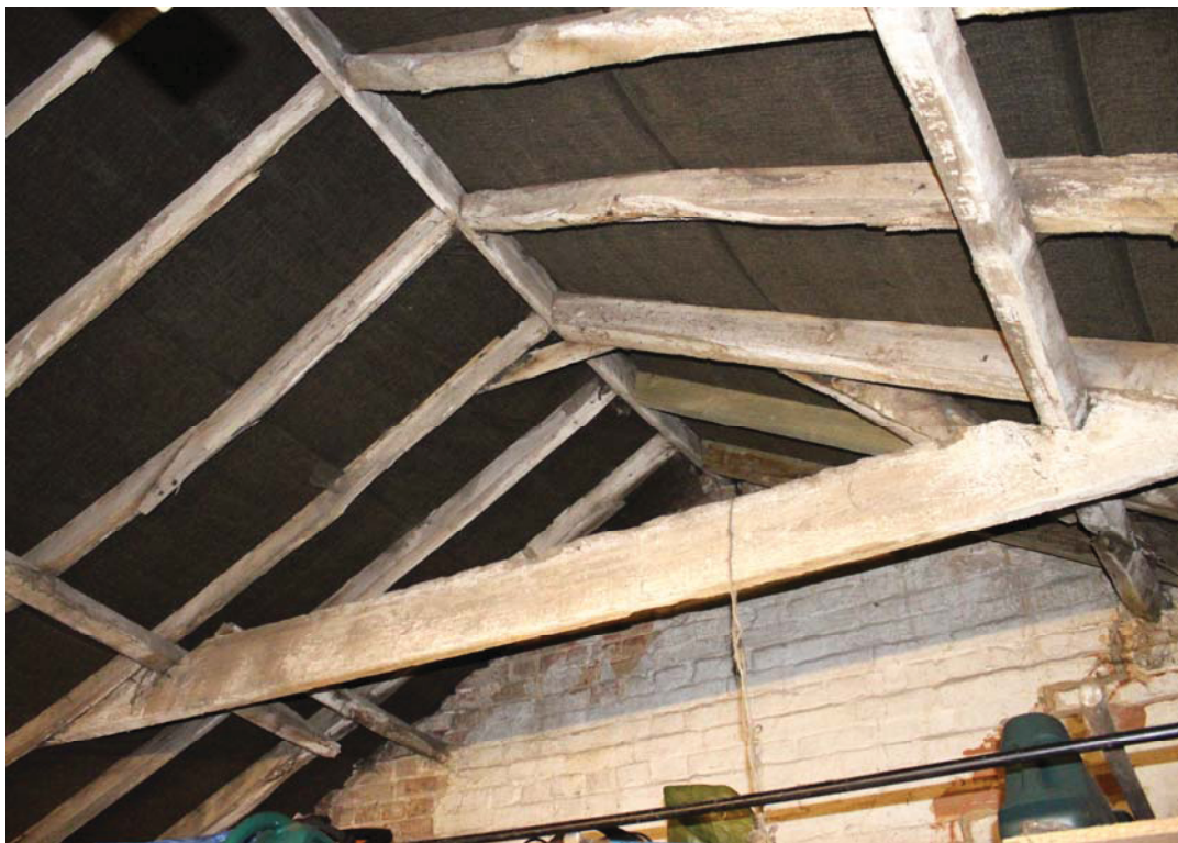
A2.10 Original roof structure from south showing clasped purlins with nailed collar and ridge-board. The rafters vary in size and several show evidence of re-use from earlier structures.
