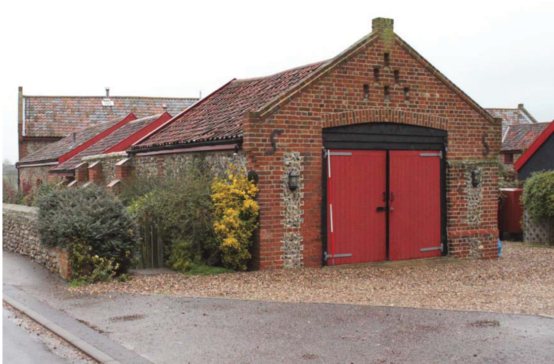
A2.3 Exterior from Duff's Hill to south showing double doors and blocked ventilation holes of southern gable with main barn in rear to left. The doors and much of the brickwork was renewed in 2000
