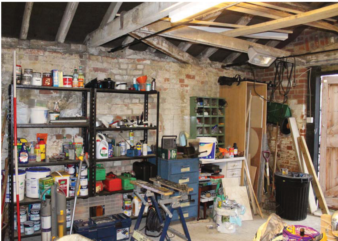
A2.8 Internal eastern elevation showing southern gable to right with original horizontal braces to tie-beam. The inserted eastern aperture to the left is obscured by shelving.
