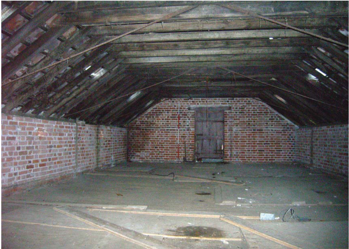
A2.9 Granary 2. Upper granary floor looking to southern gable from internal partition showing vertical scars of removed grain bins to left and right
