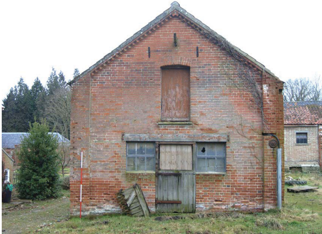
A2.7 Granary 2. External southern gable showing original loading door to first-floor granary above blocked wide aperture on lower storey
