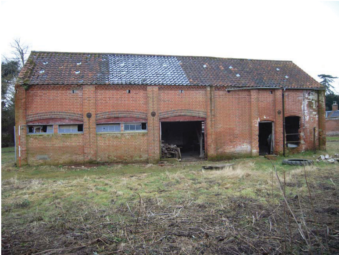
A2.6 Granary 2. External eastern elevation showing former open arcade to left & enclosed with external door and enlarged northern window to right
