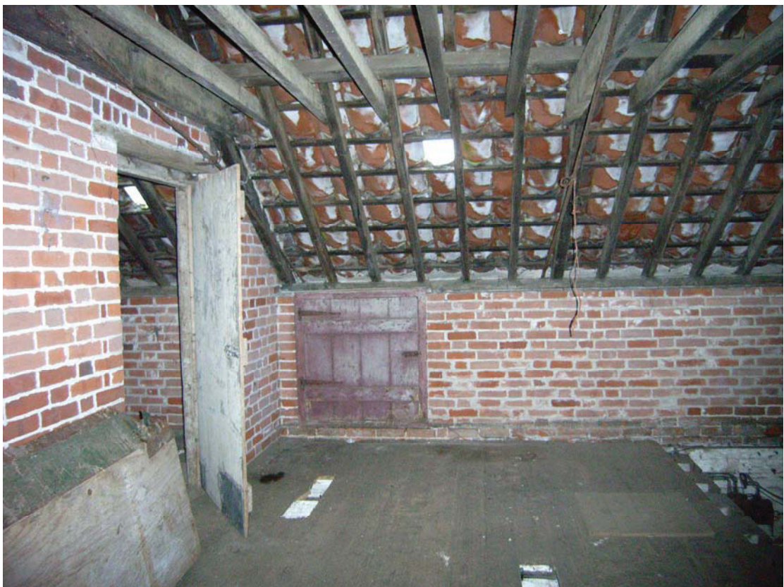
A2.10 Granary 2. Internal western elevation of northern first-floor granary compartment showing original external loading door to right and door to southern compartment to left
