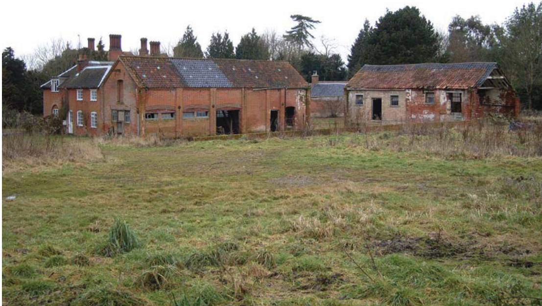
A2.1 General view from south-east showing shed 1 to right and granary 2 to left with chimneys of Hurts Hall in rear
