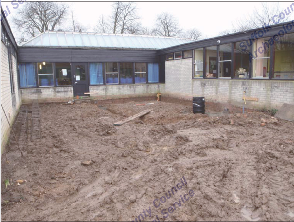
Plate 1. Stripped area at the rear centre of the school, showing the deeper footings section, facing SE
