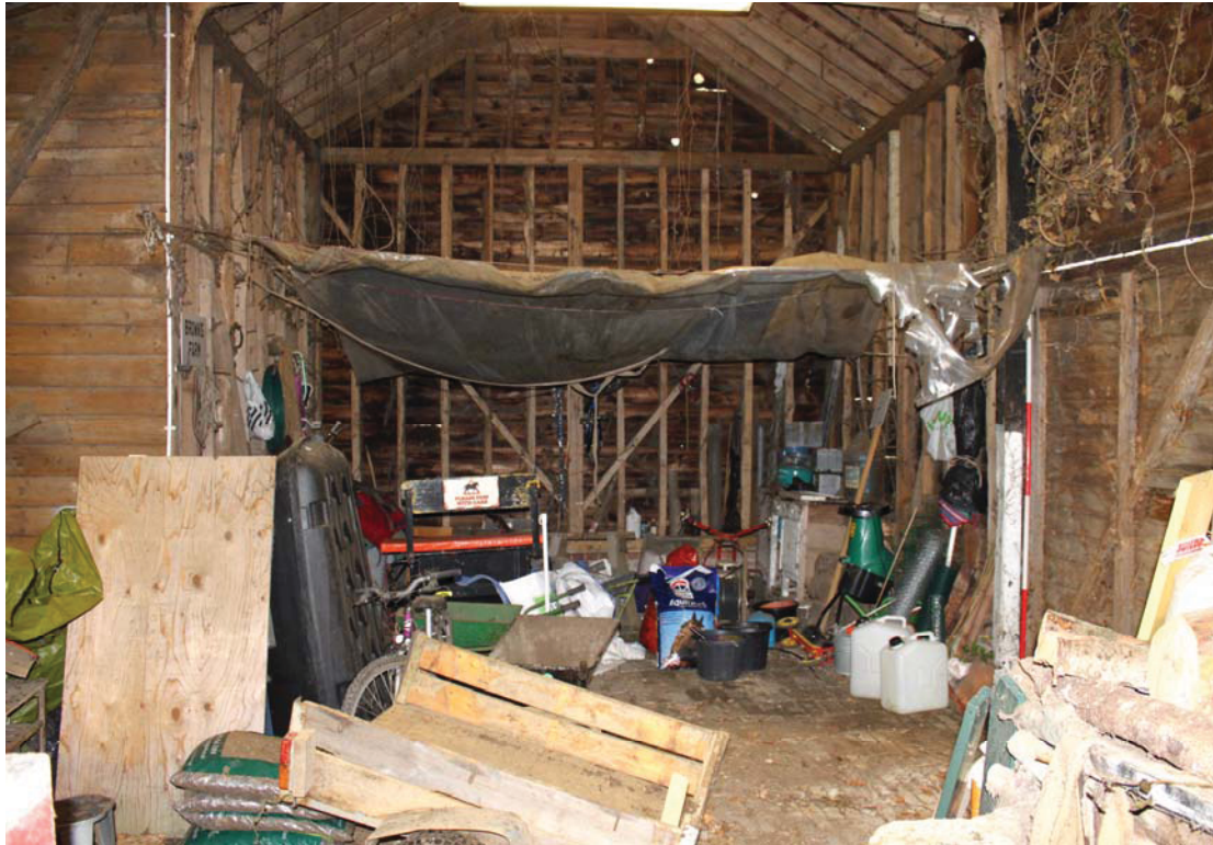
A2.5 Interior of barn (A) from east showing narrow softwood studs with nailed diagonal bracing. The central entrance bay and brick threshing floor lies in the foreground with the lean-to porch (B) to left and northern door to right.
