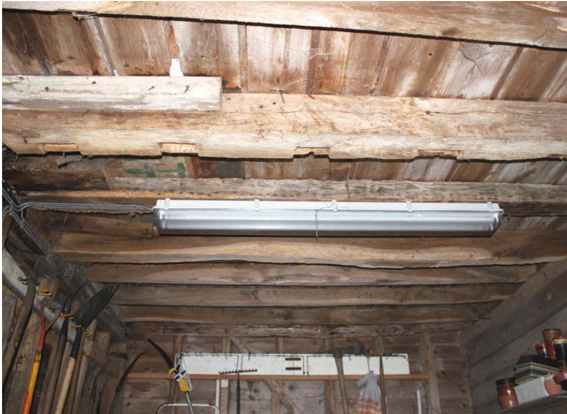
A2.7 Detail from north of re-used ceiling joists in vehicle shed (C). These substantial hardwood timbers were necessary to support the weight of the granary above.
