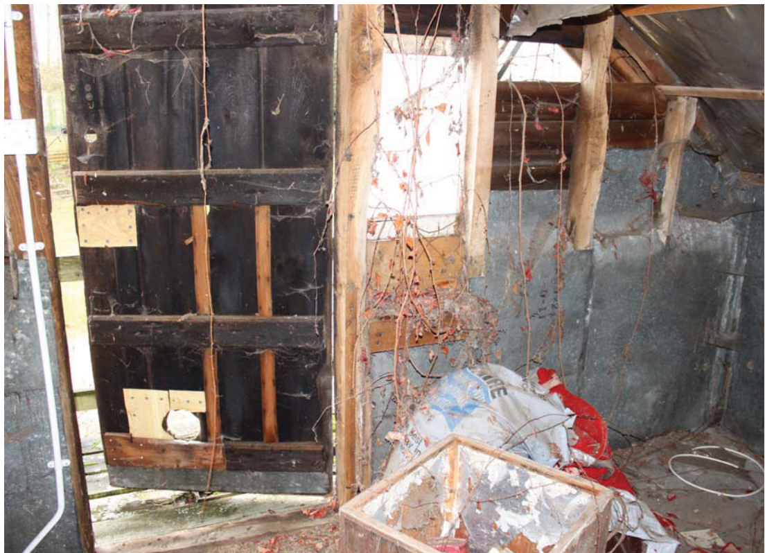
A2.8 Internal eastern gable of first-floor granary above vehicle shed (C) showing cat hole at base of door and 20 th century zinc lining.
