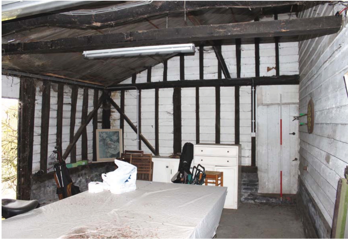
A2.9 Interior of south-eastern shed (E) from west showing external southern entrance to left and door to barn porch to right.
