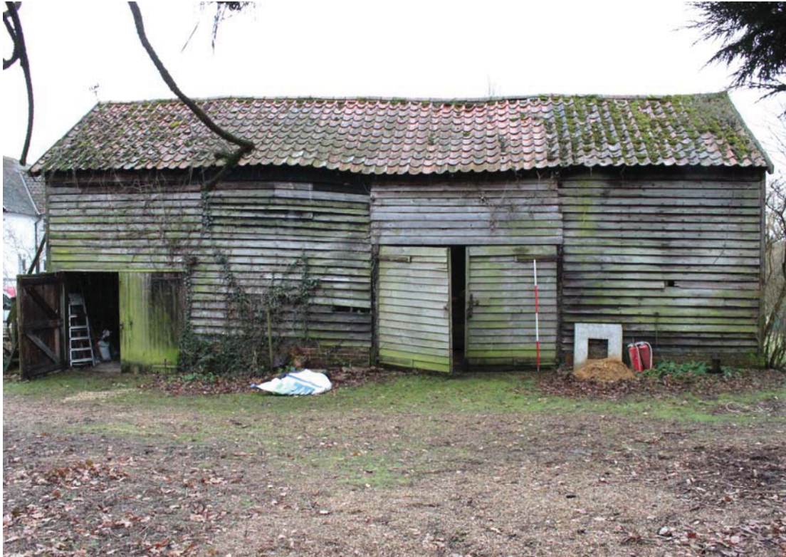
A2.3 Northern external elevation showing doors to vehicle shed (C) left & barn doors in centre. The latter have been reduced in height.
