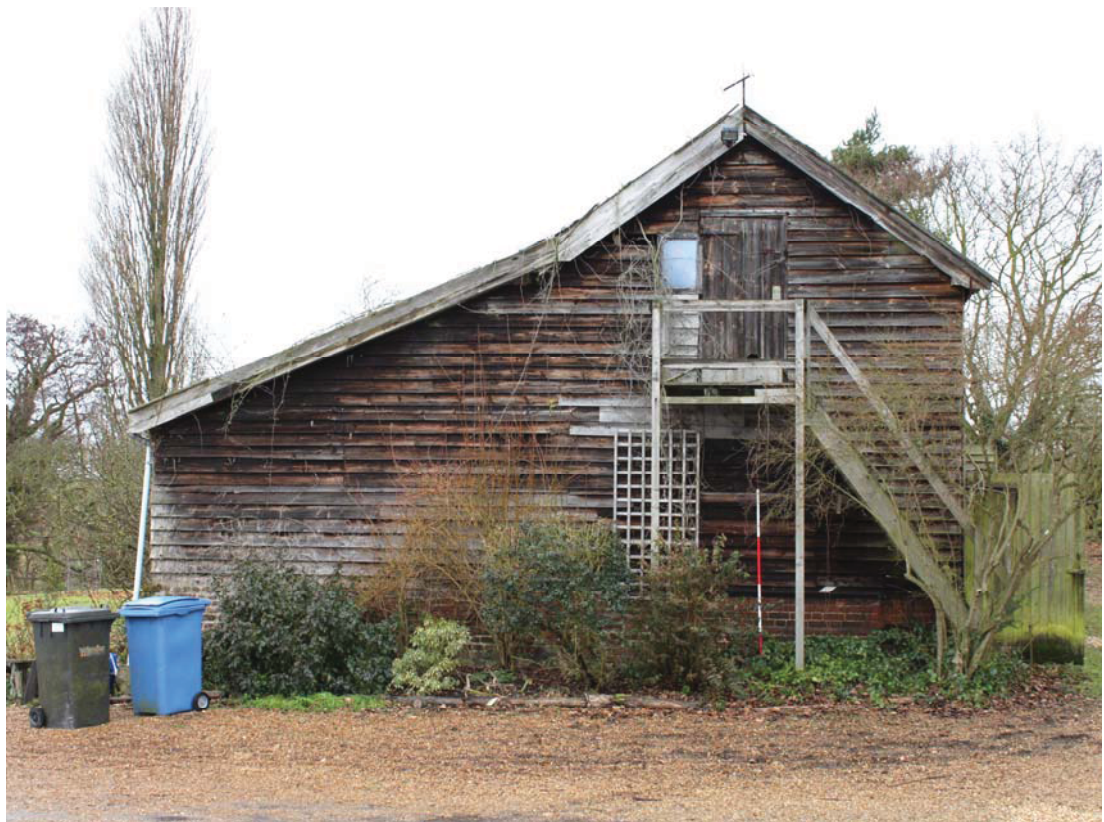
A2.4 Exterior of eastern gable showing external stair to granary above vehicle shed (C) (the stair renewed in the late-20 th century) and the profile of the contemporary southern lean-to sheds to left.
