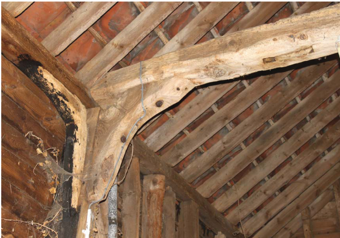
A2.6 Detail of original bolted knee-braces and re-used tie-beam in north-eastern corner of entrance bay. The empty arch-brace mortise in the underside of the tie-beam is shown to right
