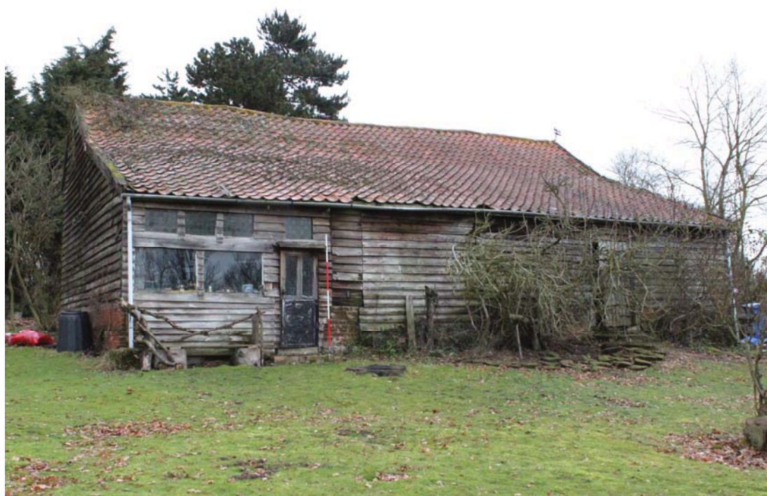
A2.2 Exterior of barn from south-west showing 20 th century glazing of lean-to cow-shed (D) to left, blocked doors to lean-to porch (B) in centre and double-hung doors to eastern shed (E) to right. A shelter shed and cattle yards have been demolished from the foreground.
