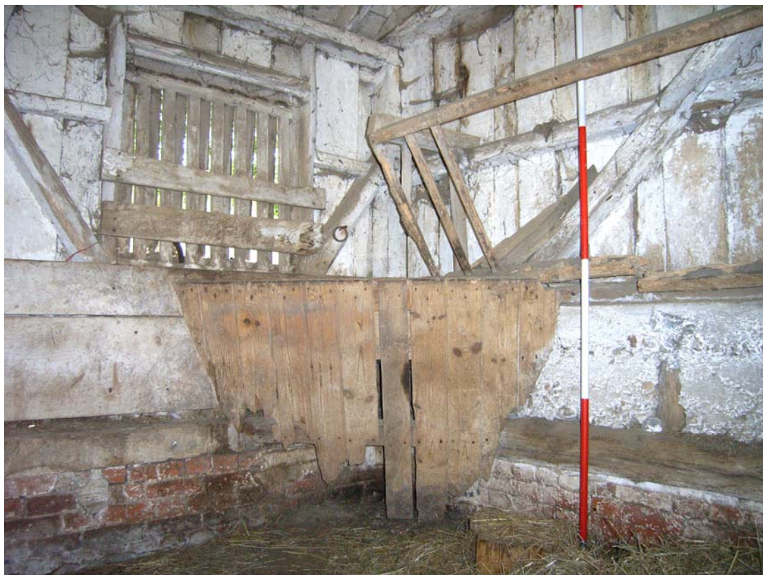
A2.10 Roadside stable (5a). Detail of boarded manger in south-western internal corner with low hay rack to right and slatted window to left.
