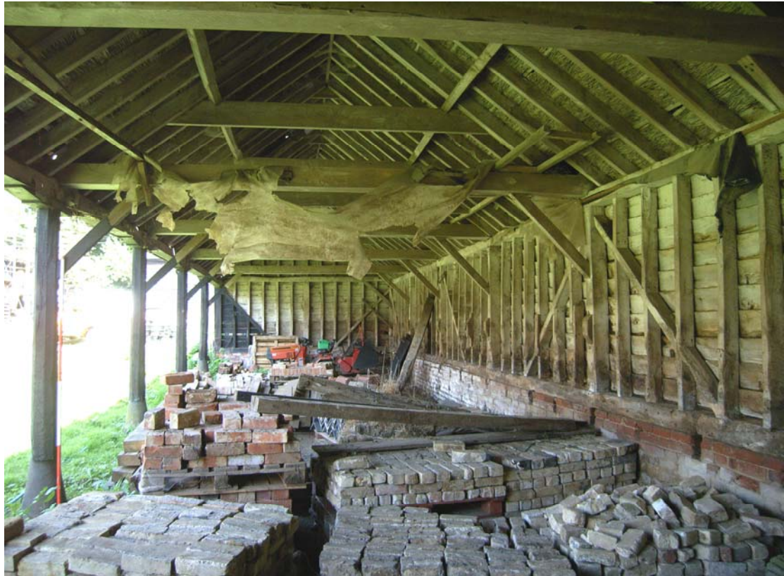
A2.11 Roadside shelter shed (6). Interior from west showing wall framing with octagonal arcade posts abutting central yard to left.
