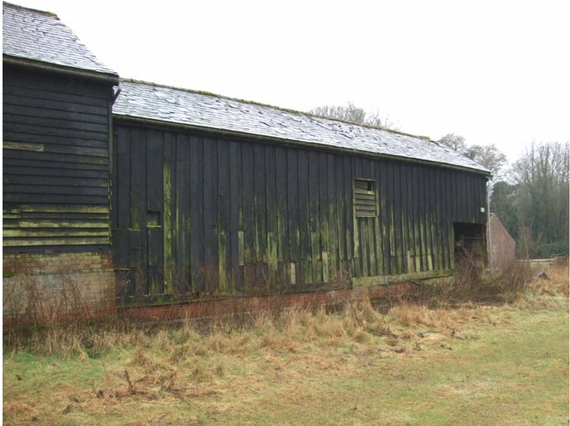
A2.13 Jan 2009. Northern external elevation of stable (2) showing vertical boarding with barn (1) to left.
