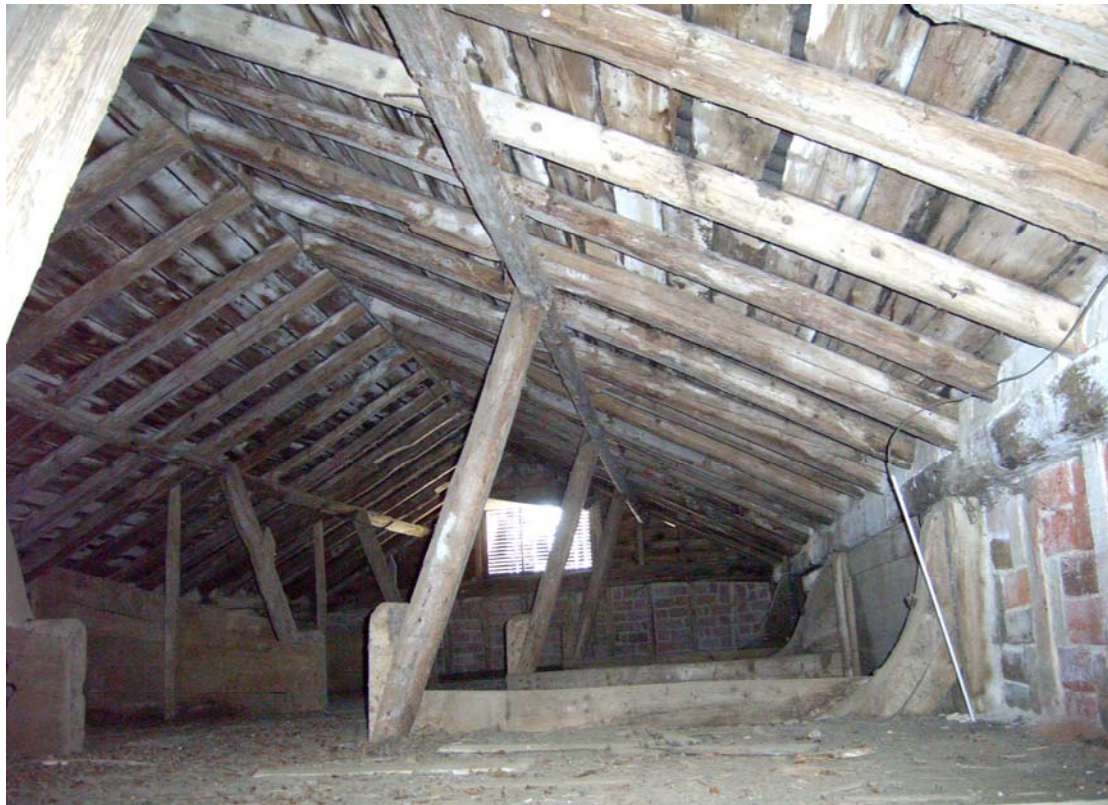
A2.9 Cart Lodge (4). Interior of first-floor granary showing remains of grain bins with axial passage to left
