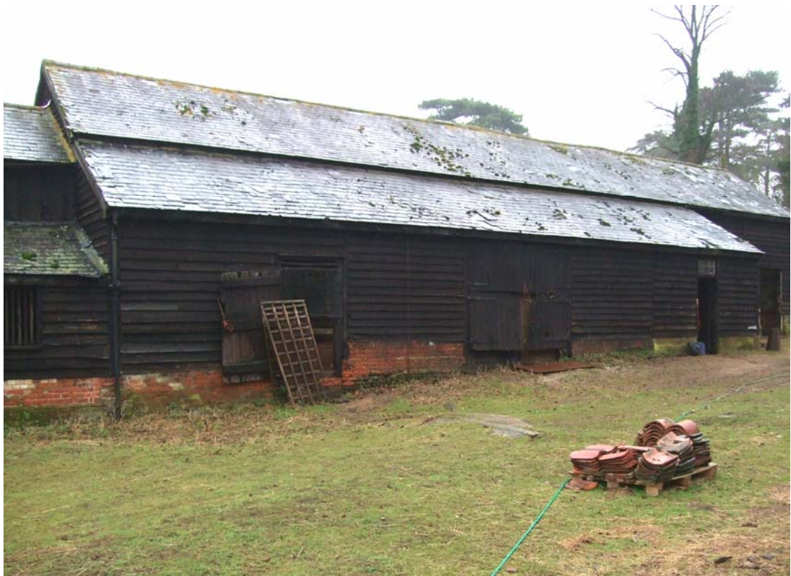
A2.14 Jan 2009. Southern external elevation of barn (1) showing lean-to porch and sheds adjoining central yard with stable and lean-to tack room (2) to left and granary (3) to right.
