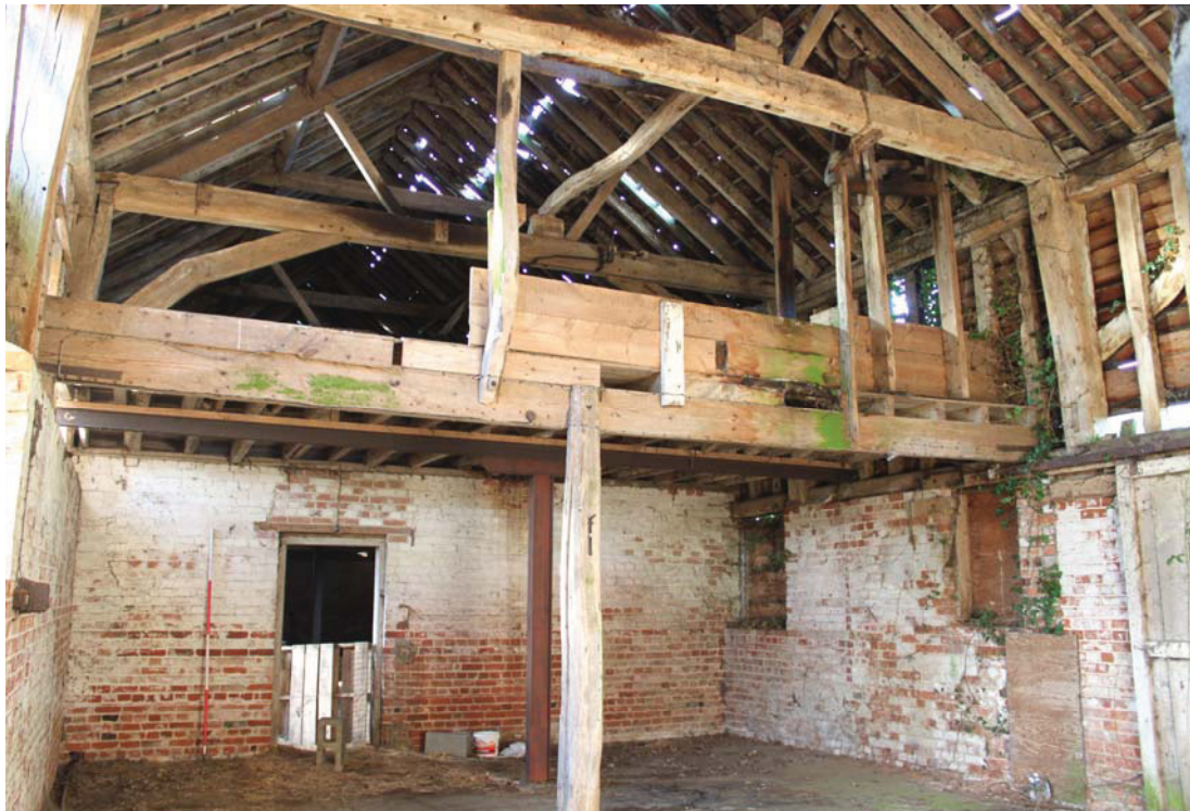
A2.6 Interior of central section of barn (1b) from east showing the 19 th century grain floor which extends above the stable (1a) to the western gable. The tie-beam contains 12 empty stud mortises for the original partition dividing the three-bay barn from the four-bay barn.
