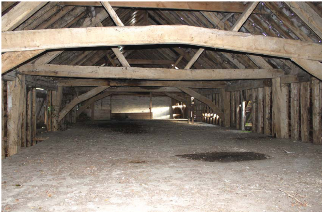
A2.8 Interior from west of the grain floor/hay loft above the 19 th century stable, showing the original tie-beams and cranked arch-braces beneath the 19 th century roof structure. The loading vent above the former hay rack is visible to the left, spanned by 'bridges' in front of each external loading doors in the northern elevation. Note the cambered tie-beam of the original hay loft in the foreground and the horizontal barn tie-beams in the rear.
