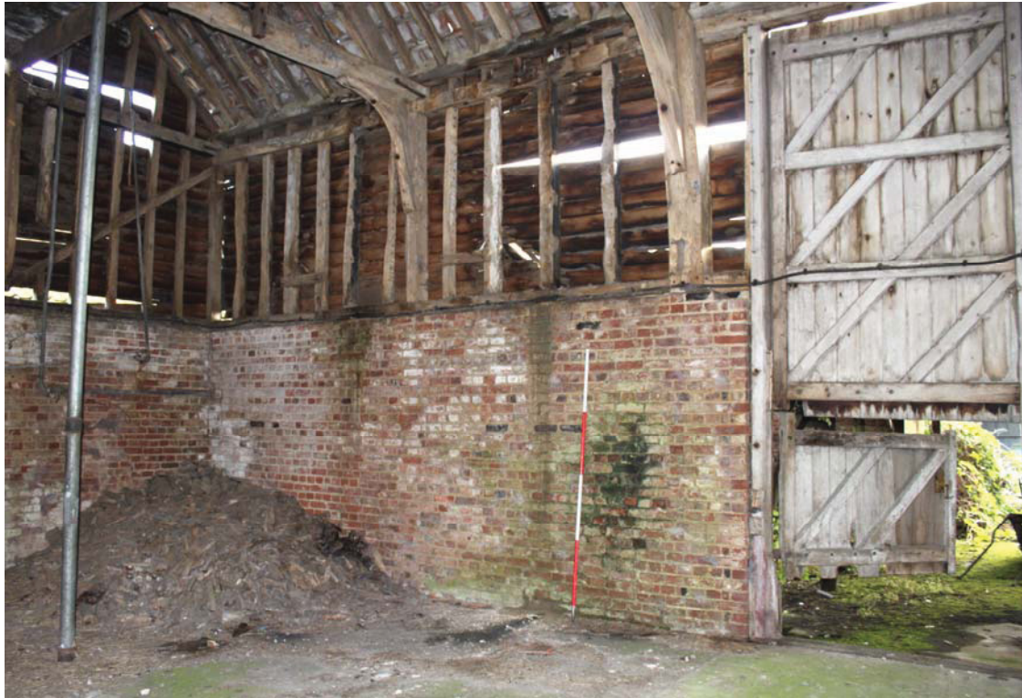
A2.5 Interior of barn showing the south-eastern corner of its eastern section (1c) with the two 19 th century bays to left & the 19 th century barn doors in the original end-bay (J) to right. The storey post and tie-beam to the left of the doors contain the 14 empty stud mortises of the late-16 th century barn's eastern gable.
