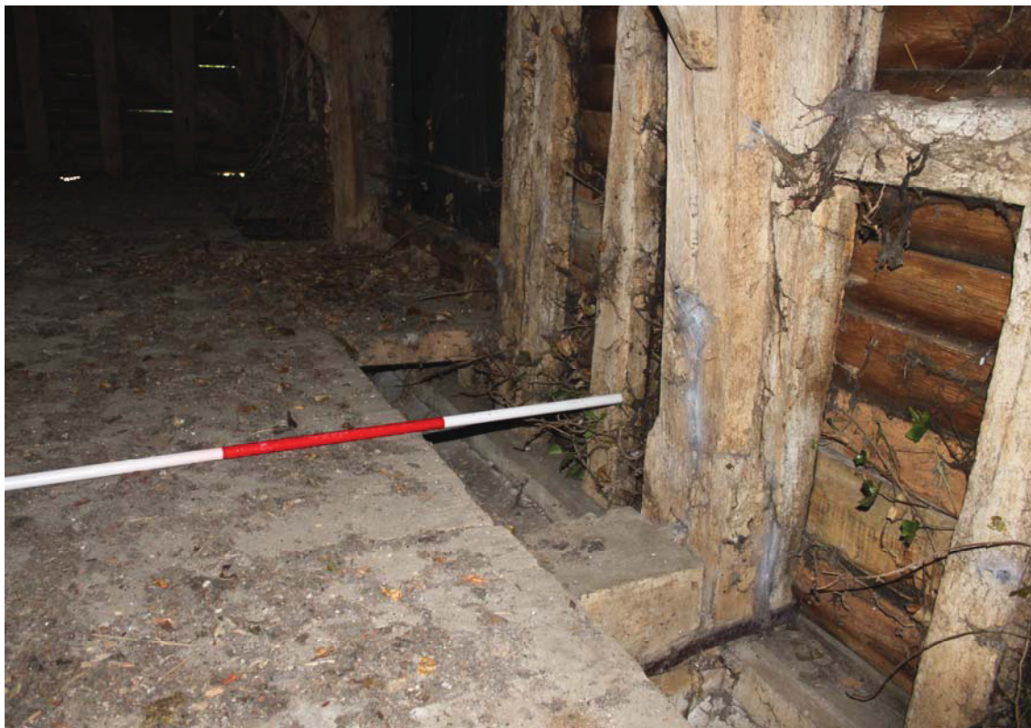
A2.12 Loading vent in floor above former hay rack (section 1a), showing the northern elevation of bay C to right with a 'bridge' to the 19 th century loading door in bay B in centre rear
