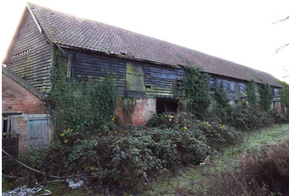
A2.4 Northern exterior of barn (1) from north-east showing the gable of the brick cow shed (5) to left. The two left-hand (eastern) bays of the barn were added in the mid-19 th century when the original roof was replaced and the lower storey rebuilt in brick.
