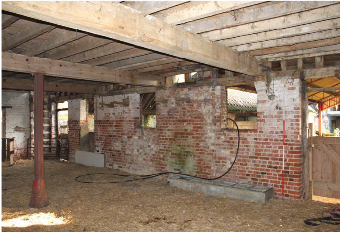
A2.7 Internal southern elevation of the 19 th century stable (1a) at the western end of the barn, showing the doors and windows to the southern yards. The principal ceiling joist in the foreground is original to the late-16 th century frame, but the rest are 19 th century insertions.
