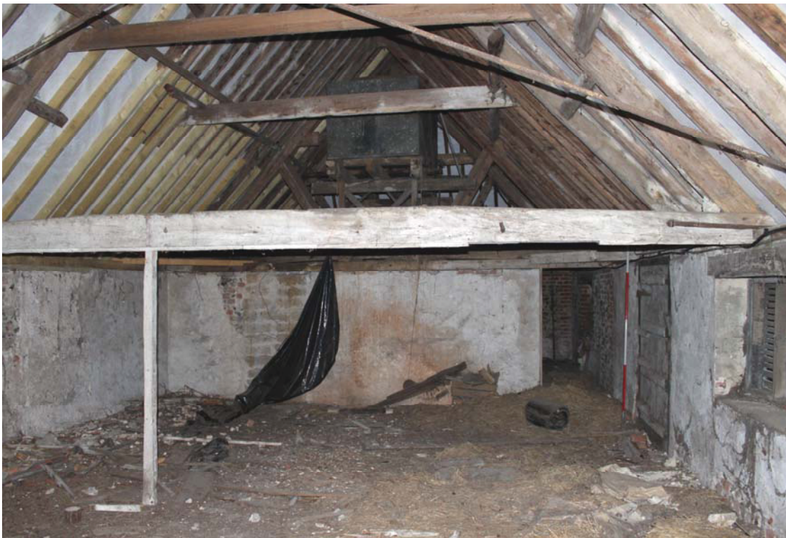
A2.8 Interior of stable loft (1) from west showing later door to coach house loft (2) and external loading door to right. The eastern gable shows a section of clay-lump repair to the left.
