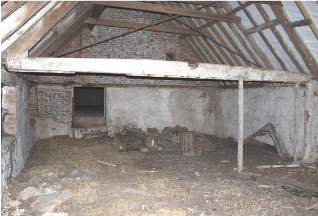
A2.7 Interior of stable loft (1) from east showing central tie-beam with remains of lateral partition and fragment of original roof structure of staggered butt-purlins to right. The secondary door in the western gable opened onto the loft above the clay-lump stable (4).
