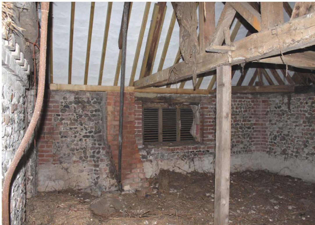
A2.10 Northern interior of coach house loft (2) showing original window and secondary chimney of copper with dentil cornice of original external gable to stable (1) to left.
