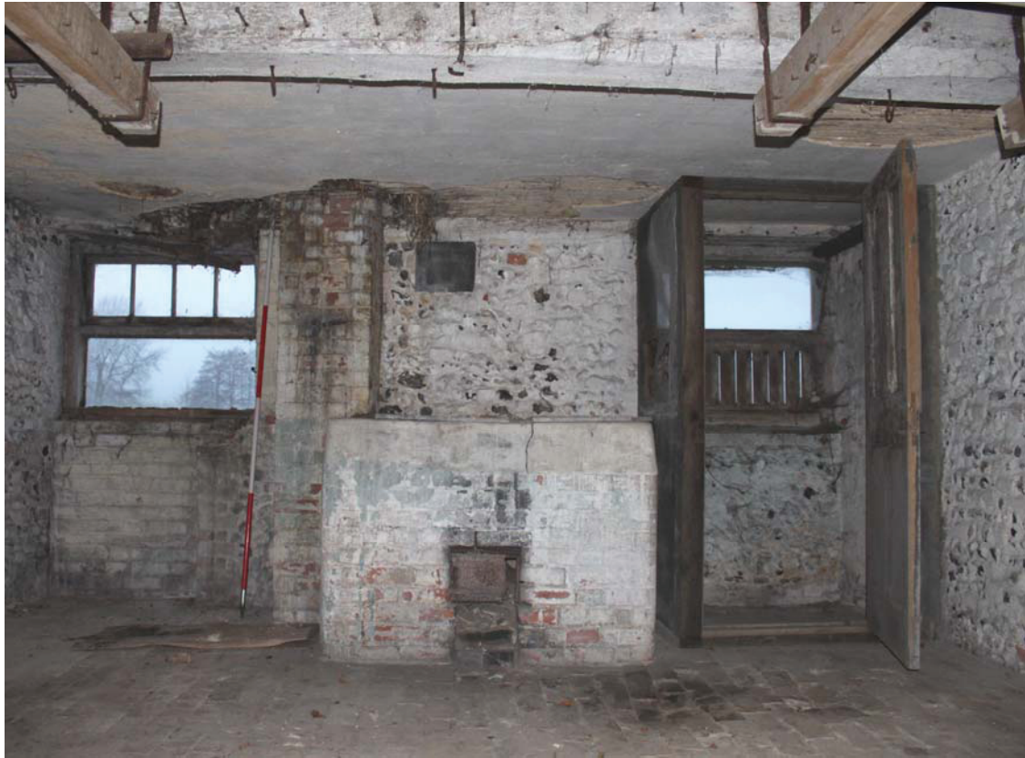
A2.9 Northern interior of coach house (2) showing later copper between blocked original doors (now converted into windows).
