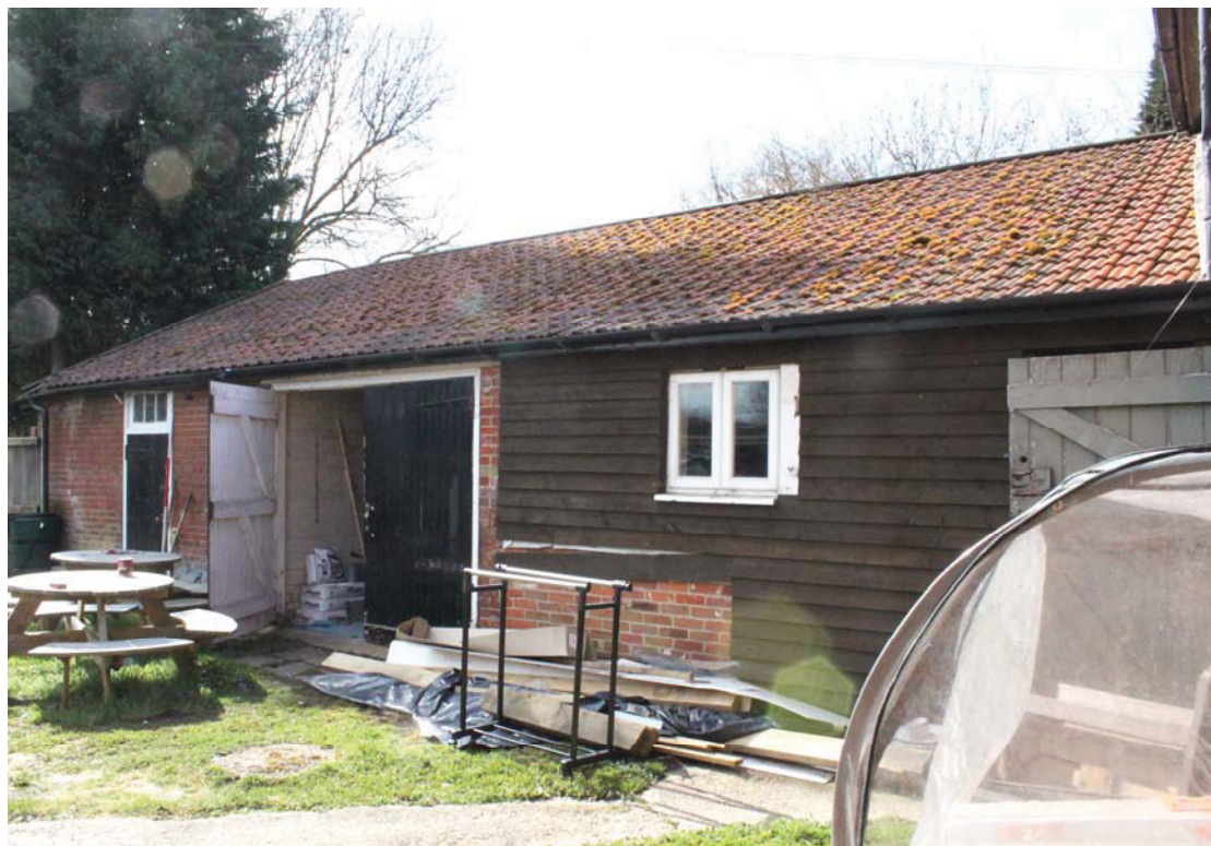
A2.6 Eastern exterior of pentice sheds seen from north-east, showing the vehicle shed (3) in centre, the enclosed southern shed to the left and the modern façade of the northern shed (2) to right.
