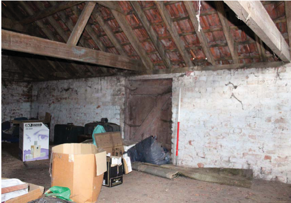
A2.7 Internal northern elevation of hay loft above stable (1) showing external loading door in centre and softwood clasped-purlin roof structure.
