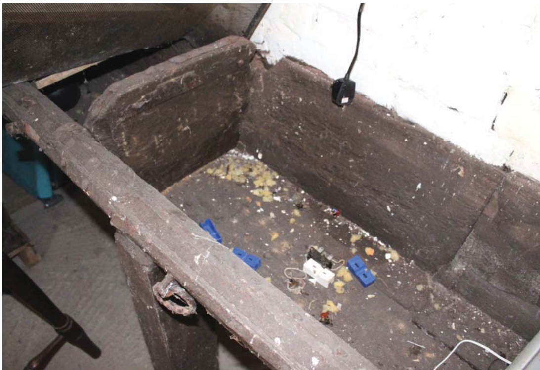
A2.10 Detail of boarded manger against northern interior of stable (1) showing internal division of trough to left.
