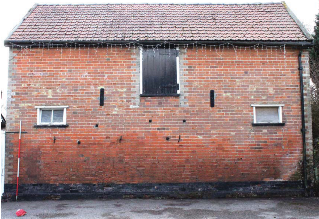
A2.3 Northern roadside facade of stable (1) showing original hay loft door with gault brick dressing in centre and evidence of blocked secondary ground-floor window or hatch to right.
