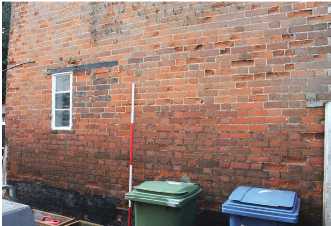
A2.4 Exterior of eastern gable showing partly blocked original window to left with numbered brick immediately beneath.
