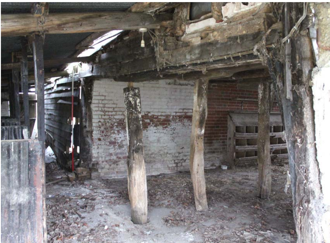
Illus. 8. 29. Northern external gable of granary seen from lean-to piggery to northwest. The gable is entirely open on the lower storey with a central Sampson post.
