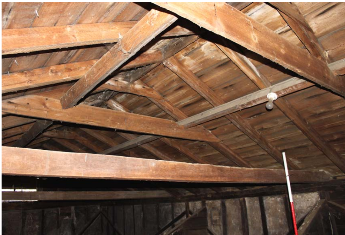
Illus. 10. Detail of softwood clasped-purlin roof structure seen from south-eastern corner of granary
