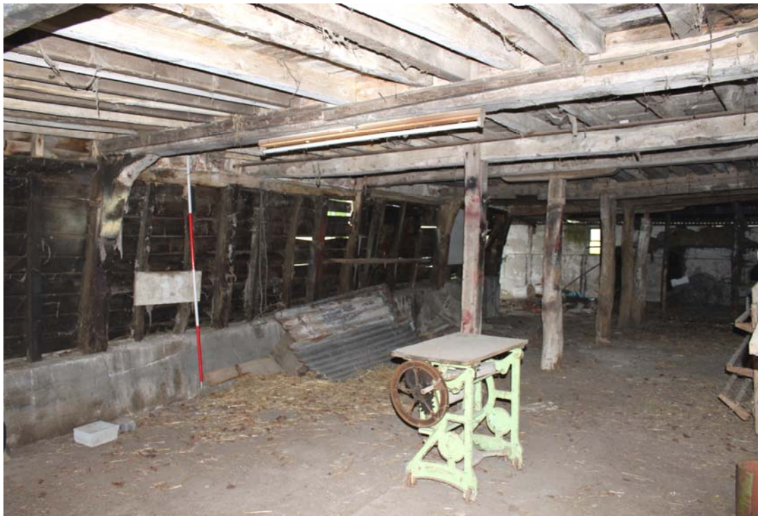
Illus. 6. Interior of lower storey from south-east, showing the Sampson posts in the centre of each binding joist (and the mid-rail of the northern gable) with the studwork western elevation to the left.
