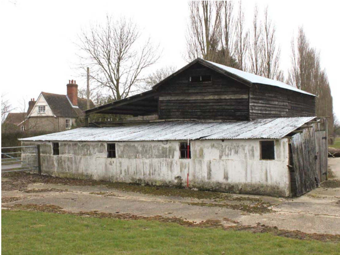
Illus. 5. Northern external gable of granary showing the adjoining 20th century lean-to piggy the proximity of Ringshall House on the opposite side of the road.
