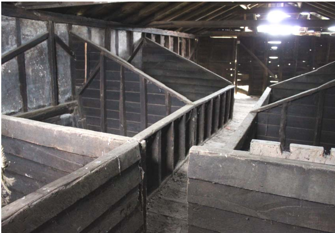
Illus. 12. The intact grain bins seen from north-western corner of the upper storey (the narrow gap in the foreground is a recent insertion).
