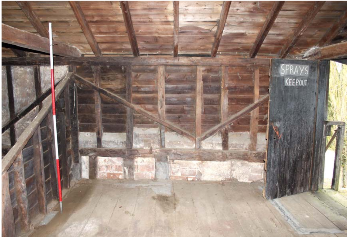
Illus. 11. Southern end of eastern internal elevation on grain floor, showing entrance in southern gable to right and the extent to which the original walls were raised in height (from the original roof-plate immediately above the floor to the present plate).
