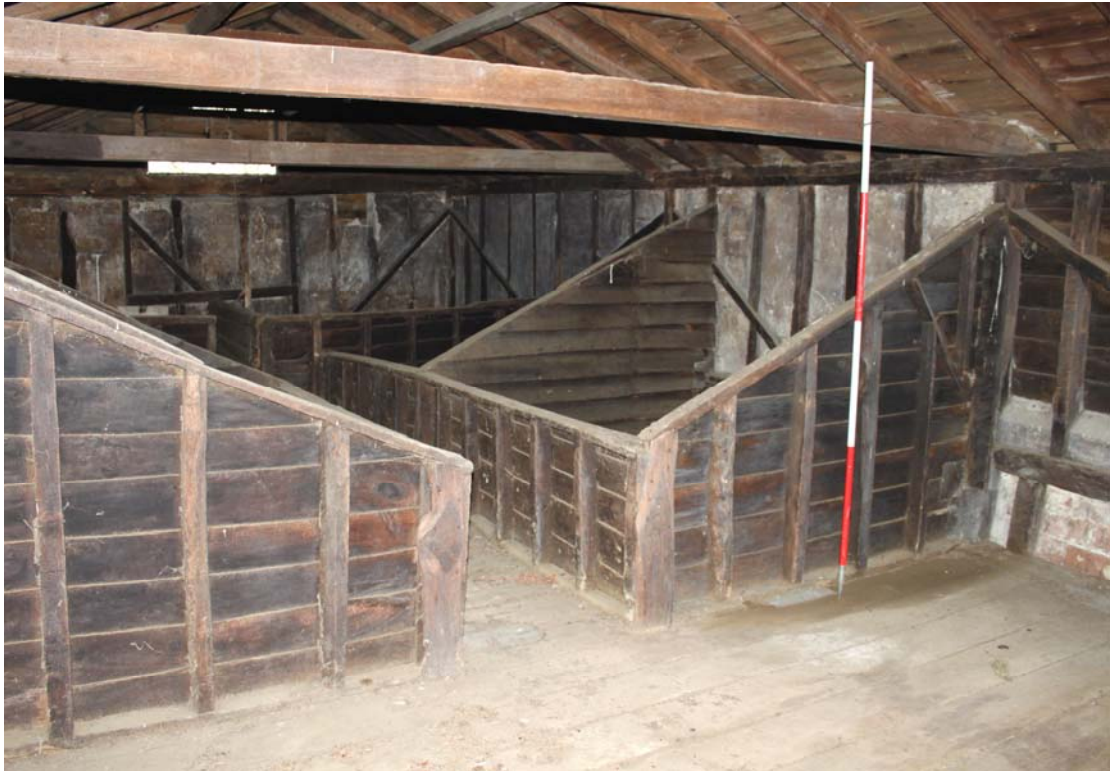
Illus. 9. Complete boarded grain bins seen from the south-western corner of the first-floor granary, showing the axial passage. The original roof plate and storey post are visible above the floor to the right. The walls were raised to accommodate the bins.
