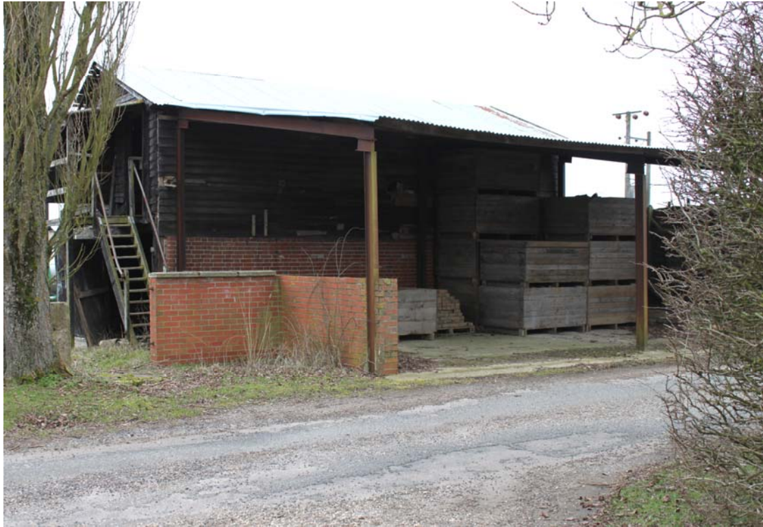
Illus. 3. Exterior of granary from east showing 20th century lean-to vehicle shelter adjoining road in foreground.
