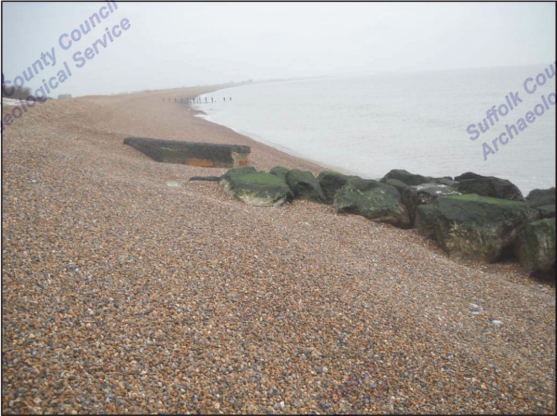
Plate 11. BAW 153 after completion of new sea defences, facing north (Courtesy of the Environment Agency)
