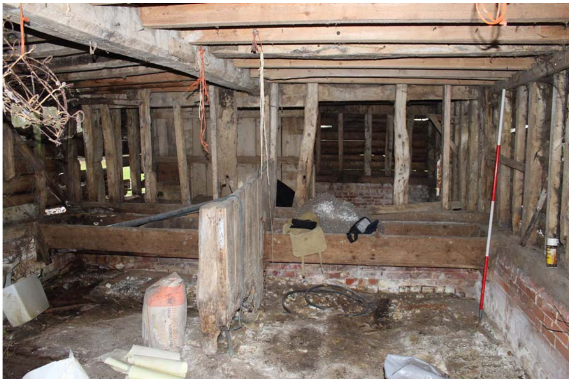
Illus. 6. Internal 'high-end' partition from east showing the low cattle manger and axial stall divider on the ground floor.
