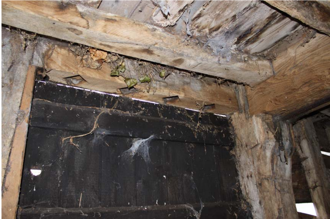
Illus. 9. Detail of the original diamond mullion mortises in the lintel of the northern door of the western stable. The step-stop chamfered binding joist with a neatly-cut corbel block is visible to the right.
