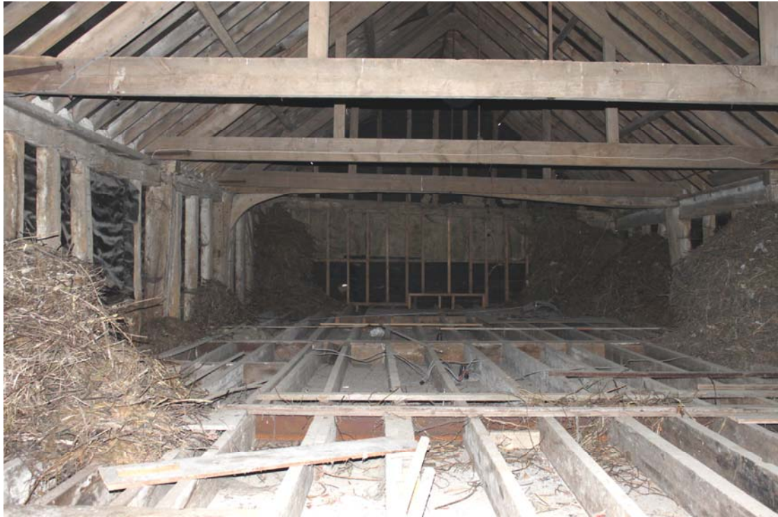
Illus. 7. General view from north of barn (1) above its ceiling of 20 th century tall-sectioned softwood joists, showing the early-20th century tie-beams and roof structure with original 16 th century framing to left & right and 20 th century rebuilt southern gable in rear.
