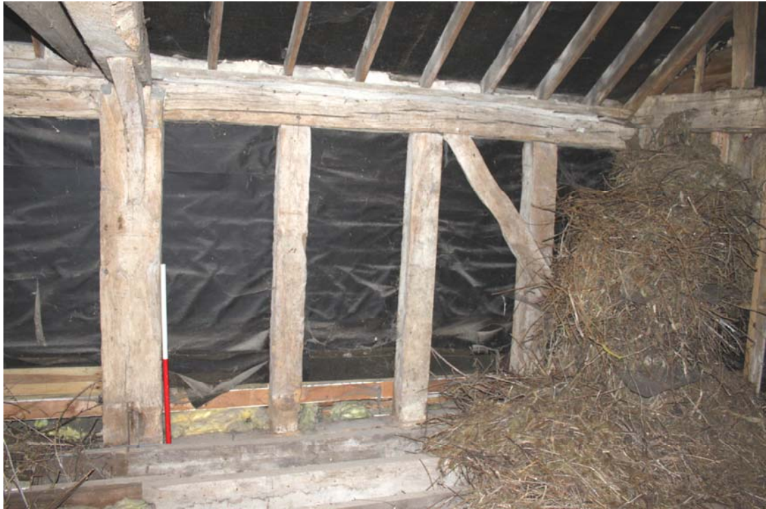
Illus. 11. Southern bay of eastern internal elevation of barn (1) showing the original internally trenched corner brace to right and the open truss of the two-bay stable to left. An identical brace survives at the southern end of the western elevation.
