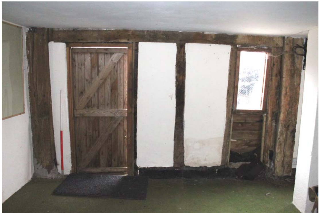
Illus. 6. Western interior of penultimate southern bay of barn (originally the northern bay of a two-bay integral stable) showing the inserted modern yard door to the left and the position of the original stable door to right (as indicated by a pegged and tenoned jamb abutting the storey post and a corresponding gap of 106 cm (3.5 ft) to its left). The southern bay beyond the modern left-hand partition forms a pair of WCs with no exposed framing.
