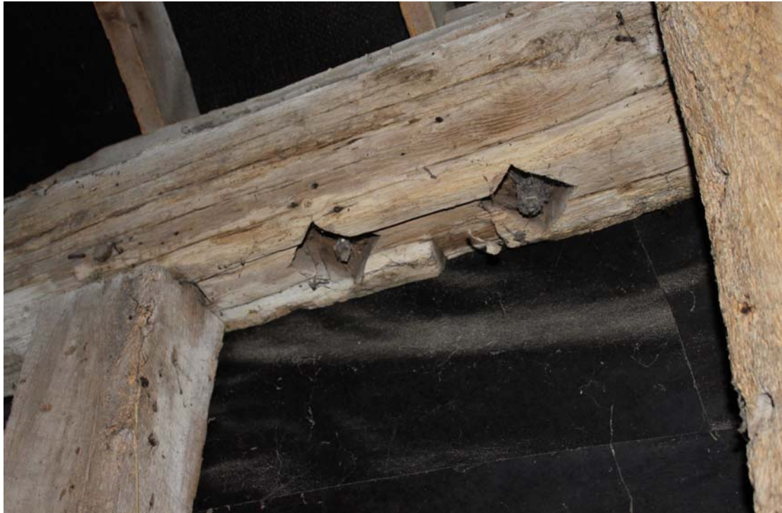
Illus. 9. Detail of eastern roof plate showing the diamond mullion mortises of the hay loft window in the penultimate southern bay (with storey post of central open truss to right). An identical three-light window adjoined the other (southern) side of the same truss in the western elevation, and the tie-beam of the southern gable contains six mullion mortises.
