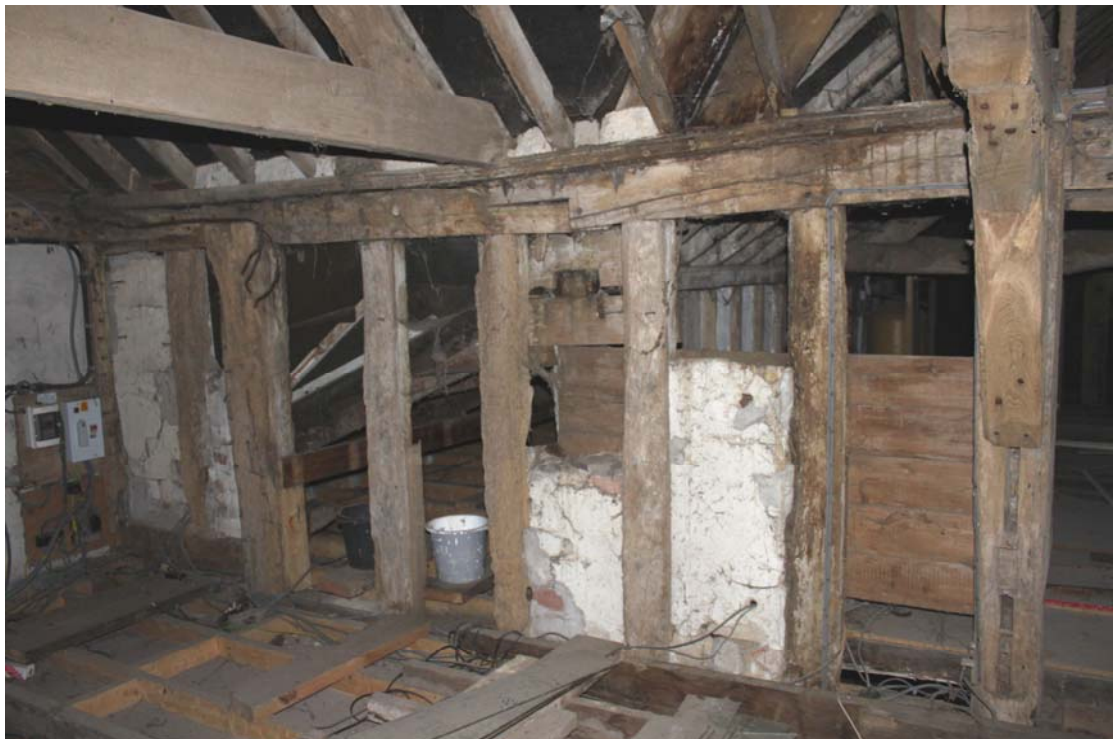
Illus. 8. Northern end of eastern internal elevation of barn (1) showing to left the narrow truncated bay with an original door lintel immediately above the modern ceiling and the original entrance bay to right. Note the edge-halved and bridled scarf joint in the roof plate and the empty mortises of the re-used storey post.
